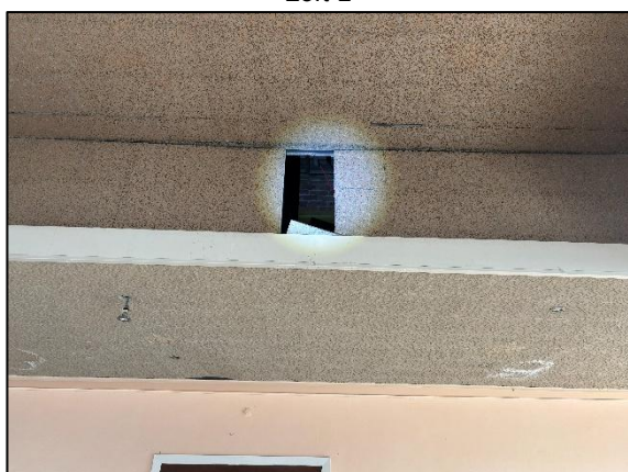
Holes in ceiling panelling leading to Loft 2
