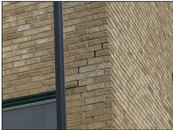
Missing mortar along the western elevation.
