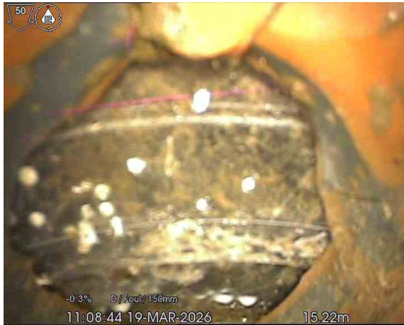
1, 00:01:51, 15.10 m Hole in drain or sewer from 11 o'clock to 1 o'clock
