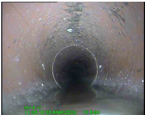
1, 00:02:04, 19.78 m Fracture, spiral from 7 o'clock to 10 o'clock
