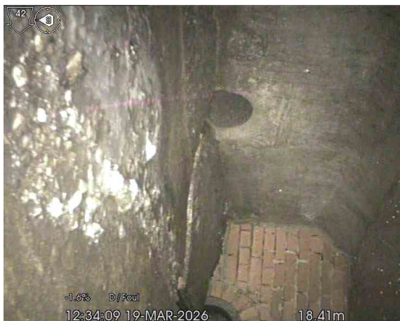
7, 00:04:52, 19.40 m Connection other than junction at 9 o'clock, 300mm dia, SURFACE WATER SEWER FROM MH3
