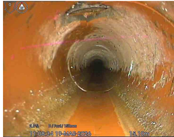
2, 00:01:51, 15.10 m Hole in drain or sewer from 11 o'clock to 1 o'clock
