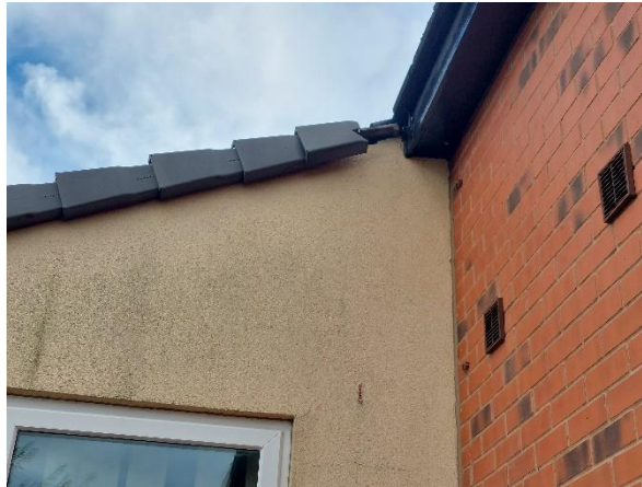
Plate 18 – View of missing dry verge tile on the eastern aspect of Surestart Children's Centre.
