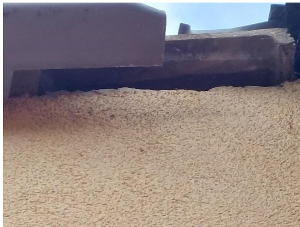
Plate 19 – View of gap to wall plate behind the missing dry verge tile on Surestart Children's Centre.
