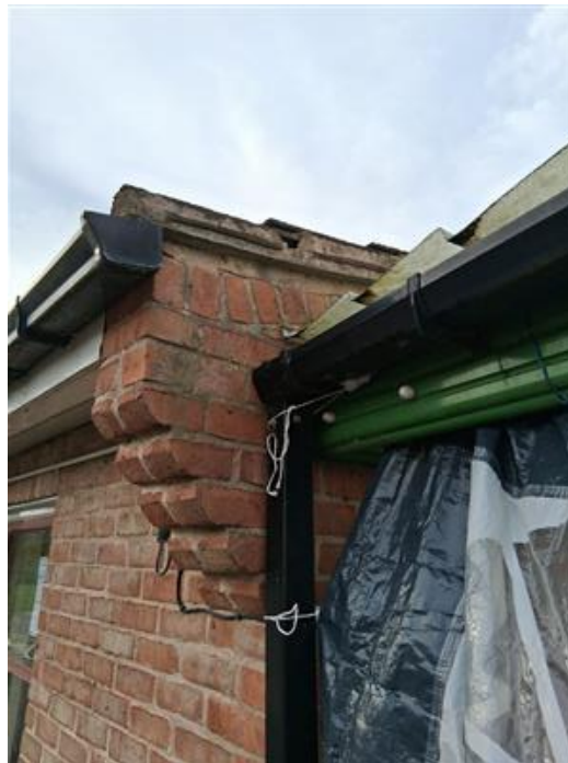
Plate 15 – View of gap in mortar on northern aspect of Building EFAA
