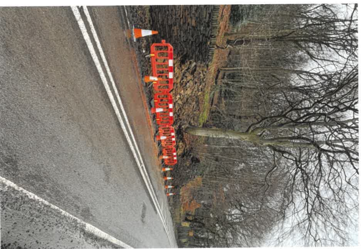
Photo 2 – Showing collapsed wall and relative proximity to dragons teeth markings and 30mph limit sign
