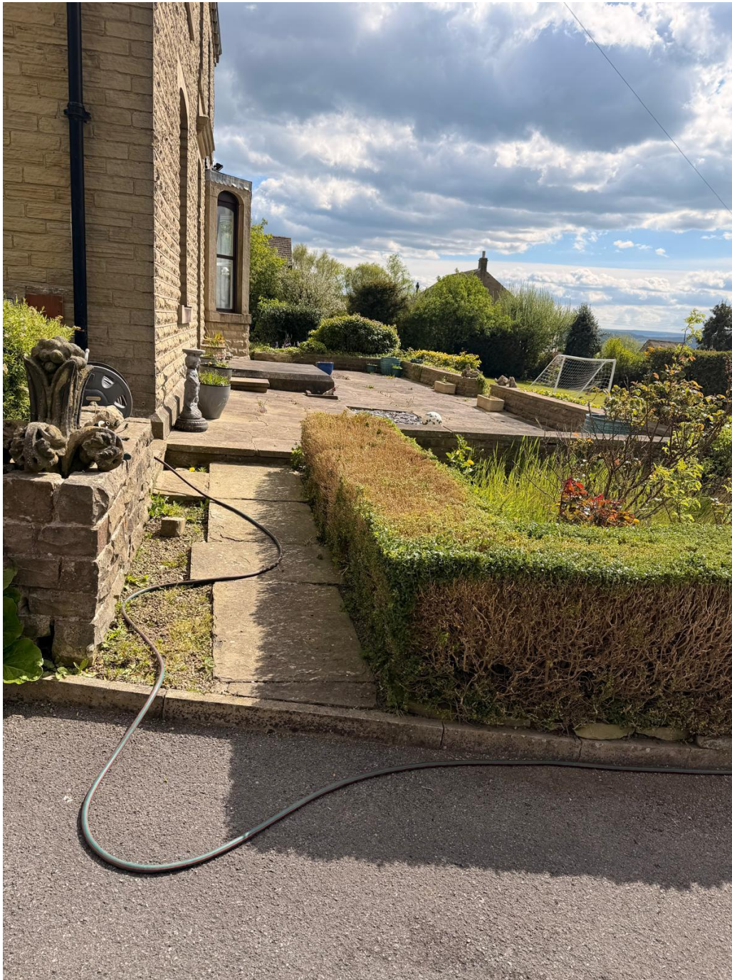
Plate 1: Internal Navigation Obstacles – View showing existing narrow, uneven paved paths and significant stone thresholds that prevent safe independent walker or wheelchair use.
