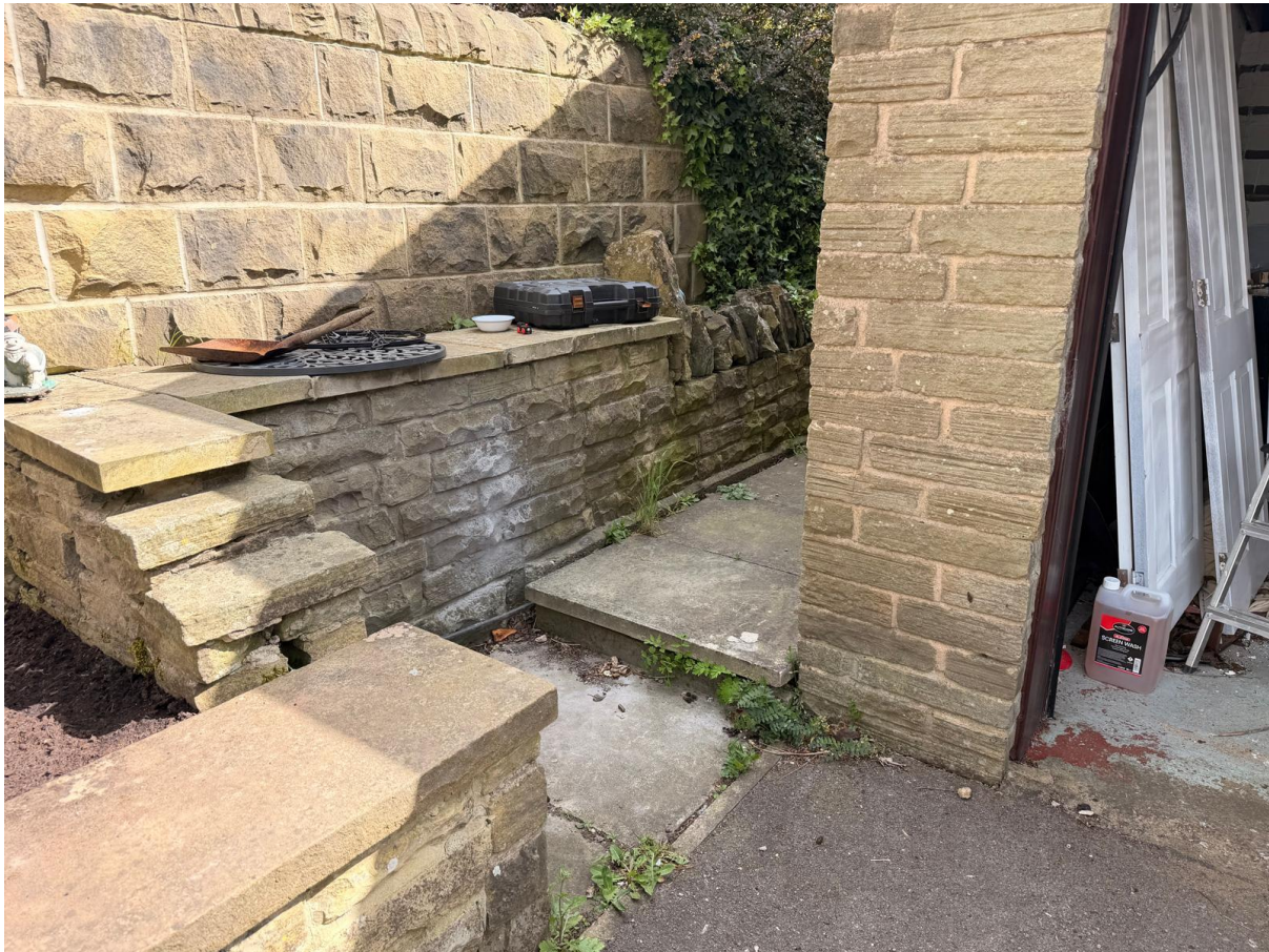
Plate 13: Technical Turning Barrier – View of stone walling and narrow steps that physically block the "continuous gait" required for effective mobility training.
