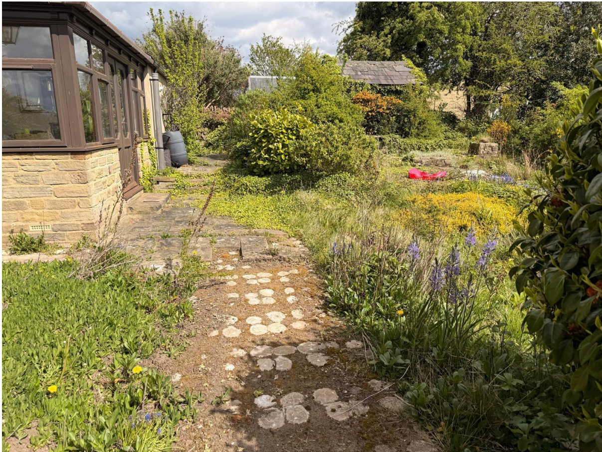
Plate 6: Unsafe External Surfaces – View of broken, overgrown paving and steep drops that necessitate a level, weather-protected internal therapy zone.
