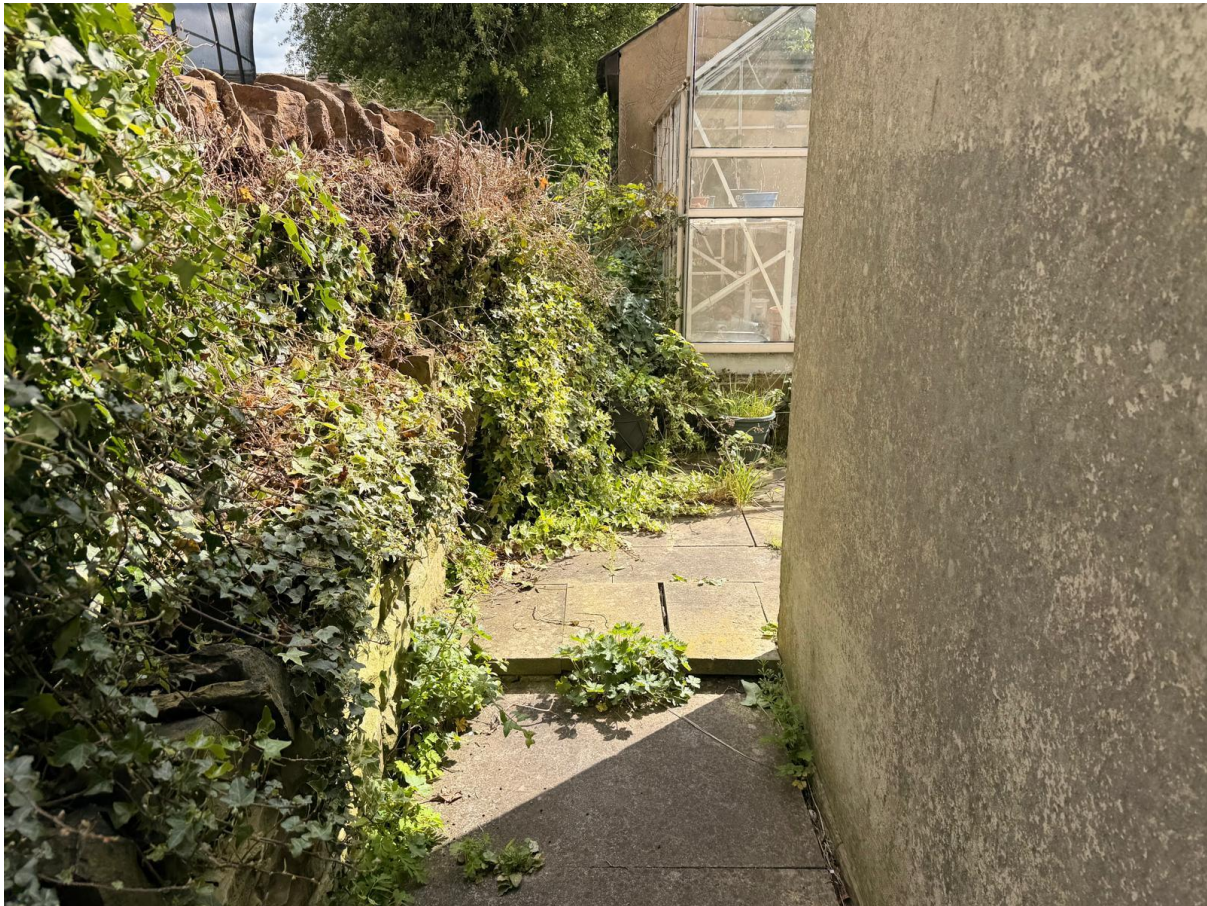
Plate 14: Confined Boundary Access – Final view showing the narrow, unsafe corridors between existing structures that justify the need for a spacious, open-plan Pavilion.
