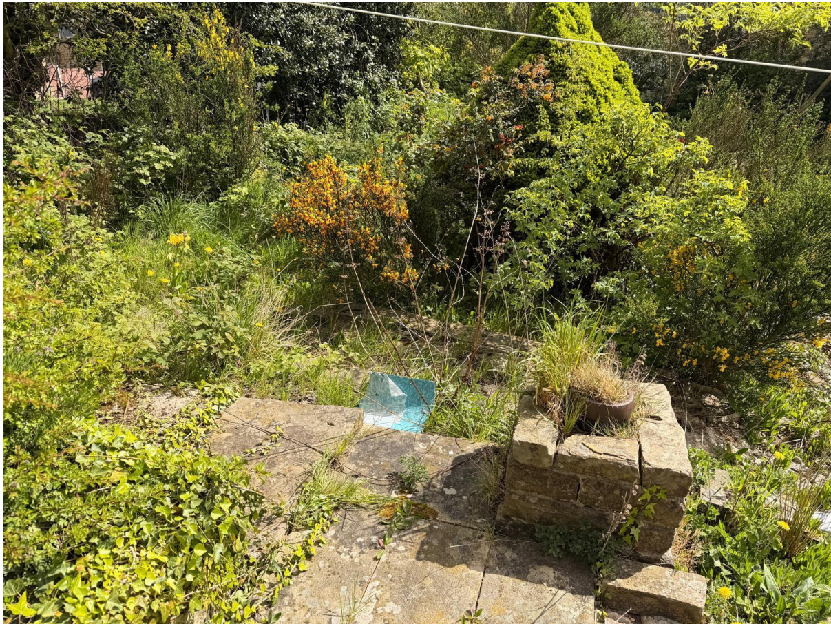
Plate 10: Infrastructure Barrier – View of essential drainage and utility placements located on uneven ground, further restricting the footprint of "safe" land.
