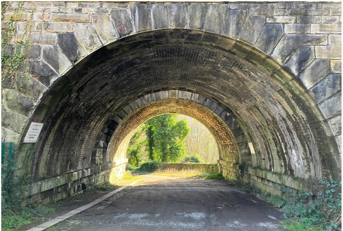
Figure 12: North elevation of Golcar New Viaduct MVL3/69, from farm track, with plain voussoirs and keystone, with the eastern arch of MVL3/70 beyond.
