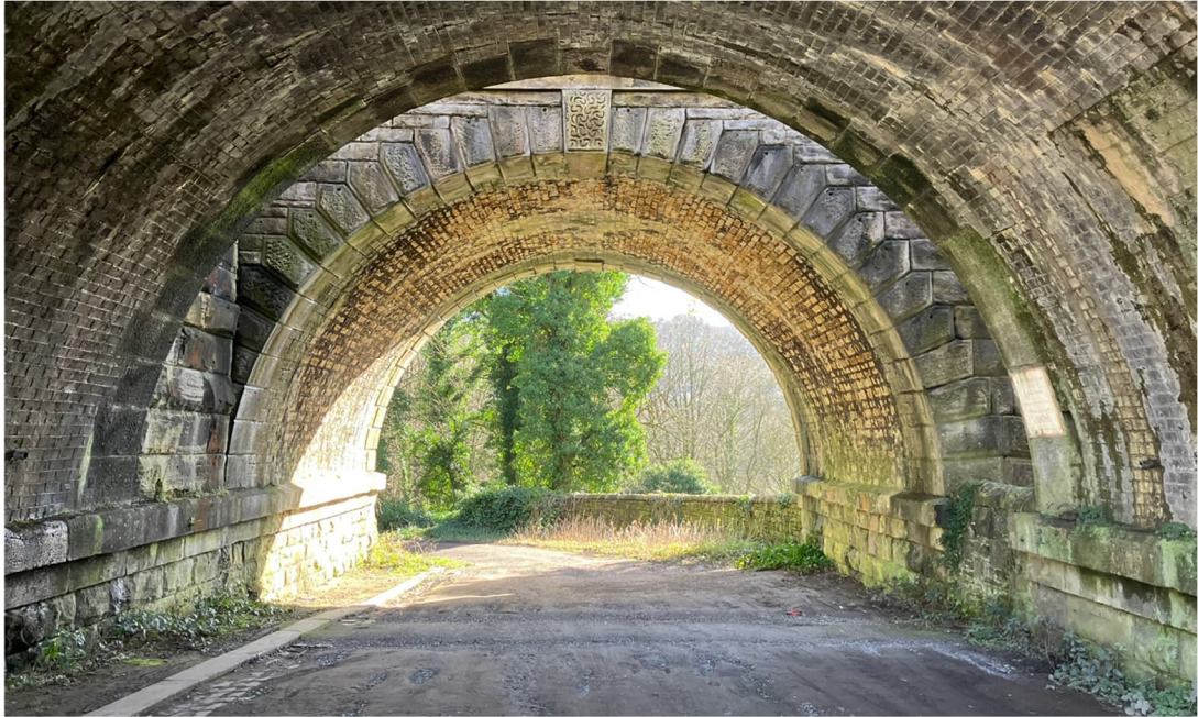
Figure 13: North elevation of the older Golcar Viaduct MVL3/70 featuring more decorative keystone and voussoirs.
