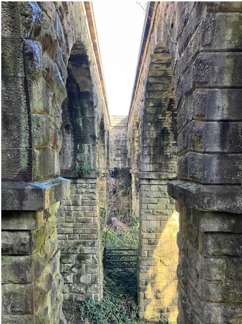
Figure 16: South elevation of Golcar new viaduct (MVL3/69) to left, original viaduct (MVL3/70) to right, looking north east from footpath.
