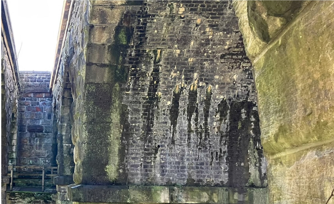
Figure 17: Water staining on arch of later viaduct MVL3/69, with a plastic water pipe centre bottom, looking south west from farm track.
