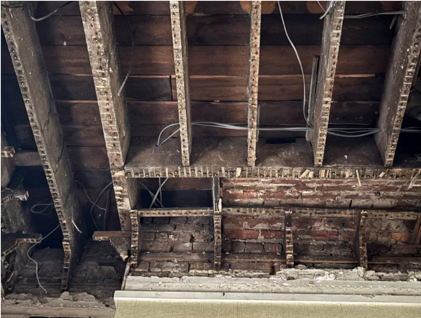
IMG_4403 - 2 nd floor (U/S) as viewed from 1 st floor (Room 095). Note: unsupported hearth vault & joists to hearth bearer not notched (gaff nailed only)
