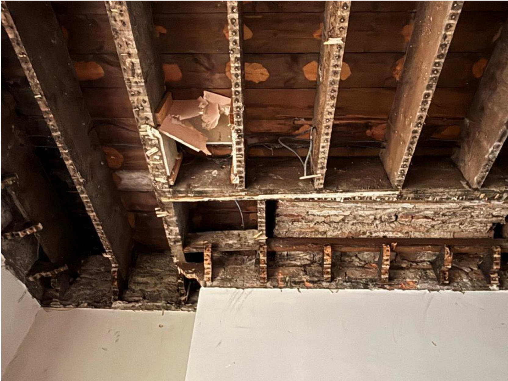
IMG_4398 - 3 rd floor (U/S) as viewed from 2nd floor (Room 140) Note: other end of timber joist with unsupported hearth vault support (lack).
