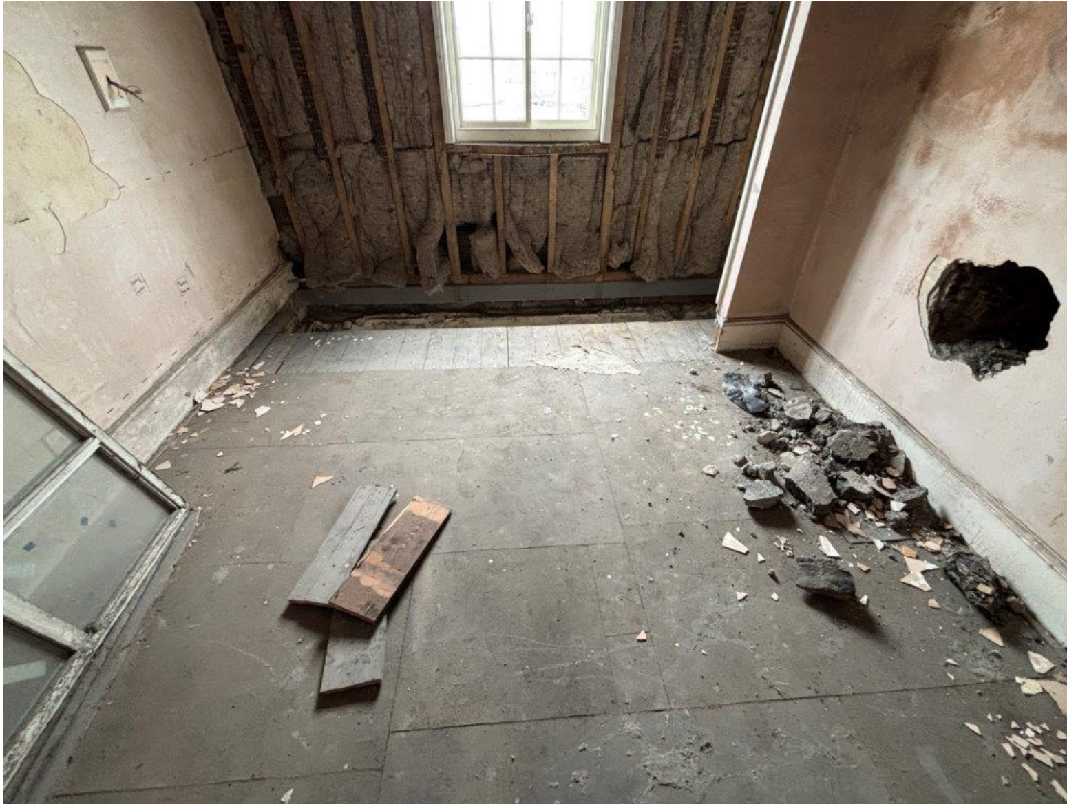
IMG_4390 – 4 th Floor (Room 193) Note: loss of 2nr joists and end floor timber floorboards (Historic)
