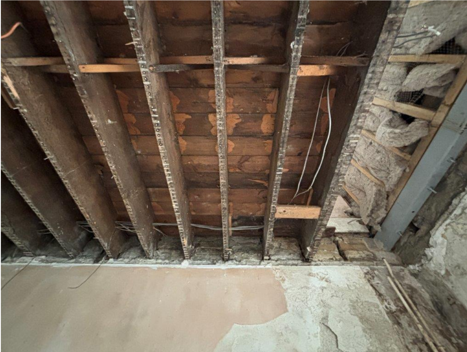
IMG_4394 - 4 th floor (U/S) as viewed from 3 rd floor (Room 181) Note: 5nr slim joists (from right of image) ends rotten – limited repair option due to joist slenderness.
