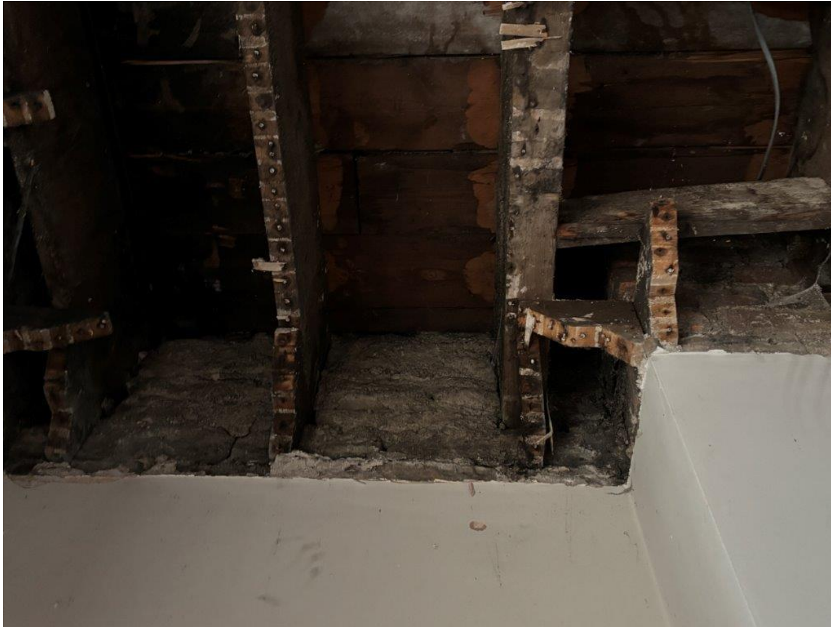
IMG_4399 - 3 rd floor (U/S) as viewed from 2nd floor (Room 140). Closeup – extremely slender pockets limiting replacement/ end repair approaches.
