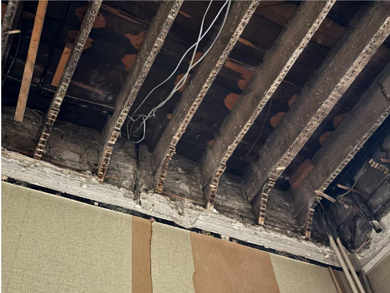
IMG_4402 – 2 nd floor (U/S) as viewed from 1 st floor (Room 095). Note: slender joists with some evidence of historic water impact
