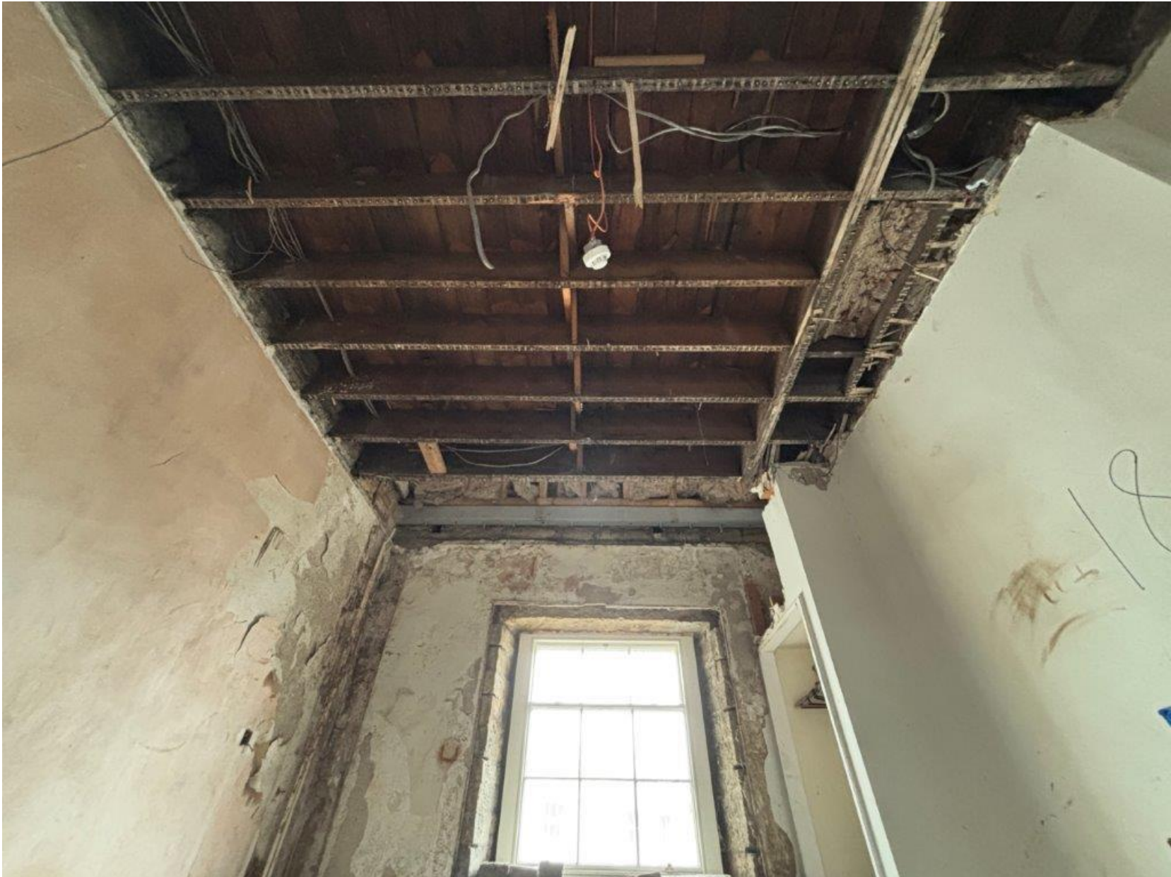
IMG_4392 – 4 th floor (U/S) as viewed from 3 rd floor (Room 181) Note: Unsupported hearth vault
