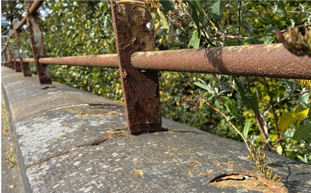
Figure 12: East parapet without bottom rail fixed directly into the coping stone joints.
