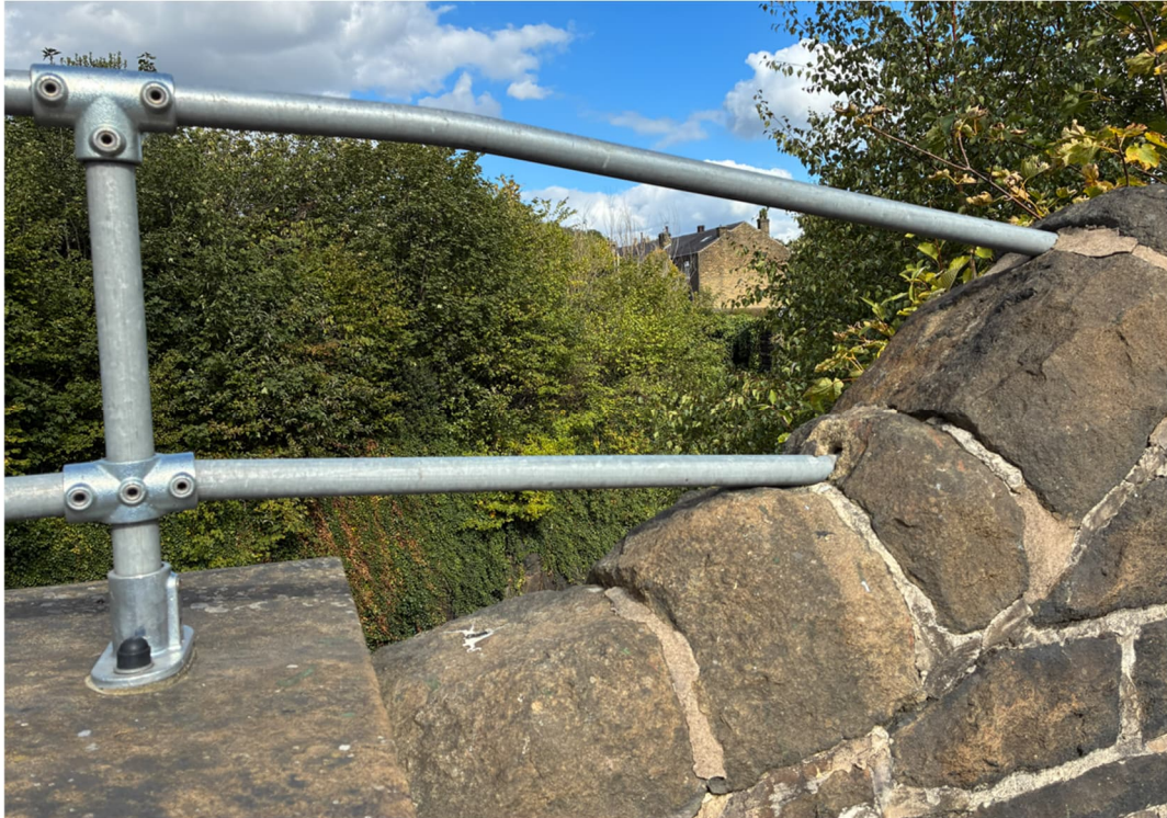
Figure 10: Detail of more recent replacement handrail at south end of east parapet.
