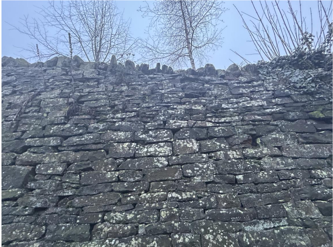
Photo B/F/5T – Wall B, Front Face, ~CH 10.2m (Upper Section)
