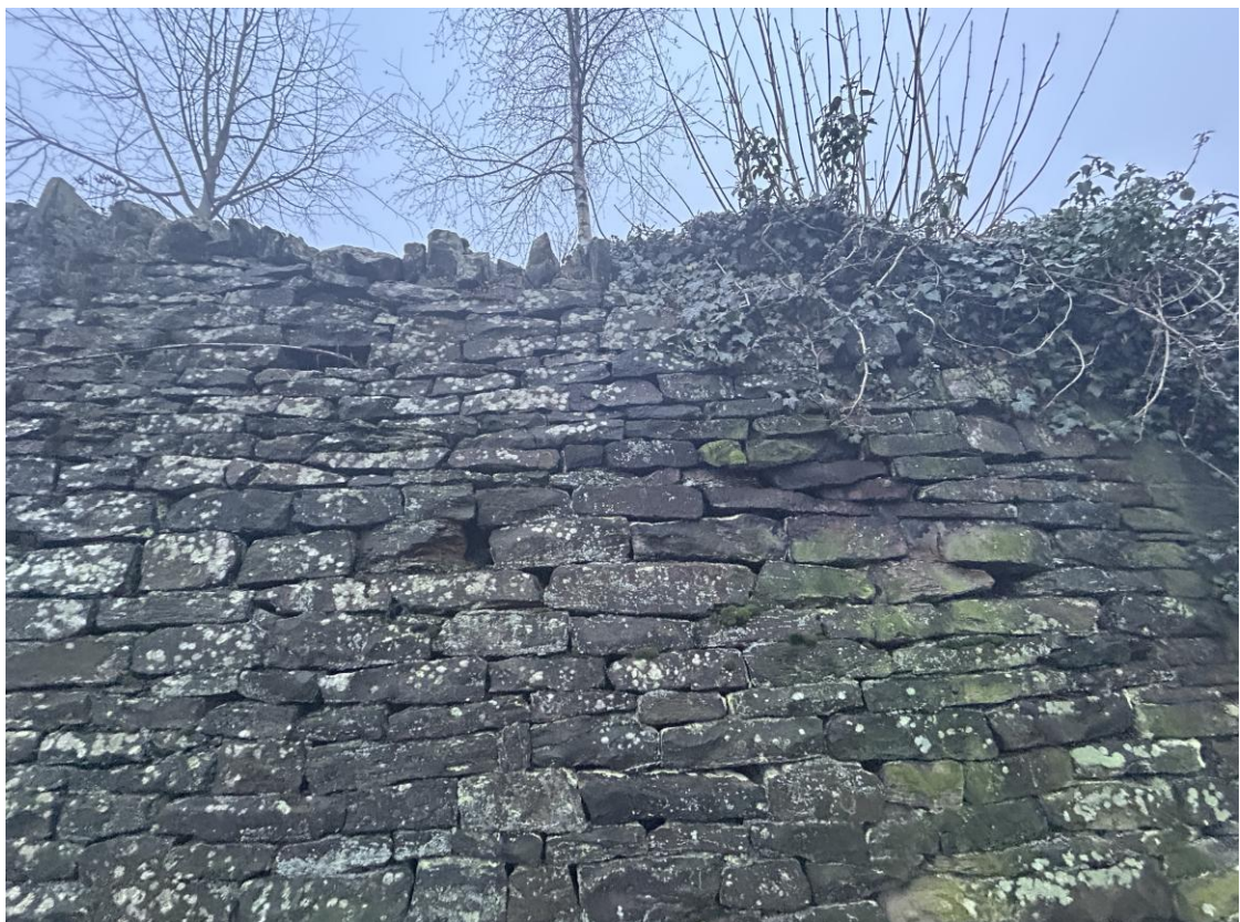
Photo B/F/4T – Wall B, Front Face, ~CH 8.5m (Upper Section)
