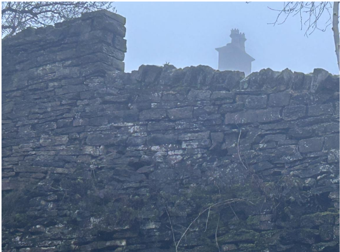
Photo B/F/12T – Wall B, Front Face, ~CH 23.5m (Upper Section)
