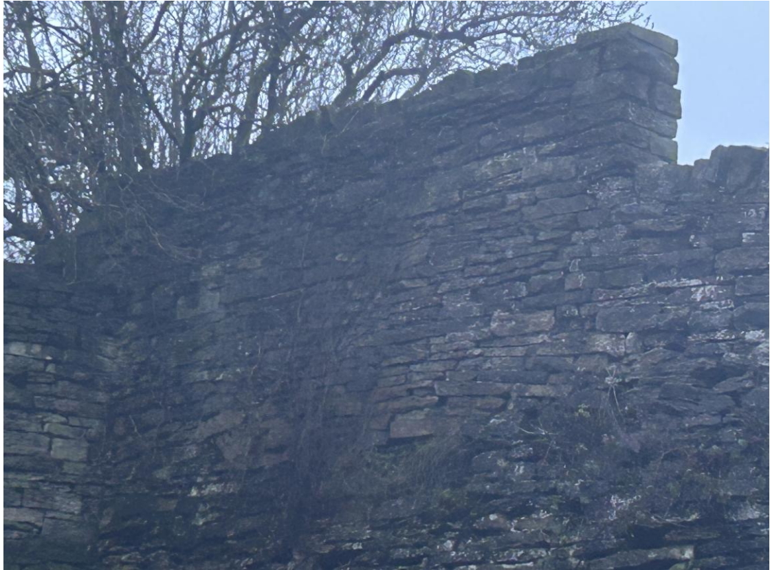
Photo B/F/13T – Wall B, Front Face, ~CH 25.5m (Upper Section)
