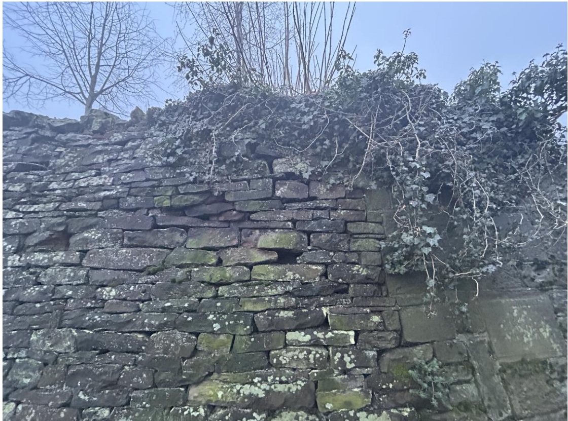
Photo B/F/3T – Wall B, Front Face, ~CH 7.5m (Upper Section)
