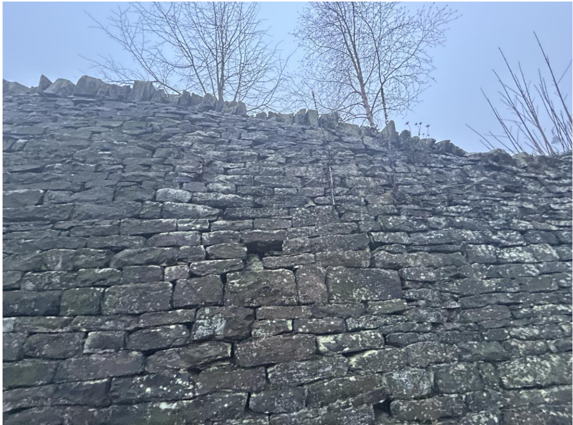
Photo B/F/7T – Wall B, Front Face, ~CH 12.5m (Upper Section)
