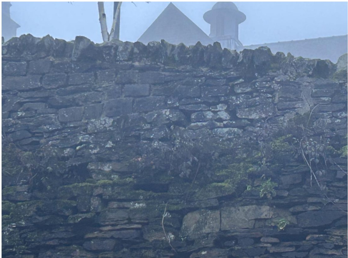
Photo B/F/11T – Wall B, Front Face, ~CH 21.5m (Upper Section)
