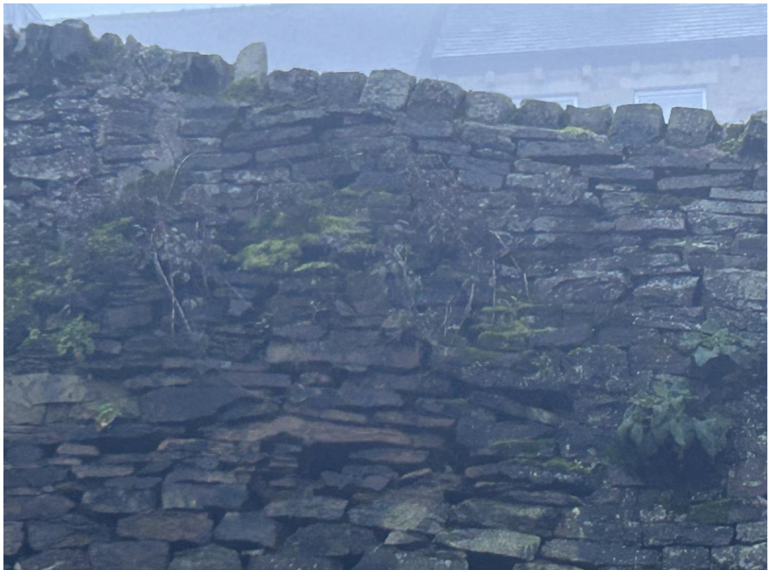
Photo B/F/10T – Wall B, Front Face, ~CH 19.0m (Upper Section)
