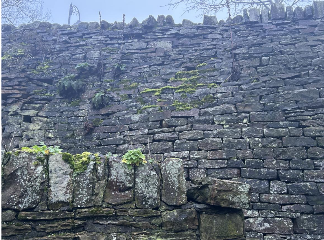
Photo B/F/9T – Wall B, Front Face, ~CH 16.0m (Upper Section)
