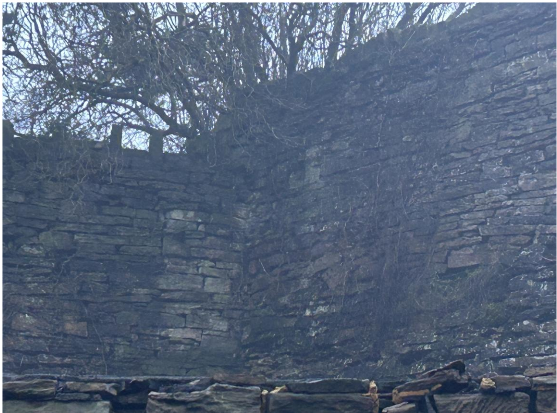
Photo B/F/14T – Wall B, Front Face, ~CH 27.0m (Upper Section)
