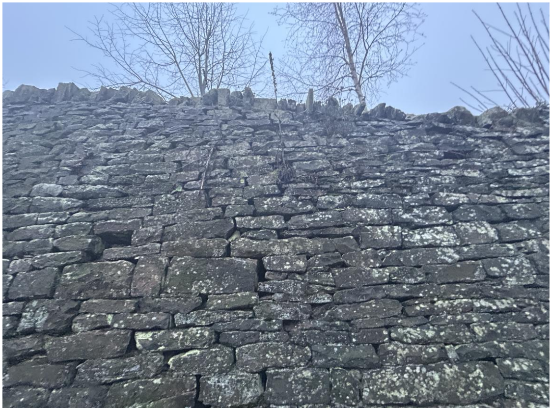
Photo B/F/6T – Wall B, Front Face, ~CH 11.5m (Upper Section)
