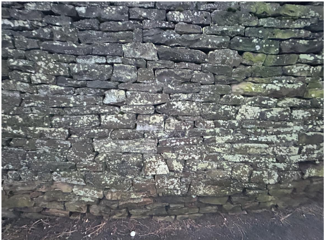
Photo B/F/4L – Wall B, Front Face, ~CH 8.5m (Lower Section)
