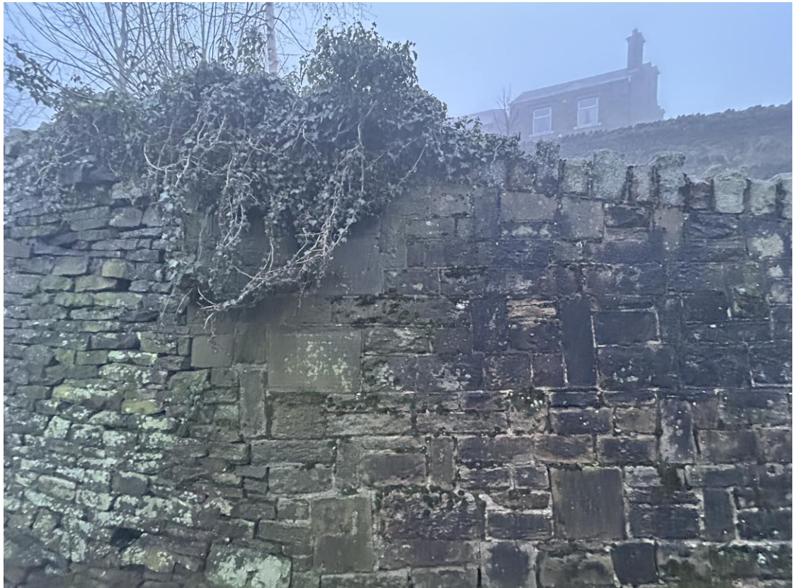
Photo B/F/1T – Wall B, Front Face, ~CH 5.5m (Upper Section)
