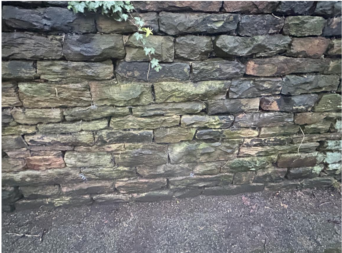
Photo G/F/4B – Wall A, Front Face, ~CH 2.0m (Lower Section)
