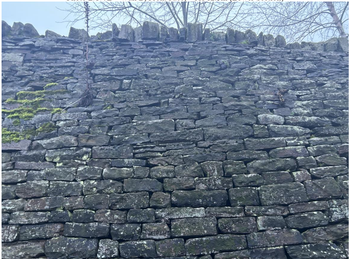
Photo B/F/8T – Wall B, Front Face, ~CH 13.2m (Upper Section)
