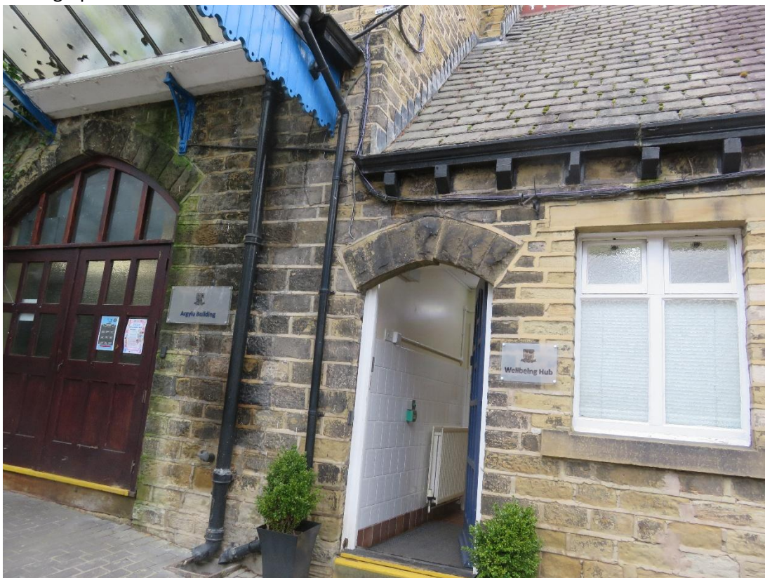
Arch opening same style as the front two storey section so built at the same period, right hand side window to the single storey section may have been inserted later.
