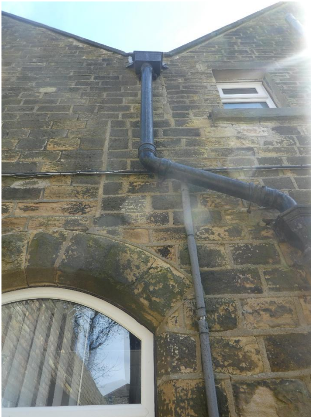
Vertical joint showing two separate buildings.
