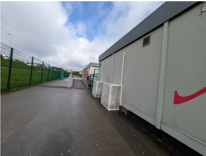
Photo 7 - Fixed AC units and security fencing
