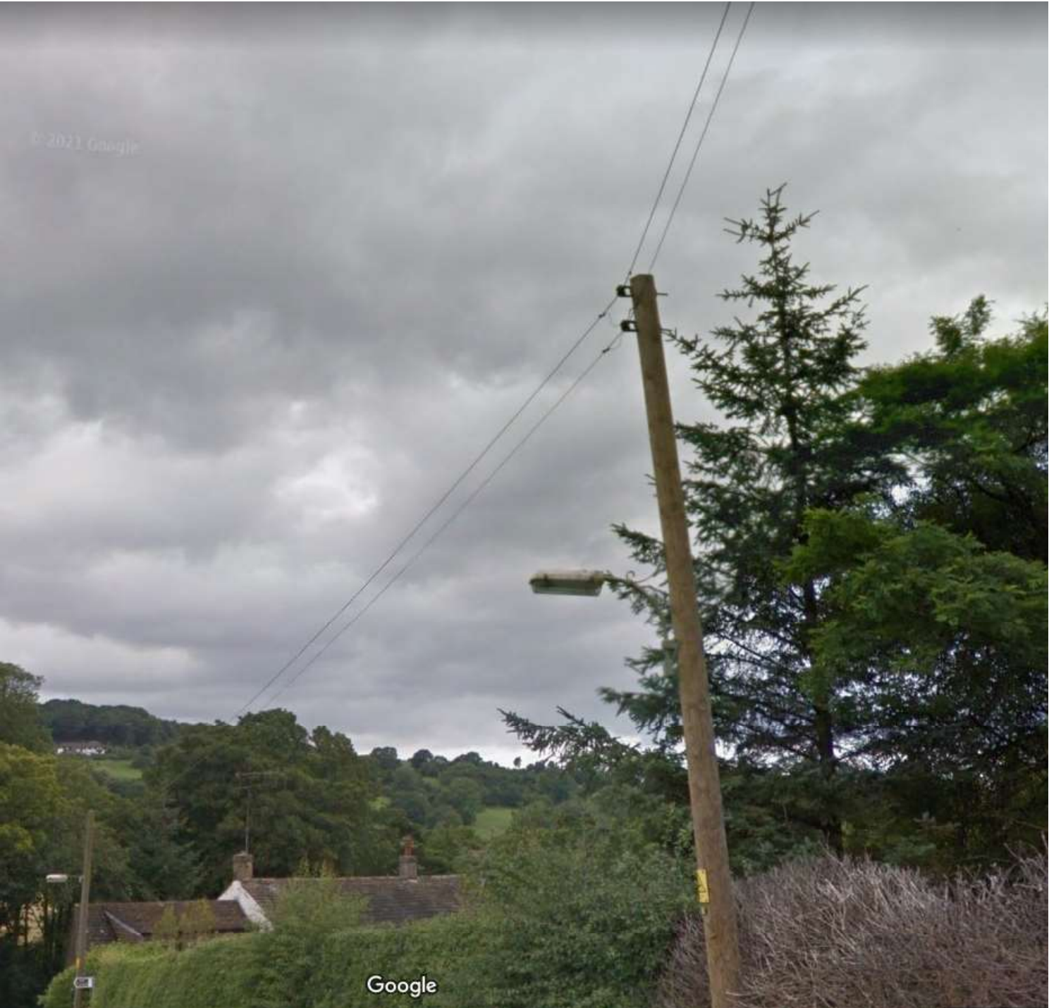
Example of open wire LV conductor before being upgraded to aerial bunched conductor
