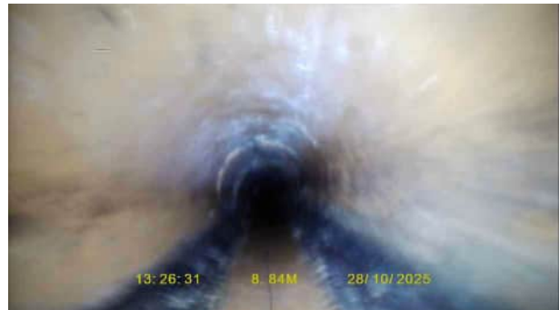
FW10X_077355ee-fb3b-4b52-b57b-9b671e513dc4_20251112_094606_908.jpg, 00:00:34, 8.90 m Crack, longitudinal at 7 o'clock
