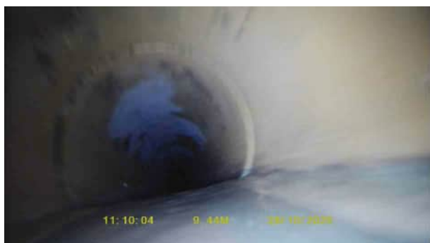
FW1X_e22c0d4d-da6a-44d6-b8d2-c4ba35c96a92_20251119_122751_755.jpg, 00:00:29, 9.40 m Joint displaced, medium
