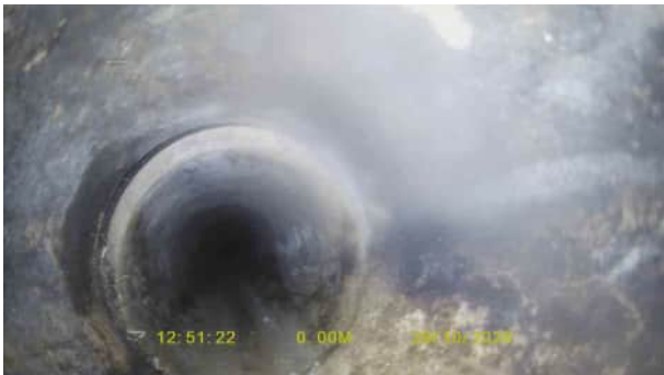
FW15X_c47f3519-2aef-4f58-b566-75b58edba86_20251120_142717_261.jpg, 00:00:02, 0.30 m Joint displaced, medium
