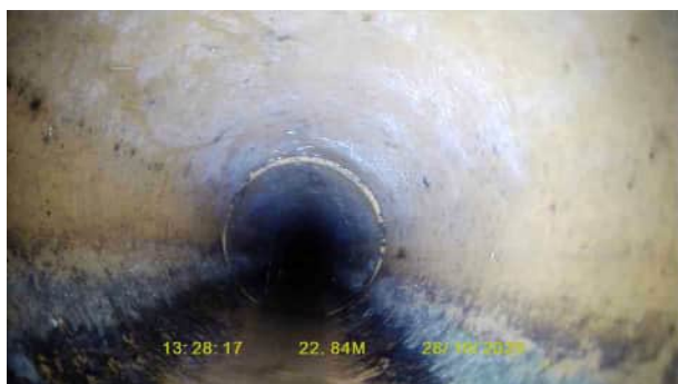
FW10X_8cb0f7d3-f8f3-4a77-9922-20841c327a18_20251112_103149_500.jpg, 00:02:20, 23.30 m Joint displaced, medium
