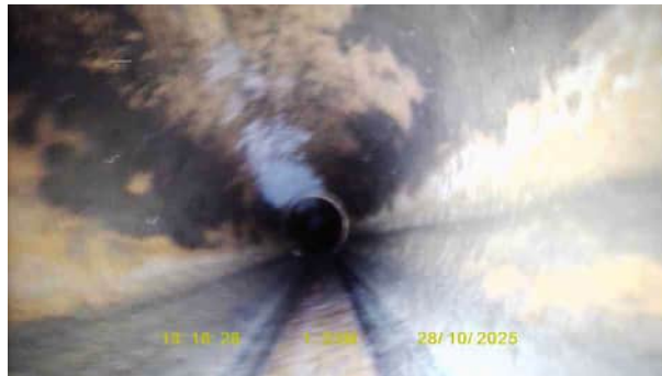
F5X_20481a2c-edda-4770-8428-e4544c3a0b90_20251111_151230_068.jpg, 00:00:07, 2.20 m Joint displaced, medium
