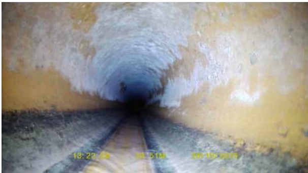
F5X_bf9c670c-df98-4406-b0ae-73b764d32fc0_20251112_090 243_777.jpg, 00:04:07, 39.42 m Survey abandoned, Traction
