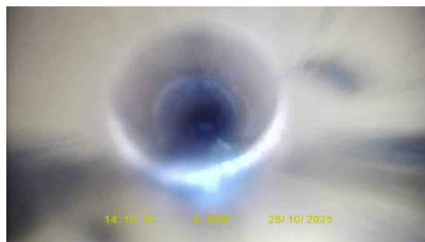
SW7X_607232eb-aa84-48b9-8e56-52da56959268_20251112_150450_649.jpg, 00:00:30, 7.00 m Joint displaced, large
