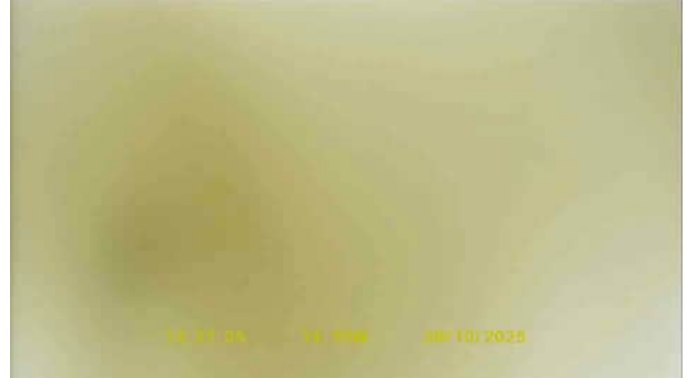
FW10X_42638c79-95bf-4fe6-b475-ce8a4adaa6bf_20251112_101011_839.jpg, 00:01:08, 15.00 m Joint displaced, medium
