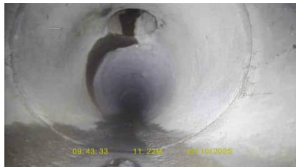
SW6AX_1cc8c72f-c0d6-49d5-a373-936b8f36c9aa_20251120_104523_188.jpg, 00:03:10, 12.30 m Junction at 12 o'clock, 150mm dia
