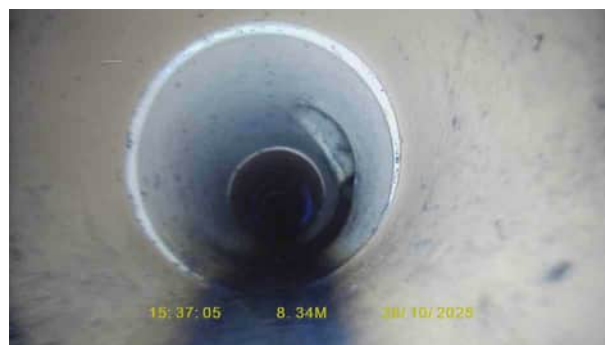
SW12X_5227fff9-69f8-4cdc-843a-ac71f5b850f6_20251120_093106_165.jpg, 00:00:38, 8.90 m Joint displaced, medium
