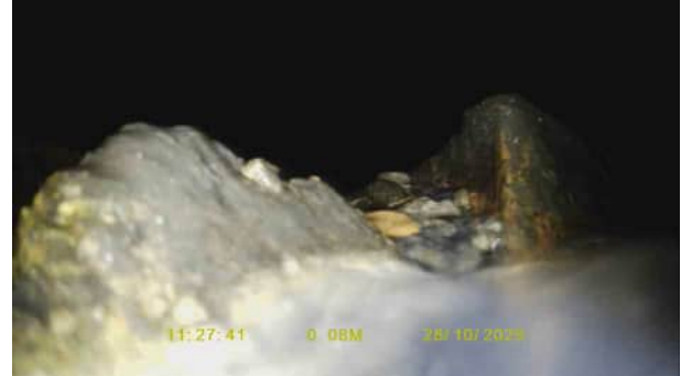
S1X_f9988cf4-086b-4b6f-a43a-42ab54f98484_20251105_145615_735.jpg, 00:00:03, 0.25 m Other obstacles, brick or masonry in invert from 5 o'clock to 7 o'clock, 30% cross-sectional area loss
