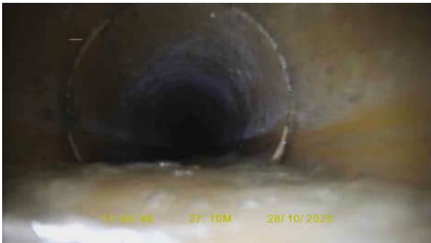
F1X_2a07ccbe-25cb-454d-a96b-777802066aa4_20251105_141332_621.jpg, 00:01:58, 27.20 m Joint displaced, medium
