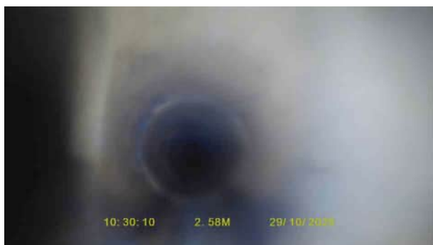
F23X_a796e45f-509e-4451-947a-2d8b60229c1f_20251120_115643_711.jpg, 00:00:11, 3.00 m Junction at 9 o'clock, 100mm dia
