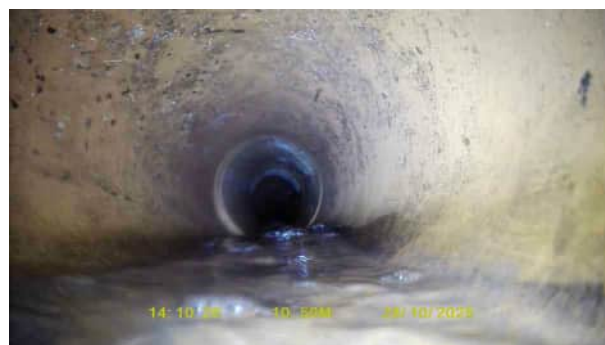
SW7X_2c5e743a-e503-4b7b-9c62-5ce043e88d00_20251112_153020_408.jpg, 00:00:47, 10.90 m Joint displaced, large
