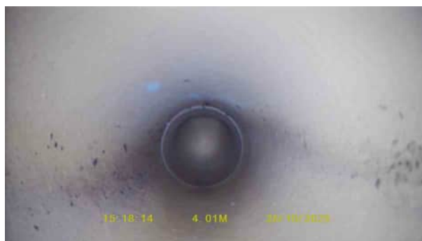
F17X_30355b48-7cba-4b5c-ae37-c60b2e39dc3f_20251120_085819_011.jpg, 00:01:09, 4.50 m Finish node, other special chamber, reference: F17, WP
