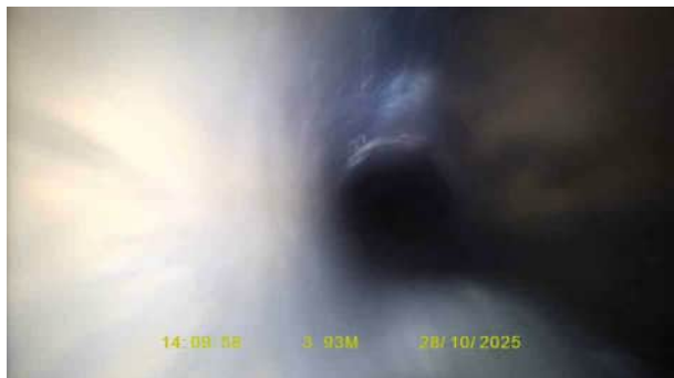
SW7X_ddec846a-44d6-42c7-b6b0-1c121ad126d2_20251112_145057_336.jpg, 00:00:18, 4.40 m Joint displaced, medium
