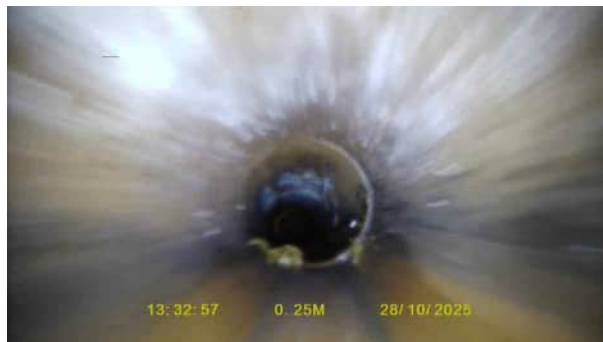
FW5X_26907e93-da37-43a8-b343-da660b5443da_20251112_104058_307.jpg, 00:00:02, 0.50 m Joint displaced, medium
