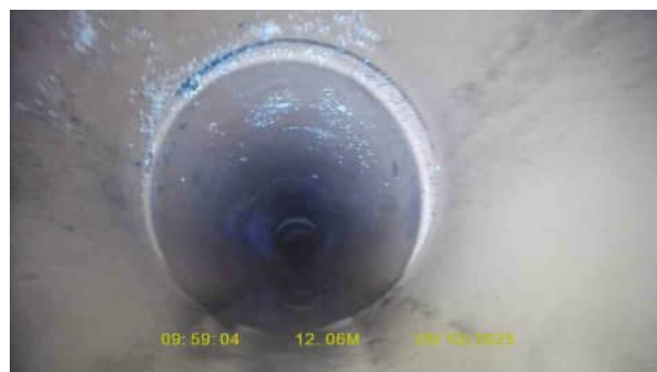
SW8X_6b7aa3e6-624d-43c7-a01f-2c84c24d9417_20251120_111340_944.jpg, 00:00:54, 12.40 m Joint displaced, medium
