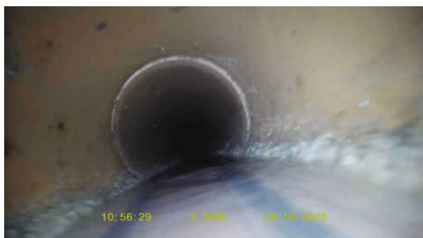
FW3X_e738eed4-f1b5-4782-b250-e9f5282f7fa0_20251105_132143_702.jpg, 00:00:16, 4.00 m Joint displaced, medium
