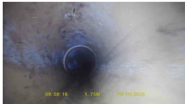
SW8X_7c4436a6-c99b-4f92-9f0b-8304691609a5_20251120_110306_556.jpg, 00:00:06, 2.40 m Joint displaced, medium
