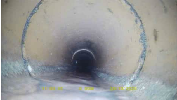
FW1X_2afb8f16-cea3-45c5-88e9-e817ba18081a_20251105_142446_326.jpg, 00:00:00, 0.00 m Start node, inspection chamber, reference: FW1
