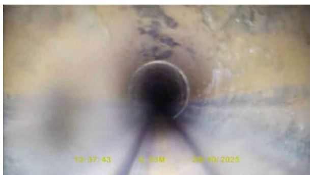
FW3X_d94fc0fa-2b98-4d40-8bcb-c1e5c83bc869_20251112_113714_025.jpg, 00:00:04, 0.80 m Joint displaced, medium
