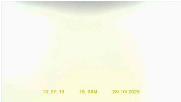
FW10X_0c9968a9-4ddf-46d7-9399-b31673ade2fc_20251112_101230_846.jpg, 00:01:16, 16.60 m Joint displaced, medium
