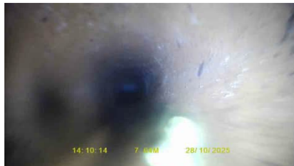
SW7X_caea7f4e-565c-40fa-838f-788255641e35_20251112_150945_664.jpg, 00:00:35, 8.20 m Cracks, spiral from 12 o'clock to 12 o'clock
