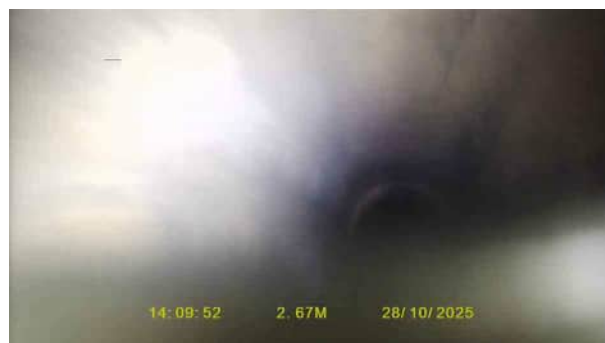
SW7X_4fc16604-51e6-4740-b5f3-8dba510fab5d_20251112_1 44910_050.jpg, 00:00:13, 3.10 m Joint displaced, medium
