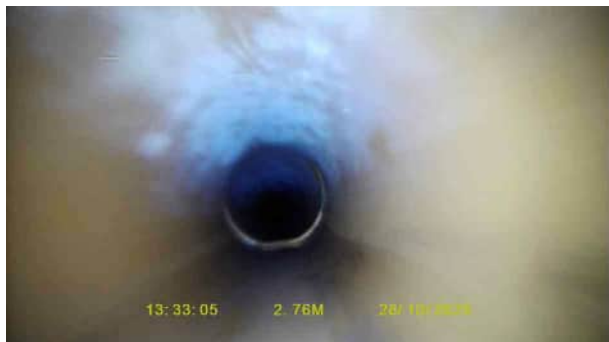
FW5X_9053817d-fad6-48c5-b896-a1d56bd0ecf9_20251112_104229_971.jpg, 00:00:10, 3.20 m Joint displaced, medium
