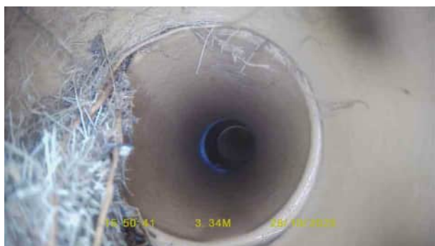
F16X_ca098908-7440-4f91-bfb8-af5343603fbc_20251120_094917_659.jpg, 00:00:17, 3.35 m Roots, mass at joint, 15% cross-sectional area loss
