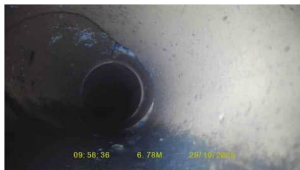
SW8X_106a91c9-6d69-4953-8b4d-d6b8dc7cecd_a_20251120_110445_438.jpg, 00:00:27, 7.00 m Fracture, circumferential at joint from 12 o'clock to 12 o'clock
