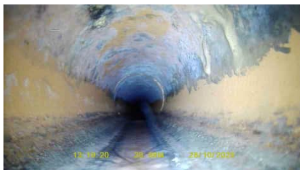
F5X_d6a7aa87-dce6-45ac-9724-88720cfde97b_20251111_152206_594.jpg, 00:00:58, 21.30 m Joint displaced, medium
