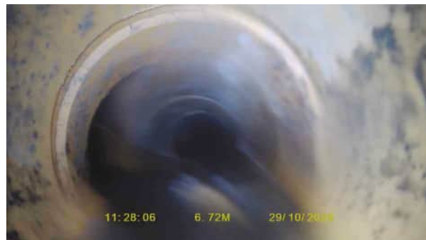
S22X_a7c82911-39fa-47bb-9953-3503c041849e_20251120_132211_885.jpg, 00:00:31, 7.00 m Junction at 9 o'clock, 100mm dia
