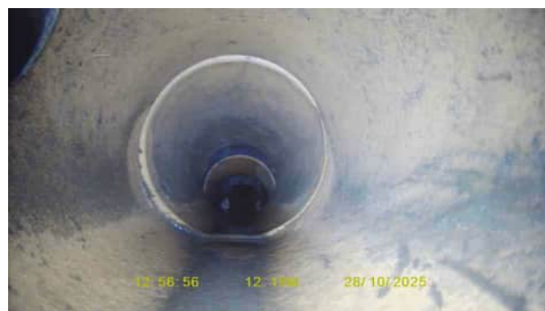
SW4X_76ca052a-4878-4405-91c2-da6a748b62bf_20251105_161536_485.jpg, 00:02:12, 12.30 m Joint displaced, medium
