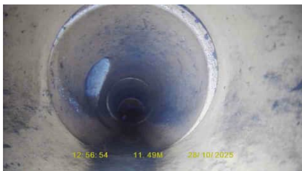
SW4X_0384d613-8e0b-4560-8eaa-1ffee7734846_20251105_161316_891.jpg, 00:02:10, 11.40 m Joint displaced, large
