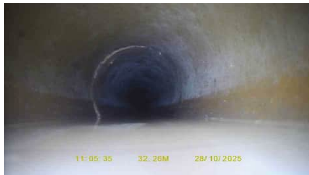
F1X_d374c5be-b6c6-4f32-a187-84de2f0924b3_20251105_14 1840_879.jpg, 00:02:45, 32.50 m Joint displaced, medium
