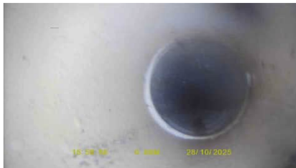
F19X_6afdfd43-a8e3-4970-9bdb-038c5f50a752_20251120_101332_001.jpg, 00:00:04, 0.40 m Joint displaced, medium
