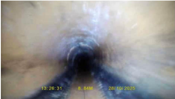
FW10X_489b6e79-5db5-4ef5-a0f8-95d66fbbe097_20251112_094659_471.jpg, 00:00:34, 8.90 m Crack, longitudinal at 12 o'clock
