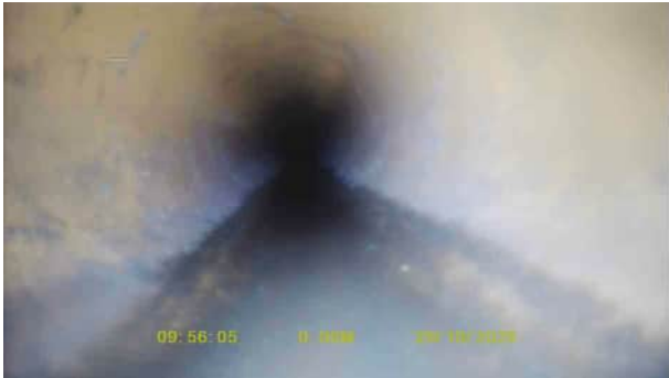
S13X_ebc9fef7-e626-4fdb-8e4f-f7819504d956_20251120_10 5632_720.jpg, 00:00:00, 0.00 m Start node, inspection chamber, reference: SW7
