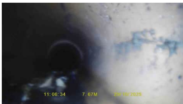
SW11X_56da5348-cdd6-4006-96dd-fee3d40f985_20251120_130437_224.jpg, 00:00:51, 8.35 m Joint displaced, medium
