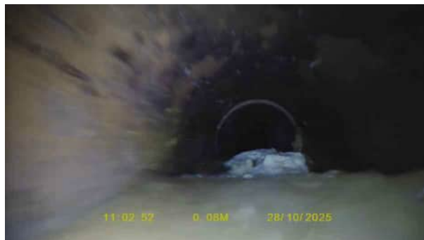
F1X_4c7e71f5-719c-4dc9-94a1-7f3bba4236da_20251105_135027_113.jpg, 00:00:02, 0.10 m Other obstacles from 4 o'clock to 7 o'clock, 30% cross-sectional area loss, Toilet Roll
