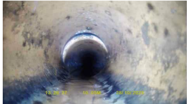
FW10X_35fc7b96-006a-4807-9626-0c2ef77b51d7_20251112_094753_344.jpg, 00:00:40, 10.20 m Joint displaced, large
