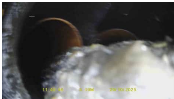
F26X_b94183f1-739c-4493-93b7-b68a8541690c_20251120_132902_276.jpg, 00:00:12, 3.20 m Junction at 9 o'clock, 100mm dia
