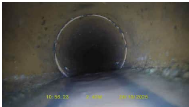
FW3X_a445b793-2a80-4e35-8496-ca9087429080_20251105_132059_614.jpg, 00:00:10, 2.50 m Joint displaced, medium
