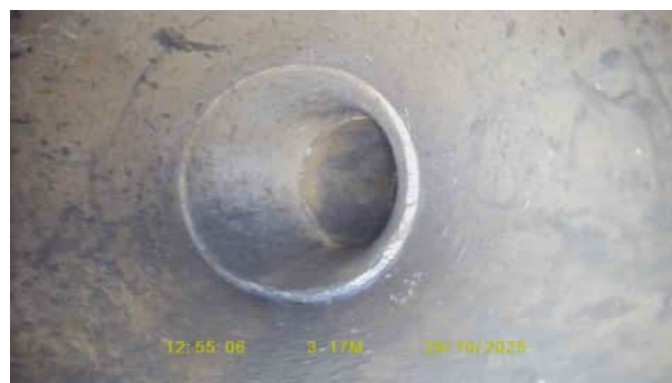
SW4X_3e585ab9-7d0f-44ea-9d1d-10f6a8a65c99_20251105_160023_596.jpg, 00:00:22, 3.30 m Joint displaced, medium
