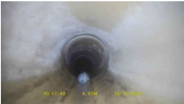
FW13X_60e47147-1baf-41fa-8881-d245d2a19dcf_20251120_123723_383.jpg, 00:00:21, 5.17 m Joint displaced, large
