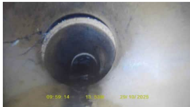
SW8X_69134f3b-dfb0-48c4-a638-60a7a5ee793f_20251120_12009_894.jpg, 00:01:05, 13.80 m Joint displaced, large
