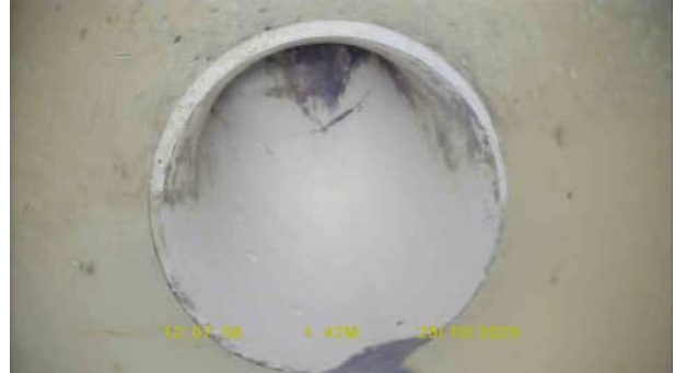
F3X_aa5e5e11-ceed-4417-b385-c2c5321bf1f8_20251105_14 4706_463.jpg, 00:00:14, 1.40 m Finish node, other special chamber, reference: F3, WP
