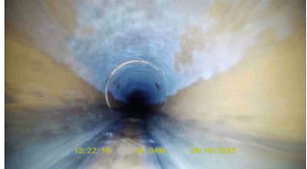
F5X_4f78a5c3-e6c6-4d3a-b391-cc41a5f31005_20251111_15 5138_101.jpg, 00:03:54, 37.00 m Joint displaced, medium
