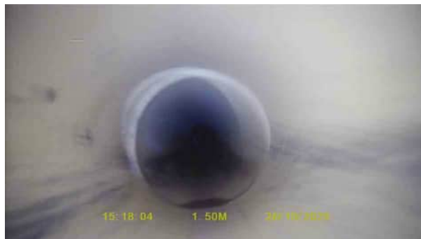
F17X_e672bf31-b12a-43ec-853c-c1446073dc43_20251120_085721_547.jpg, 00:00:58, 1.80 m Joint displaced, medium
