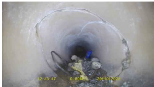
S27X_75b41ab2-d5f4-4b5d-b5e1-61a0704ed9ac_20251120_1 141706_698.jpg, 00:00:06, 0.70 m Fracture, circumferential from 7 o'clock to 5 o'clock
