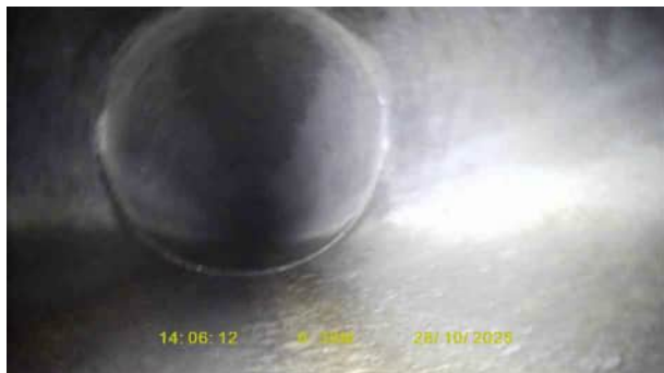
SW6X_8156ae88-9333-4efd-bb9c-f8500dd038ac_20251112_130129_689.jpg, 00:00:22, 6.70 m Joint displaced, medium
