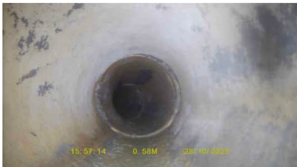
F18X_c7e4496d-2752-4866-8a41-ee8af329f7dc_20251120_095819_872.jpg, 00:00:06, 1.30 m Joint displaced, medium
