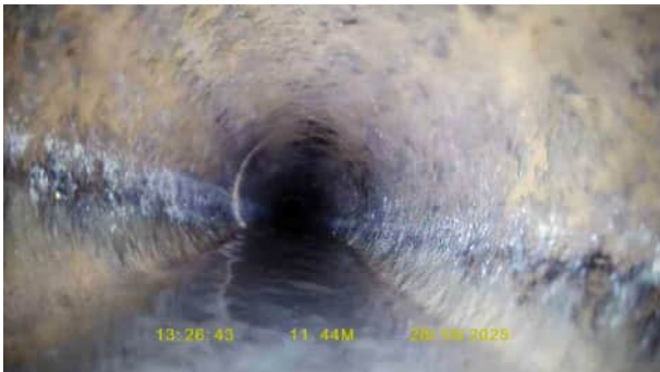
FW10X_db7cfa2-fd05-44a5-9589-2edd2dbbb439_20251112_095209_492.jpg, 00:00:47, 11.50 m Joint displaced, medium
