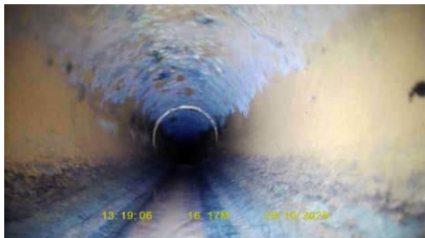
F5X_186ab68e-9783-46da-b64a-9a03585a2133_20251111_151757_964.jpg, 00:00:45, 16.80 m Joint displaced, medium
