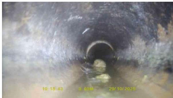
FW11X_233712f4-b549-4f77-92a5-c976eede4891_20251120_113830_811.jpg, 00:00:05, 1.16 m Joint displaced, medium
