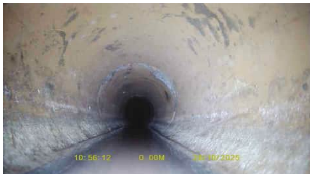
FW3X_f96d133b-4b66-4a8e-bb0a-ab71a3787eff_20251105_131826_068.jpg, 00:00:00, 0.00 m Start node, inspection chamber, reference: FW1
