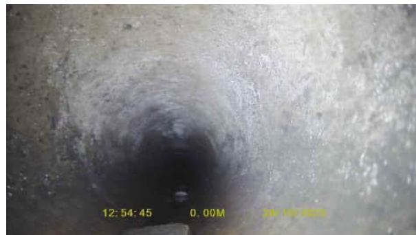
SW4X_e6ad774e-b271-404a-9e09-c6d9f9d401b7_20251105_155337_247.jpg, 00:00:01, 0.10 m Other obstacles, brick or masonry in invert at 6 o'clock, 5% cross-sectional area loss
