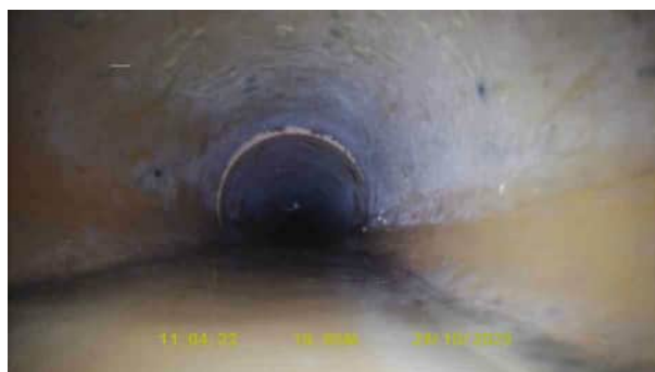
F1X_9a8f4df7-5336-4bc7-b7d3-fb74378dffa_20251105_140809_548.jpg, 00:01:31, 20.20 m Joint displaced, medium
