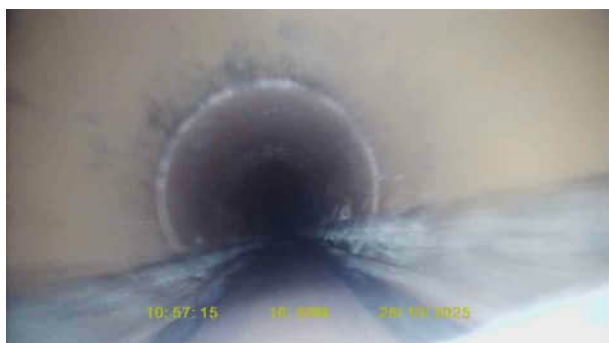
FW3X_d7ff3a7-2b1a-47aa-9810-a03255046e8f_20251105_132620_238.jpg, 00:01:02, 16.20 m Joint displaced, medium
