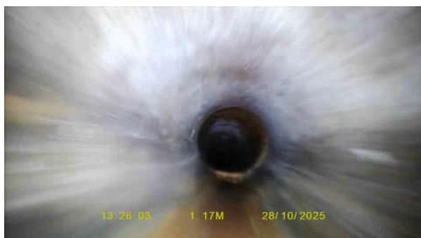
FW10X_c054f2e3-c390-4d55-a0b2-094de3b03151_20251112_092657_521.jpg, 00:00:07, 1.70 m Crack, circumferential from 12 o'clock to 12 o'clock
