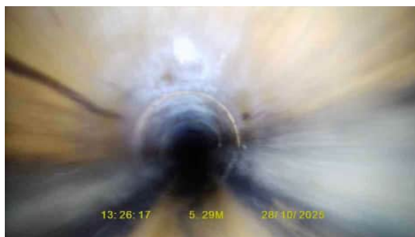
FW10X_25132659-a6d9-47d5-86e5-cdcfbf520643_20251112_093850_013.jpg, 00:00:20, 5.60 m Crack, circumferential from 12 o'clock to 12 o'clock
