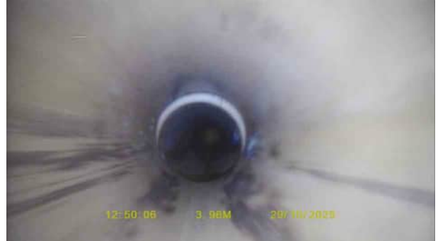
F30X_25466a79-dbe6-4cfb-8afa-e0c51efdd0e6_20251120_142507_728.jpg, 00:00:17, 4.40 m Joint displaced, large
