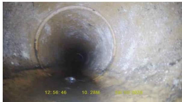
SW4X_d7e1b6aa-48f1-4d97-9785-92e518df6c6a_20251105_161238_563.jpg, 00:02:02, 10.20 m Joint displaced, medium
