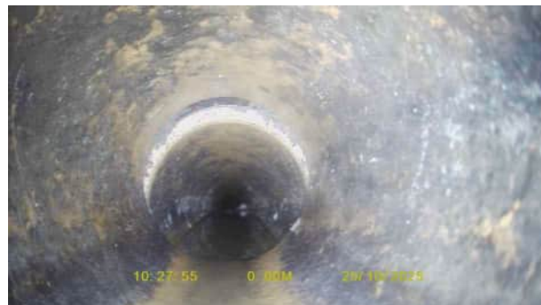
FW13X_ab5e0ca1-c957-4deb-96ab-785ed34d6408_20251120_114927_807.jpg, 00:00:00, 0.60 m Joint displaced, large
