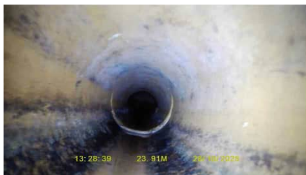
FW10X_2adfbab0-1aa4-4164-9016-1c85cfea51b3_20251112_103340_900.jpg, 00:02:43, 24.10 m Joint displaced, medium
