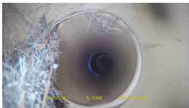
F16X_055a04e2-d450-4994-b564-6fbf0796fd2d_20251120_094943_303.jpg, 00:00:17, 3.40 m Cracks, spiral at joint from 7 o'clock to 11 o'clock
