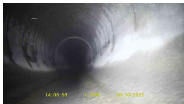
SW6X_0364a2c1-1853-4d7a-90ea-fe45b66305ba_20251112_125949_646.jpg, 00:00:08, 2.60 m Joint displaced, medium
