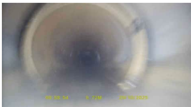
SW8X_afbda8f2-88bc-4c1a-889e-648277c45fe1_20251120_110621_345.jpg, 00:00:45, 10.15 m Joint displaced, medium
