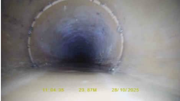
F1X_7ef61e4e-ab48-4070-99f4-73e215dc79c3_20251105_141016_166.jpg, 00:01:45, 23.75 m Joint displaced, medium
