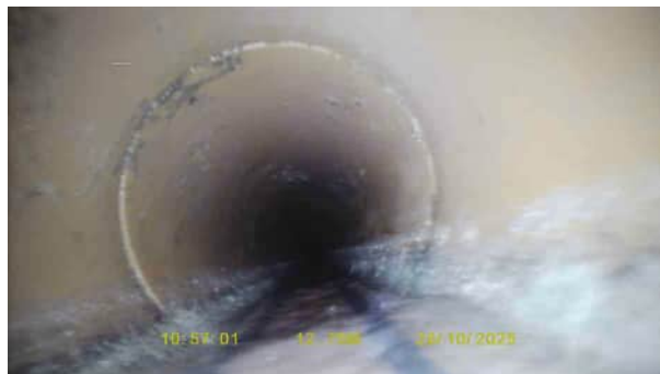
FW3X_242d2110-7232-4526-a57d-6bedde13ea2d_20251105_132508_165.jpg, 00:00:48, 12.80 m Joint displaced, medium
