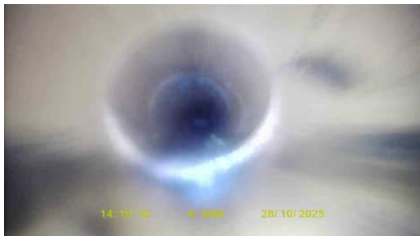
SW7X_166bd7a7-3827-45ca-9213-111b38a73bc2_20251112_150617_885.jpg, 00:00:30, 7.10 m Crack, circumferential from 12 o'clock to 12 o'clock
