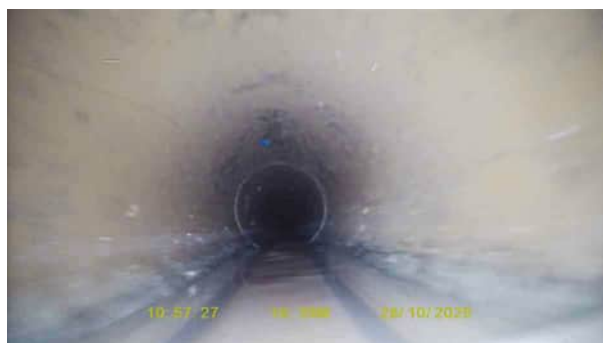
FW3X_ee52754c-29d2-4ad9-82b1-c68fedff838d_20251105_132852_886.jpg, 00:01:15, 19.30 m Crack, longitudinal at 10 o'clock
