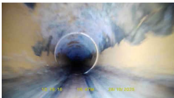
F5X_1dff66bd-032e-4a8e-bacd-66fb24f26518_20251111_152044_033.jpg, 00:00:54, 19.70 m Joint displaced, medium
