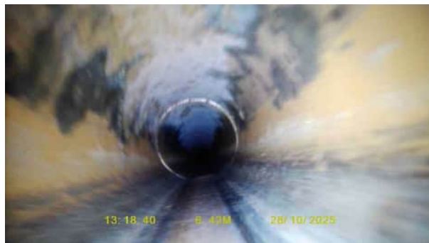
F5X_7d85b6ee-c78c-444c-a187-0e71105c7bbc_20251111_151402_932.jpg, 00:00:18, 7.00 m Joint displaced, medium
