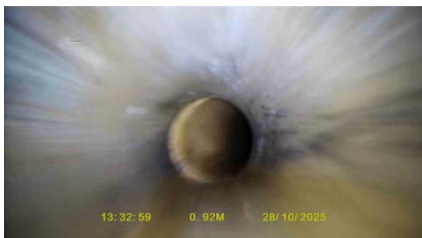
FW5X_c14c5f38-df04-489c-bb58-9c5b14575b02_20251112_104120_606.jpg, 00:00:04, 1.00 m Joint displaced, large
