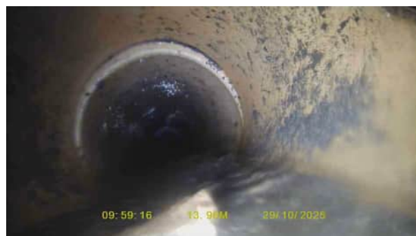
SW8X_48ac1778-fd06-46a2-8c1f-0e6059bf6c79_20251120_12056_486.jpg, 00:01:07, 14.25 m Joint displaced, medium
