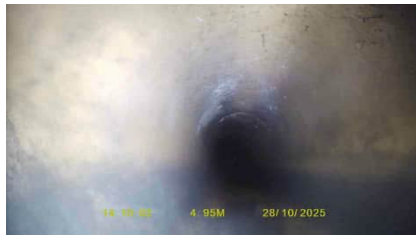
SW7X_ced3cadb-0bb5-4313-9763-cc7a7c42bef9_20251112_145649_468.jpg, 00:00:23, 5.40 m Crack, circumferential from 12 o'clock to 12 o'clock
