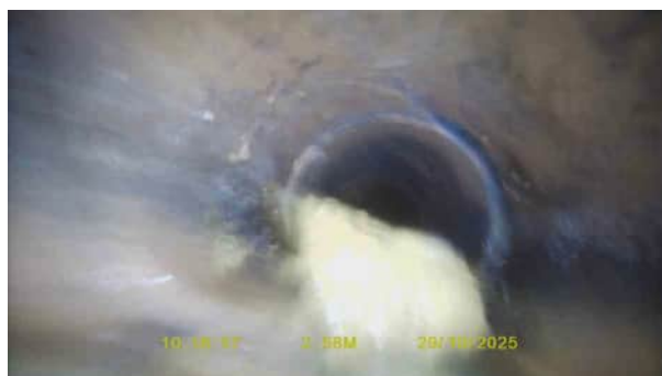
FW11X_6a9dff3-148d-45b8-b387-6fbfaa13c859_20251120_114008_688.jpg, 00:00:18, 2.30 m Fracture, spiral from 10 o'clock to 8 o'clock
