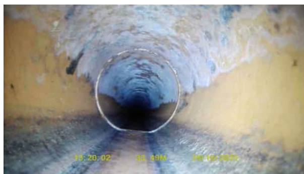
F5X_0f6711bb-da22-4f6b-844e-7ba240578ac5_20251111_15 4255_973.jpg, 00:01:40, 34.00 m Joint displaced, medium
