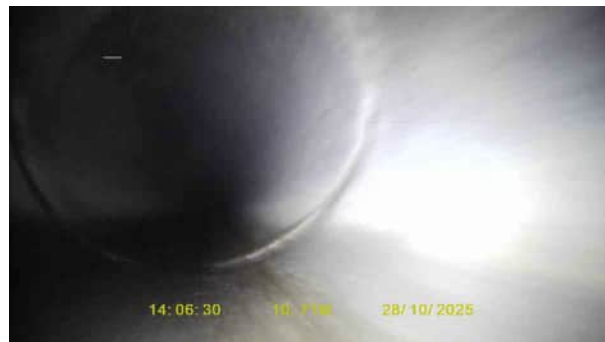
SW6X_9809e080-7b3f-46eb-9453-336645aa06d1_20251112_130252_993.jpg, 00:00:40, 11.00 m Joint displaced, medium
