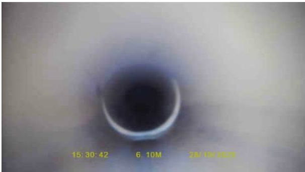
FW8X_678862db-929b-46e8-b434-01713861fd8f_20251120_091429_518.jpg, 00:00:20, 6.35 m Joint displaced, medium
