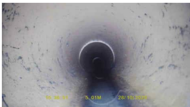
SW12X_3930fb8c-112a-4c4a-978d-c214271d1fcf_20251120_092927_788.jpg, 00:00:25, 5.25 m Joint displaced, medium
