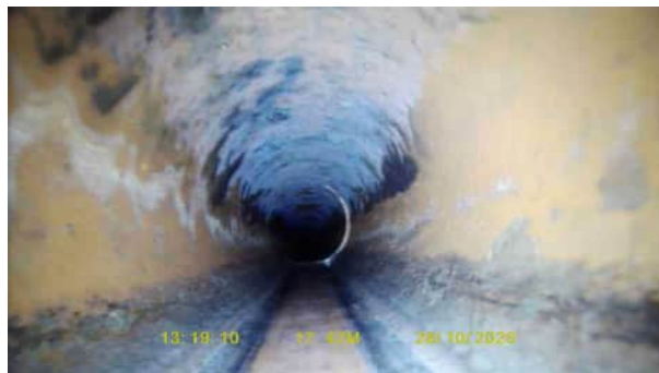
F5X_b261c99f-01b4-4737-b120-e29244078c5d_20251111_151905_154.jpg, 00:00:49, 18.40 m Joint displaced, medium
