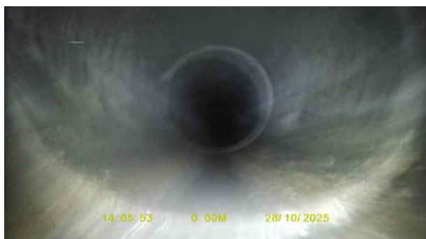
SW6X_0dbe22f1-c6ad-4f60-8883-99275f9d9ee6_20251112_125843_407.jpg, 00:00:03, 0.70 m Joint displaced, medium
