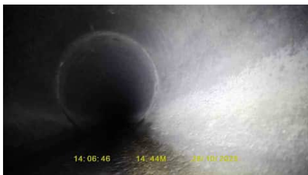
SW6X_010c3b8e-ebd8-4f97-b7f4-cfd7704ee0b7_20251112_130710_801.jpg, 00:00:57, 14.70 m Joint displaced, medium
