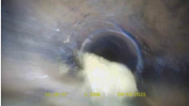
FW11X_26d85041-8c72-4dde-a82d-4ce203946c4a_20251120_114026_559.jpg, 00:00:18, 2.60 m Joint displaced, large
