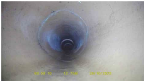
SW8X_1e420b4b-68cd-4a27-bdd6-f47a0e51f55b_20251120_111411_622.jpg, 00:01:00, 12.90 m Crack, circumferential from 12 o'clock to 12 o'clock
