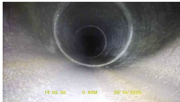
SW6X_cf6c720b-8193-4c25-8249-174885ec6e19_20251112_125747_867.jpg, 00:00:01, 0.20 m Joint displaced, medium
