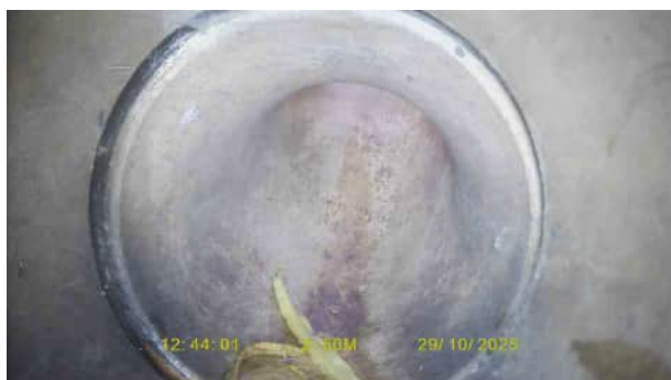
S27X_879180dd-aa87-40f4-9a13-efa9ee612d65_20251120_1 41806_059.jpg, 00:00:20, 2.50 m Finish node, other special chamber, reference: S27, RWP
