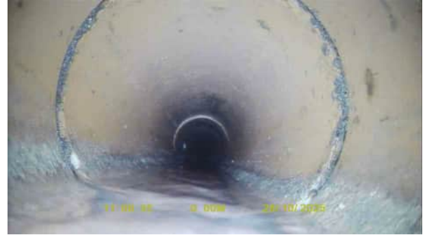
FW1X_bb6485bd-548d-4be5-91c5-705dffaed8c2_20251105_142555_498.jpg, 00:00:00, 0.10 m Joint displaced, medium
