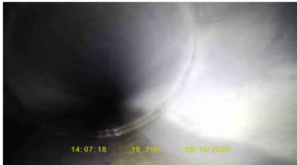
SW6X_92c50ce9-9d5d-435c-8de1-50a8ed6cc66f_20251112_131701_226.jpg, 00:01:28, 19.30 m Joint displaced, medium
