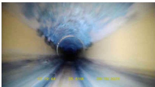
F5X_a9c42148-3f50-4634-a154-bce27f79a3a9_20251111_15 3305_087.jpg, 00:01:22, 29.00 m Joint displaced, medium
