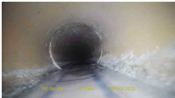
FW3X_e09411e4-4c7b-4c1b-85fa-4bc1ed0eae81_20251105_132408_611.jpg, 00:00:36, 9.30 m Joint displaced, medium
