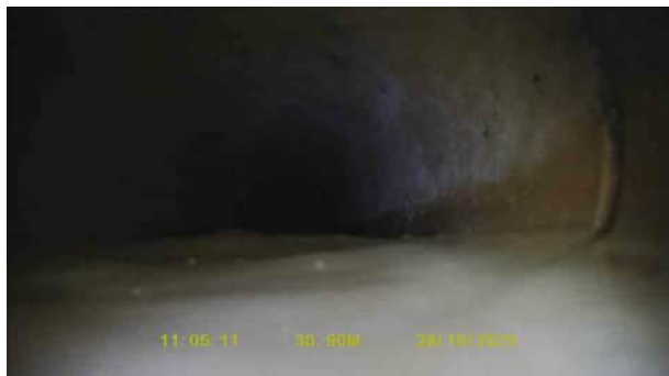
F1X_d18718f8-3ad9-41a6-966c-4f6e2f15b3b4_20251105_14 1719_174.jpg, 00:02:21, 31.00 m Joint displaced, medium
