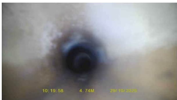
F21X_074d1524-77c2-4efc-b2b1-ea565621575a_20251120_1 14331_298.jpg, 00:00:21, 5.20 m Junction at 9 o'clock, 100mm dia
