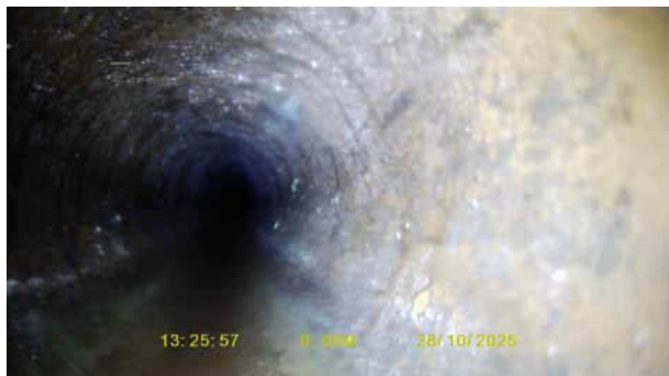
FW10X_c7c03ad1-0c23-4449-97d2-95f42c85b789_20251112_091930_056.jpg, 00:00:00, 0.00 m Start node, inspection chamber, reference: FW3
