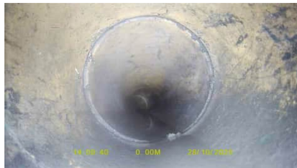
SW7X_a791ce40-ffb1-4423-b40c-b3869c745efc_20251112_1 32819_891.jpg, 00:00:00, 0.20 m Joint displaced, medium
