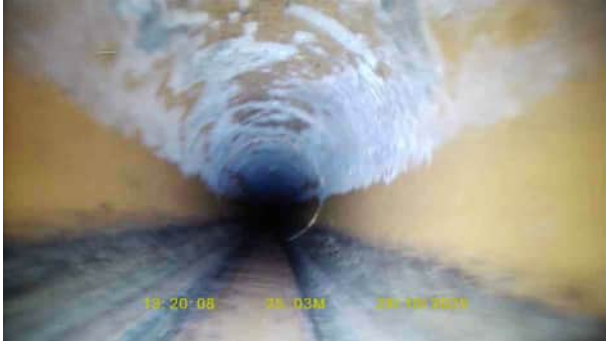
F5X_8bb544a3-cf0a-48fa-a29e-19c2b8d823d8_20251111_15 4407_360.jpg, 00:01:47, 35.30 m Joint displaced, medium
