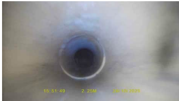
FW9X_99a7e607-1d8d-4e43-a25e-42f48c057b03_20251120_095504_821.jpg, 00:00:11, 2.50 m Joint displaced, medium
