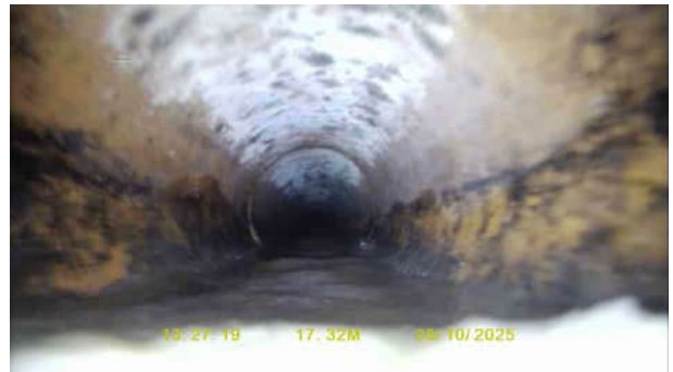
FW10X_81088a87-189d-4eeb-b334-c13ca4e55463_20251112_101705_448.jpg, 00:01:23, 17.60 m Joint displaced, medium
