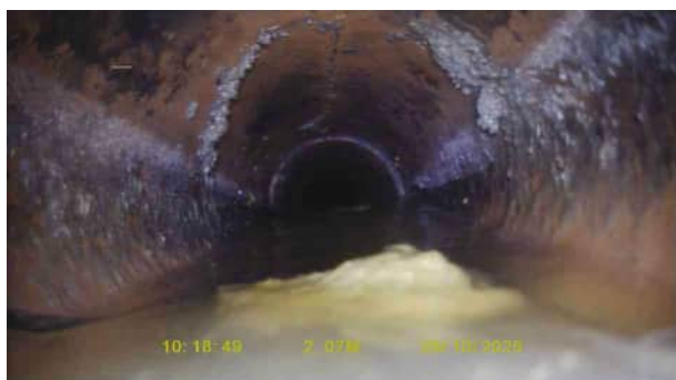
FW11X_f4fa0d8a-fa89-4324-a3b1-3c5d7799767d_20251120_113918_841.jpg, 00:00:10, 2.10 m Crack, longitudinal at joint at 12 o'clock
