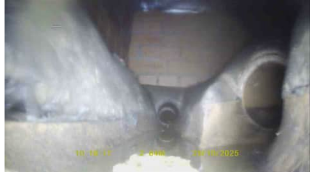
FW11X_d164bb39-a2ff-4201-9e3c-136bcbe43cfd_20251120_114043_092.jpg, 00:00:38, 2.90 m Finish node, inspection chamber, reference: FW11
