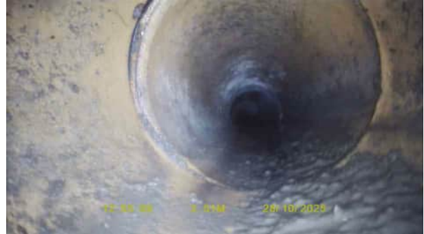
SW4X_0bff2009-5ac1-4039-917c-d5662af05af0_20251105_160209_044.jpg, 00:00:25, 3.80 m Joint displaced, large
