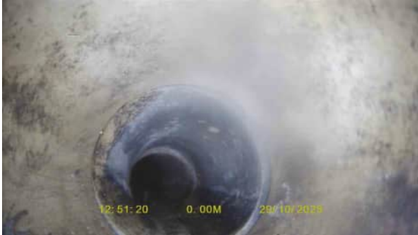
FW15X_842db7ba-f857-4f86-9676-71779cf196c2_20251120_142648_489.jpg, 00:00:00, 0.00 m Start node, inspection chamber, reference: FW15
