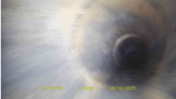
SW4X_ac15fd9d-b3cb-408d-9338-c22110519835_20251105_160126_610.jpg, 00:00:24, 3.40 m Joint displaced, medium
