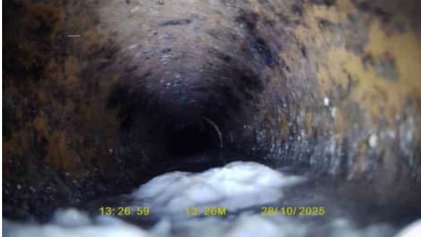
FW10X_895e0a00-141f-4287-92d8-25938a8ac141_20251112_100631_338.jpg, 00:01:03, 14.00 m Joint displaced, medium
