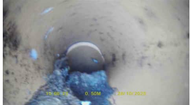
S9X_51322b8a-ae6d-43bd-9632-2d49537fac94_20251120_082840_553.jpg, 00:00:09, 0.60 m Joint displaced, medium
