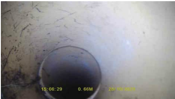
S9X_cac218d6-5050-4ac9-95ae-9cfbb463f60c_20251120_082837_710.jpg, 00:00:14, 0.80 m Joint displaced, medium
