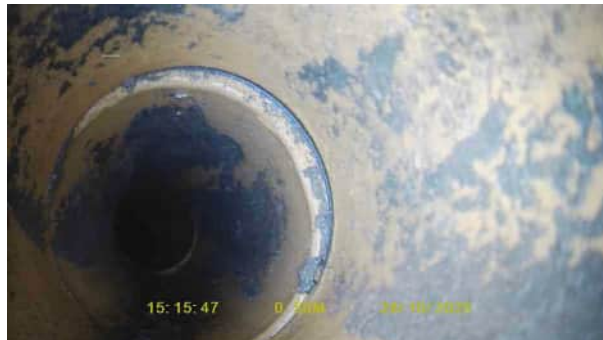
F12X_1414158c-9cc2-454c-81ca-7f4db72234b7_20251120_084949_077.jpg, 00:00:10, 0.60 m Joint displaced, large
