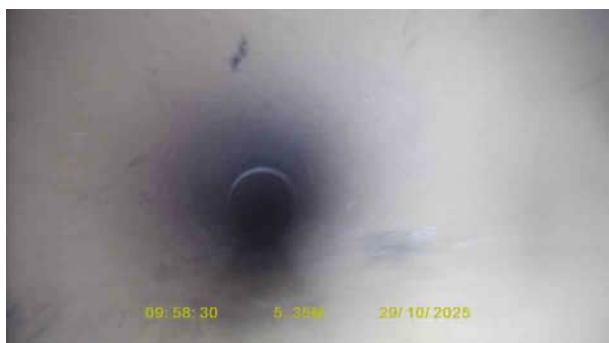
SW8X_9f9d6bec-d13b-491e-9f74-bff07f54fa4e_20251120_110401_438.jpg, 00:00:21, 6.10 m Joint displaced, medium
