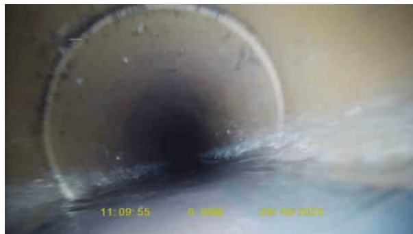
FW1X_d7d02a65-f620-4ce9-b720-8c0dc29dab83_20251105_142949_117.jpg, 00:00:19, 6.10 m Joint displaced, medium
