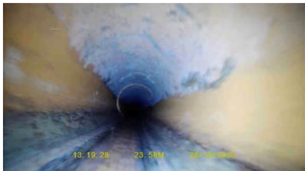
F5X_51817b73-068f-4963-a431-87c08025ca0e_20251111_15 2352_977.jpg, 00:01:07, 24.50 m Joint displaced, medium
