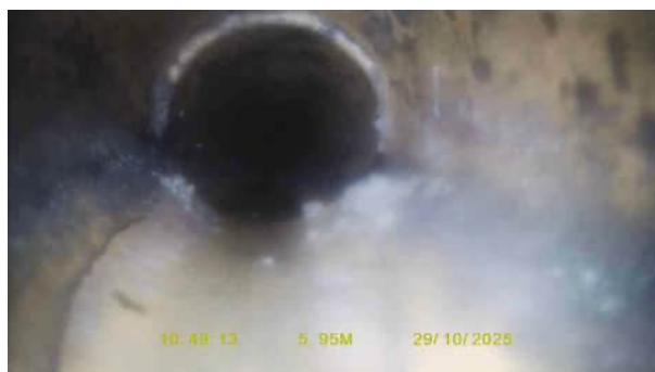
FW12AX_38cf8bb1-48c1-46a1-8f4c-39dde8b70faf_20251120_124045_174.jpg, 00:00:28, 6.20 m Joint displaced, medium
