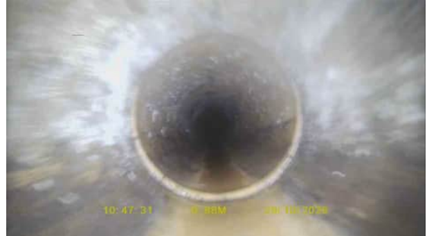
FW13X_3edb8a71-4c39-4554-9429-70adf5819015_20251120_123654_775.jpg, 00:00:04, 0.90 m Joint displaced, medium
