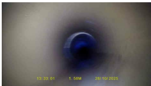
FW5X_d3886a20-5566-4197-b158-1086b139d2d7_20251112_104200_300.jpg, 00:00:06, 1.90 m Joint displaced, medium
