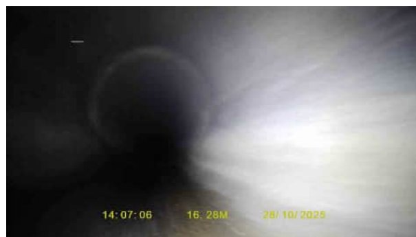
SW6X_f108b99a-c7f9-4d56-80d3-ae6fcf5583d6_20251112_130822_026.jpg, 00:01:17, 17.00 m Joint displaced, medium
