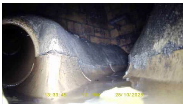
FW5X_514029e4-114e-4ae3-9d41-7c7f72d4af35_20251112_105315_471.jpg, 00:00:51, 12.80 m Finish node, inspection chamber, reference: FW5
