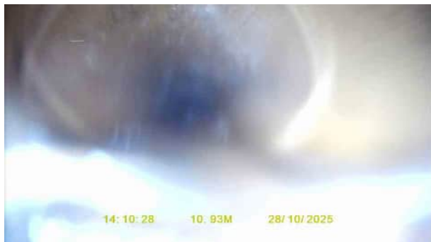
SW7X_e8edcfe6-8ef0-4902-81ae-3bac1123c90b_20251112_153137_115.jpg, 00:00:49, 11.50 m Joint displaced, medium
