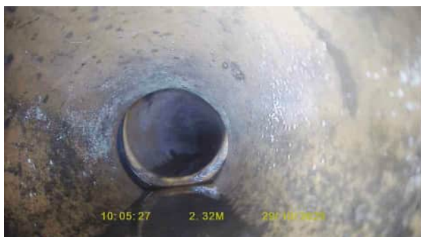
S15X_55d7f610-1805-4625-aa96-faa487de34b9_20251120_1 12929_534.jpg, 00:00:17, 2.85 m Joint displaced, large
