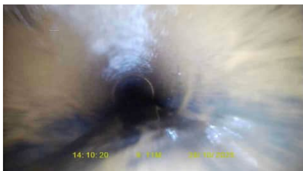
SW7X_3fc92219-8920-4a3a-a375-ff03a9f21cbc_20251112_152551_534.jpg, 00:00:41, 9.60 m Joint displaced, medium
