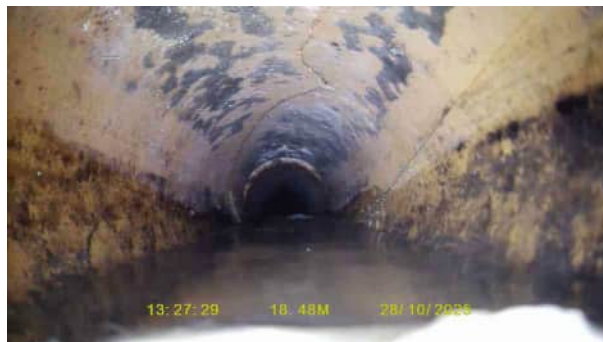
FW10X_392efeec-5fbf-4afe-8198-d4e8d0fd9419_20251112_101920_471.jpg, 00:01:32, 18.65 m Cracks, spiral from 9 o'clock to 12 o'clock
