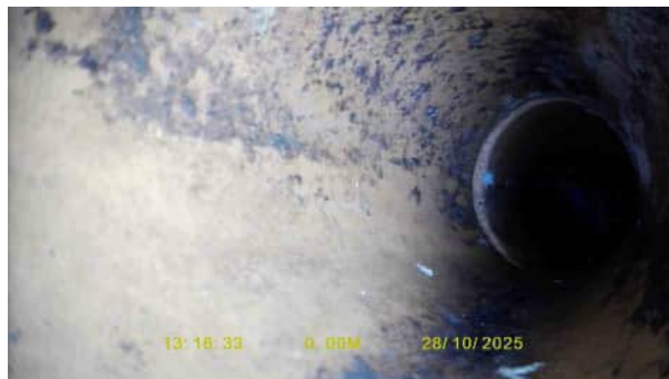
FW4X_b0ed26bb-f7b6-410a-bfa3-1cb3b7f78ce0_20251111_143723_272.jpg, 00:00:01, 0.30 m Joint displaced, medium
