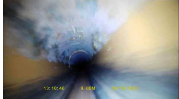
F5X_f2ad8170-38f7-4875-990a-c4721f5776df_20251111_151 502_630.jpg, 00:00:27, 10.20 m Joint displaced, medium
