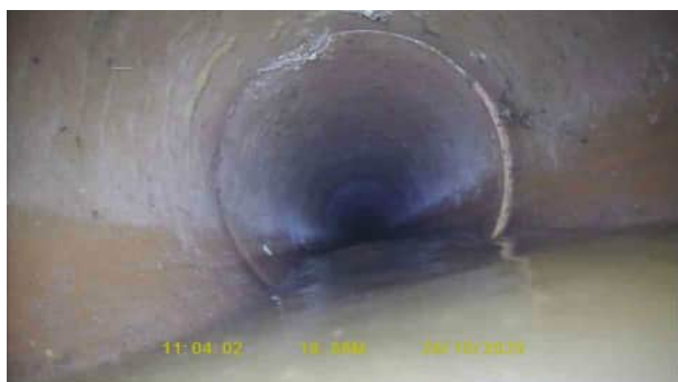
F1X_c6f60755-7b2a-4aaa-9ca6-c47bde1e8880_20251105_140504_454.jpg, 00:01:12, 19.00 m Joint displaced, medium
