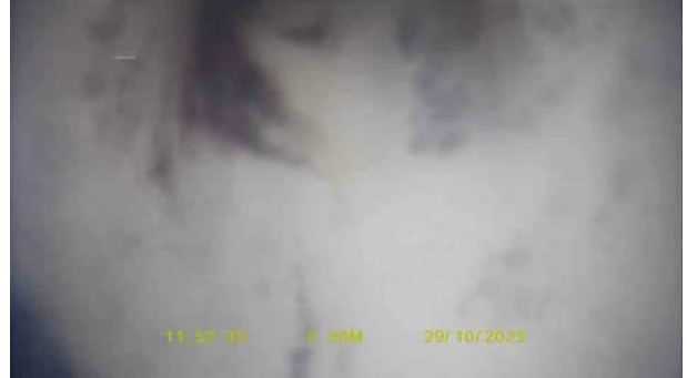
F28X_738219f8-cc74-4289-89f4-c76189dc7ca2_20251120_134021_850.jpg, 00:00:13, 2.50 m Finish node, other special chamber, reference: F28, WP
