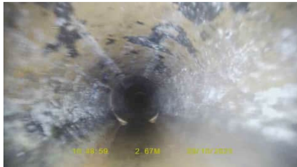
FW12AX_4bd3fe5a-ad99-4f7d-aa8f-49db1b421f49_20251120_124011_429.jpg, 00:00:14, 3.20 m Joint displaced, medium
