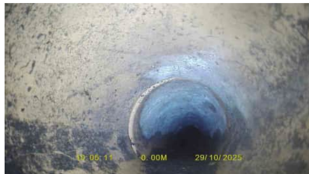
S15X_3a5e1c1c-1ba4-4a48-b102-4824188774b1_20251120_1 112808_203.jpg, 00:00:00, 0.30 m Joint displaced, medium
