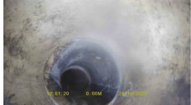
FW15X_ec53d5a4-d240-470e-b5b4-b19574d2842b_20251120_142707_026.jpg, 00:00:00, 0.10 m Joint displaced, medium
