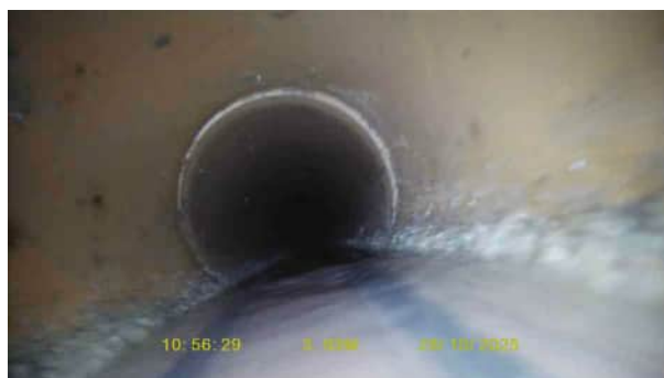
FW3X_9551a688-1181-4b2f-90e4-8d48369dc648_20251105_132245_394.jpg, 00:00:16, 5.90 m Joint displaced, medium
