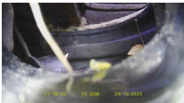
S21X_5a8501db-d797-45fa-9fdc-cfcf8017c6e0_20251120_13 1651_008.jpg, 00:01:01, 13.00 m Finish node, gully, reference: S21
