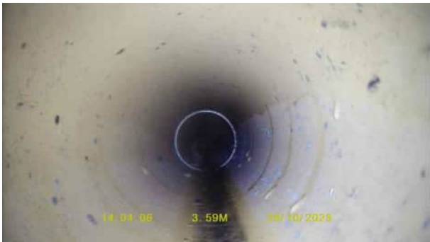
S4X_9b052903-a3b1-4167-956a-5e1d06de5878_20251112_1 21130_284.jpg, 00:00:16, 4.00 m Joint displaced, medium
