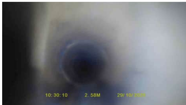
F23X_4ca446dc-c1da-45ed-a3a8-5f3963ff91ea_20251120_115644_807.jpg, 00:00:10, 2.50 m Junction at 9 o'clock, 100mm dia
