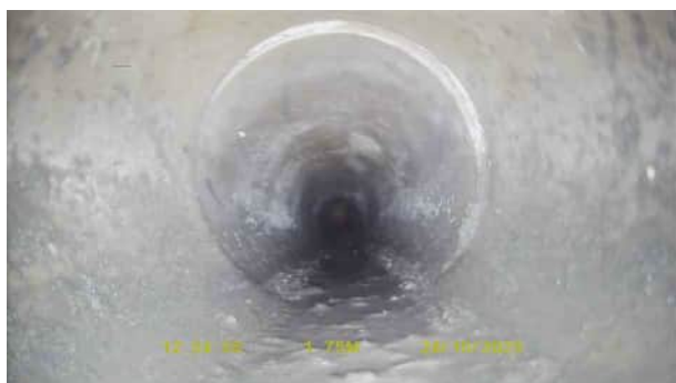
SW4X_93ebfe04-d637-4380-8188-10eb1cf44634_20251105_155848_749.jpg, 00:00:11, 1.80 m Joint displaced, medium
