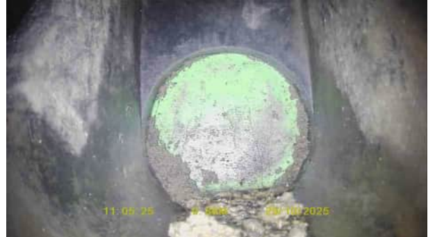
SW9X_7e3c8eb0-5ef5-43ba-8ebd-92dd69d70676_20251120_125931_790.jpg, 00:00:13, 0.80 m Finish node, inspection chamber, reference: SW9
