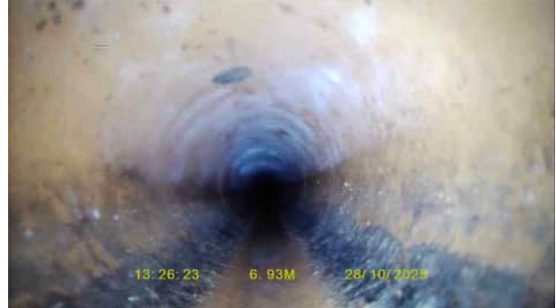
FW10X_def1cc6c-2b96-405c-a940-7b1131057b74_20251112_094113_288.jpg, 00:00:27, 7.80 m Crack, circumferential from 12 o'clock to 12 o'clock
