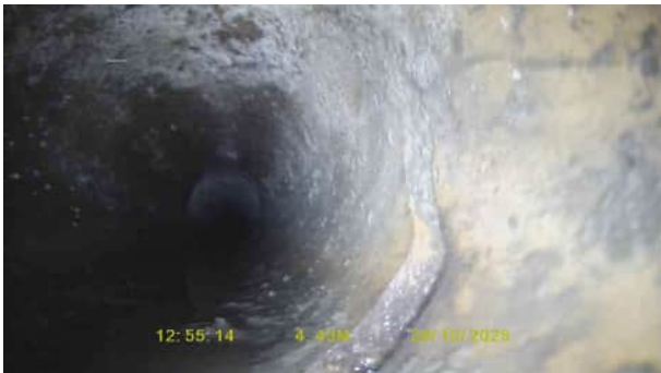
SW4X_fac33b99-32e3-441c-af58-b6fa2db43352_20251120_075201_800.jpg, 00:00:31, 4.45 m Joint displaced, large
