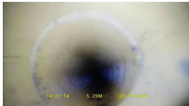
SW5X_692a298b-7fe1-42d5-bdc9-f98913986d22_20251113_090120_904.jpg, 00:00:54, 5.40 m Joint displaced, medium
