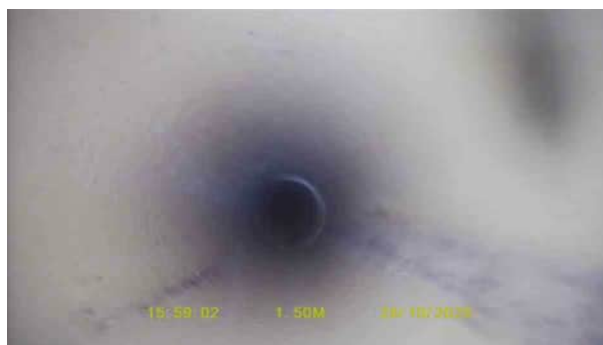
F19X_350fa825-05e1-4b2b-bbbd-cd063b224118_20251120_101422_908.jpg, 00:00:08, 2.20 m Joint displaced, medium
