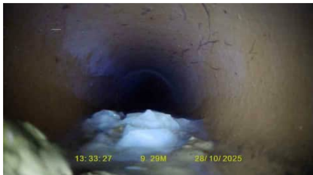
FW5X_e68be286-3fb0-4a62-9ec8-9cdf7f42df51_20251112_104940_946.jpg, 00:00:32, 9.50 m Joint displaced, medium
