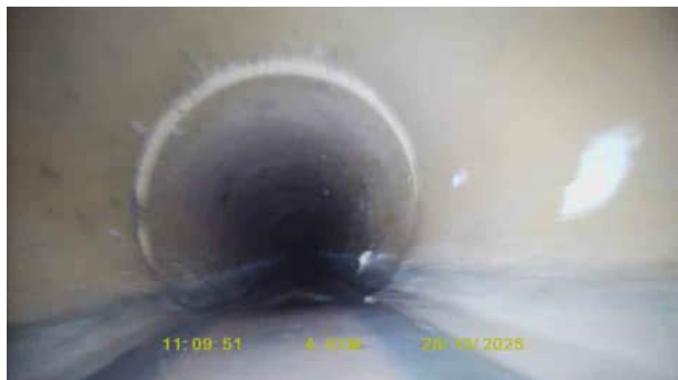
FW1X_5b273742-cf5f-47da-959e-2f2496b86c59_20251105_142910_140.jpg, 00:00:14, 4.10 m Joint displaced, medium
