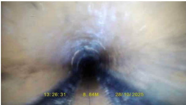
FW10X_330f6a9a-05a9-4ac3-b717-c846faa110f7_20251112_094539_645.jpg, 00:00:34, 8.90 m Crack, longitudinal at 5 o'clock
