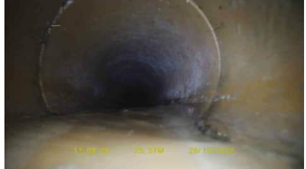
F1X_14970dac-c4da-4082-b7ad-68042f41e63c_20251105_141203_411.jpg, 00:01:51, 25.40 m Joint displaced, medium
