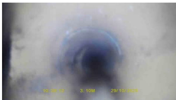
F23X_d04bb9c2-0c81-47be-b983-2a59bd8b7214_20251120_115745_849.jpg, 00:00:13, 3.35 m Junction at 9 o'clock, 100mm dia
