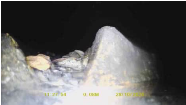
S1X_ccb87a47-8972-4be7-bc84-d2fdd4963a08_20251105_145756_969.jpg, 00:00:17, 0.25 m Survey abandoned, Debris
