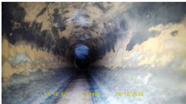
F5X_1ea38ad1-2927-441f-9033-f555f4d9b313_20251111_151311_267.jpg, 00:00:11, 3.80 m Joint displaced, medium
