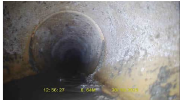
SW4X_344ace52-f5a3-4b4e-a2e0-49438cc7dd4b_20251105_160948_443.jpg, 00:01:43, 6.80 m Joint displaced, medium
