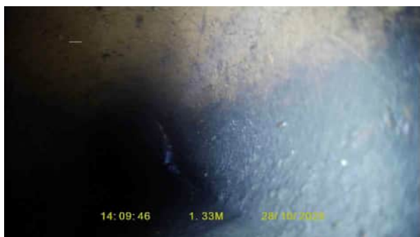
SW7X_8cde98ef-dcf8-43ac-b0e6-0aa8b5c4d3ea_20251112_1 144724_058.jpg, 00:00:06, 1.80 m Joint displaced, large
