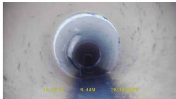
SW12X_708f9320-0168-4373-bc60-1342c6975554_20251120_093025_331.jpg, 00:00:31, 7.30 m Joint displaced, medium
