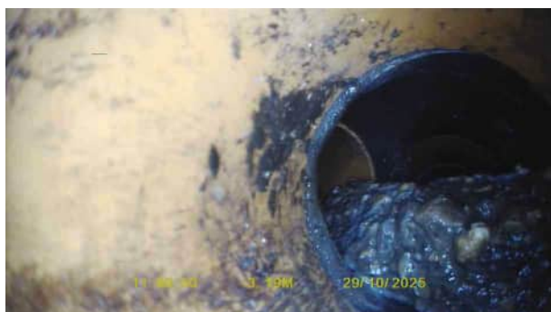
F26X_96c58a51-cfb6-4bba-8549-2484045e34fa_20251120_132918_009.jpg, 00:00:17, 3.20 m Survey abandoned, Silt
