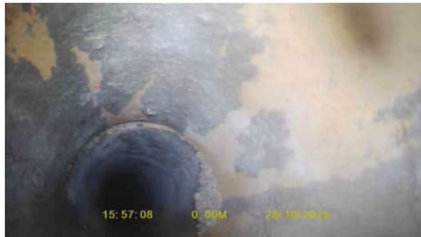
F18X_71e8331f-eacb-4d38-967e-dfb9aac1f9a7_20251120_095755_996.jpg, 00:00:00, 0.15 m Joint displaced, medium
