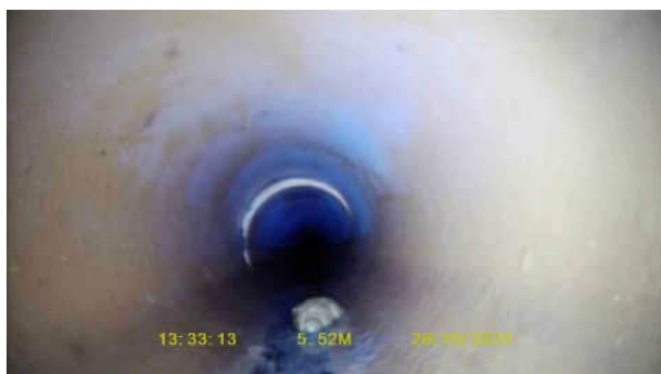
FW5X_1629d8bf-9f25-4cea-9d51-af0238f9ded7_20251112_104334_417.jpg, 00:00:18, 5.80 m Joint displaced, large
