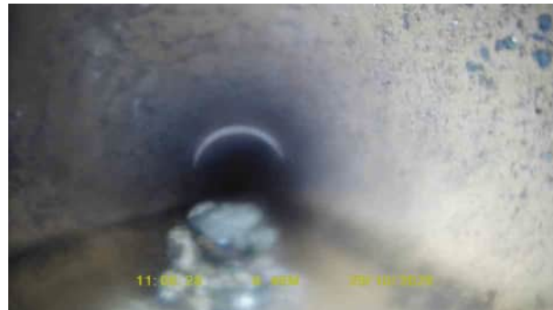
SW11X_a4ce1147-b739-468c-8bb1-2dba0af452e1_20251120_130353_190.jpg, 00:00:45, 7.20 m Joint displaced, large
