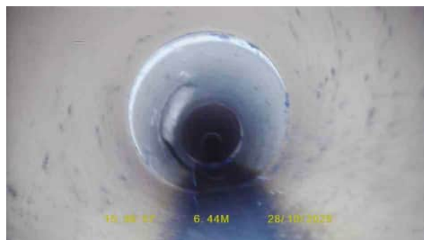
SW12X_bd5a758e-b7a6-44c0-a9df-91213b054292_20251120_092950_452.jpg, 00:00:31, 6.80 m Joint displaced, large
