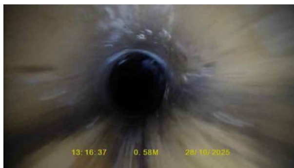
FW4X_2ac60ace-1e68-4b42-82f6-1e6de404bb26_20251111_144129_445.jpg, 00:00:04, 0.90 m Joint displaced, medium
