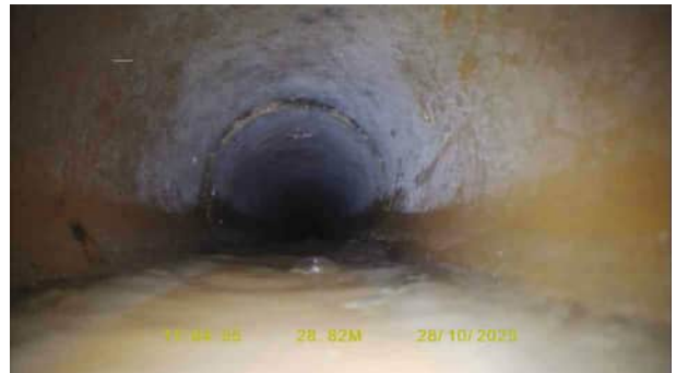
F1X_18dca5ae-c488-4489-8fb3-59bc18f92f6b_20251105_141543_239.jpg, 00:02:05, 29.00 m Joint displaced, medium
