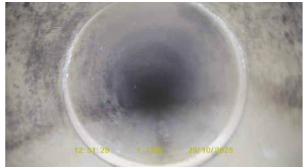
FW15X_5751b8b2-d548-4040-93d6-f1d89f78612b_20251120_142745_986.jpg, 00:00:08, 1.81 m Joint displaced, medium
