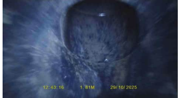
S26X_958fc31a-472a-4ef3-a377-b81b35ef4e35_20251120_160757_371.jpg, 00:00:09, 1.85 m Finish node, other special chamber, reference: S26, RWP
