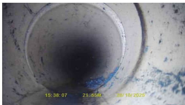
SW12X_a758d0b9-8bcb-4146-9748-1725cf15742c_20251120_093303_228.jpg, 00:01:41, 21.70 m Joint displaced, large
