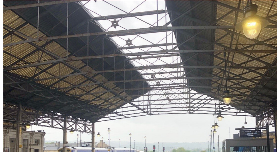
Figure 4.1.6a: Retained Roof A existing lighting scheme
