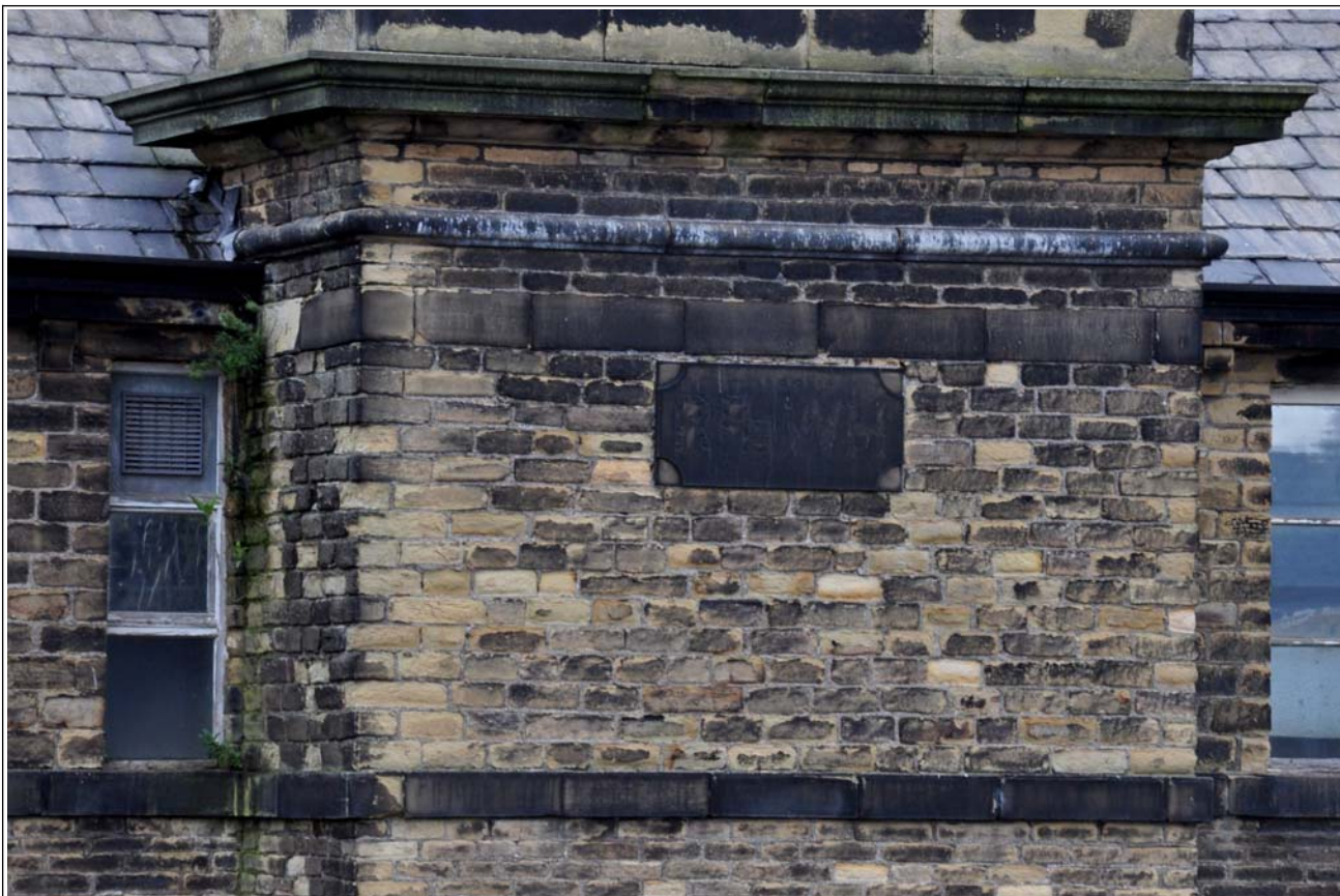
12: Building B (spinning block): top of tower in south elevation, with initialled stone "R&WH"
