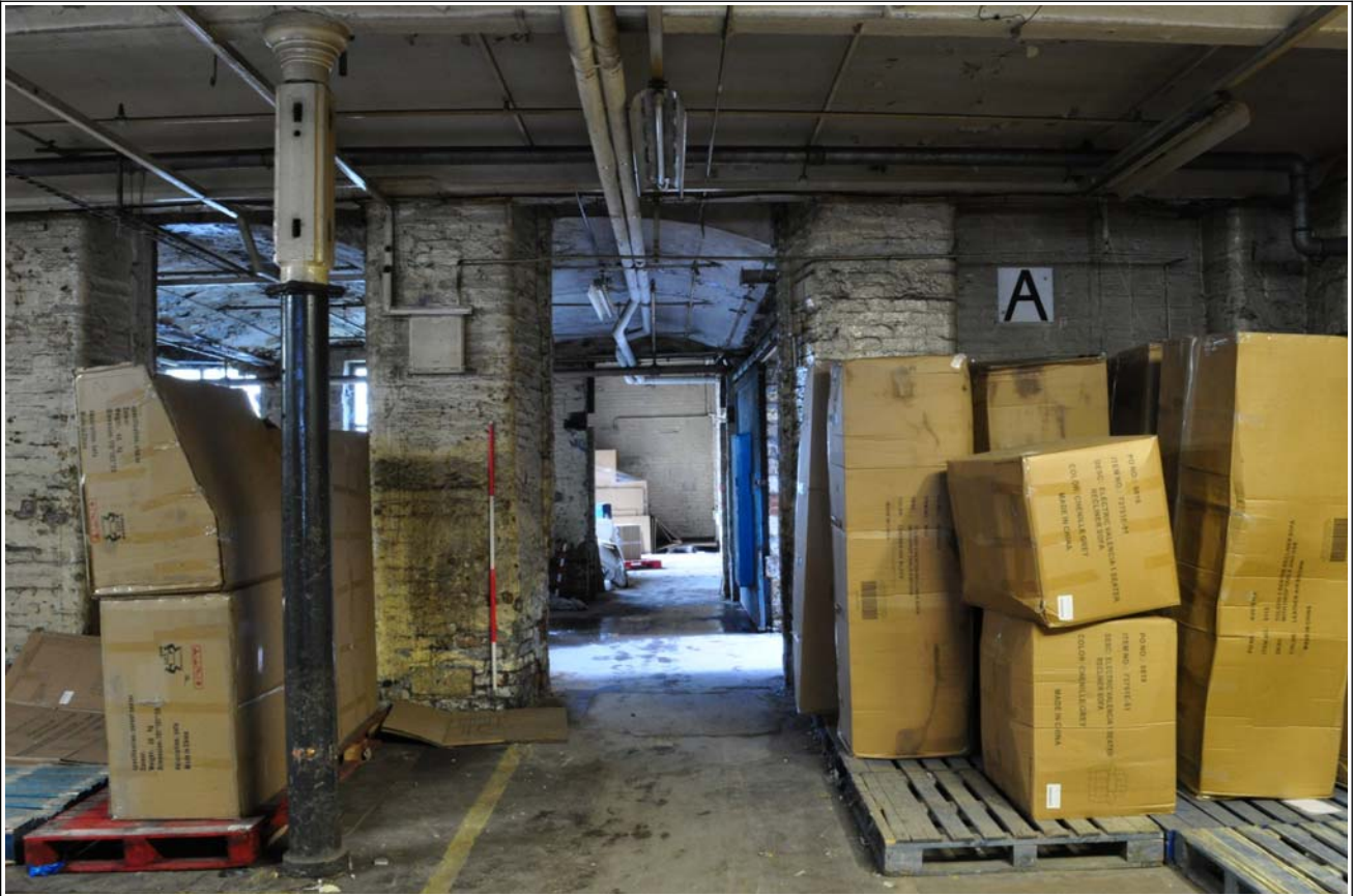
43: Building B (spinning block): doorway (former window) to west extension, ground floor
