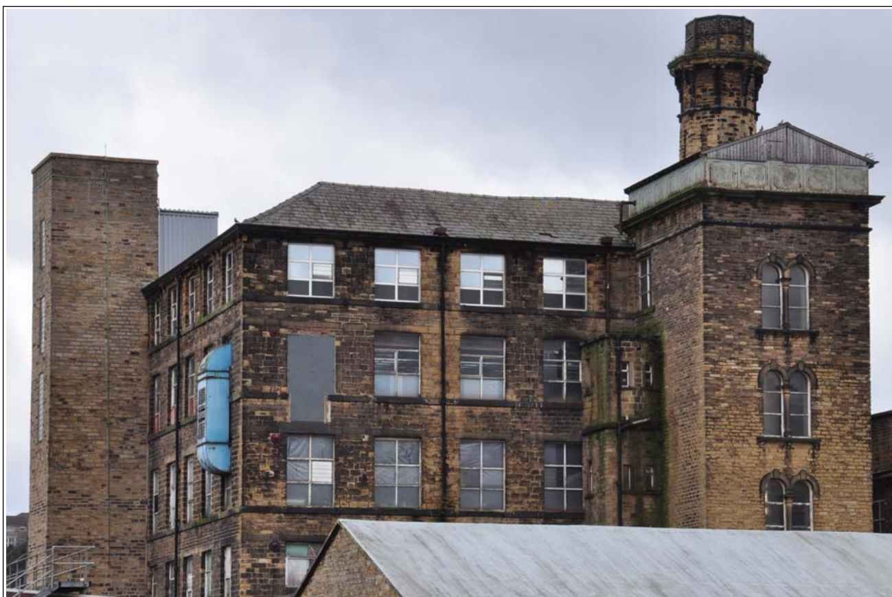
06: Building B (spinning block): upper part of west elevation and stair tower; modern lift tower at left
