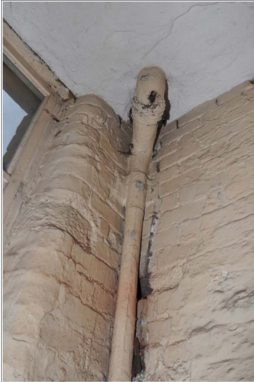
50: Building B (spinning block): stair tower on third floor: looking up towards plumbing from former WC in corner privy
