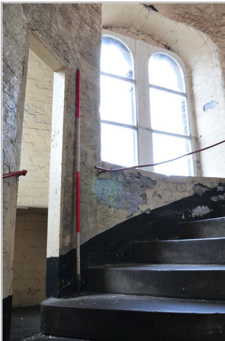
47: Building B (spinning block): stair tower on fourth floor, looking up to the west
