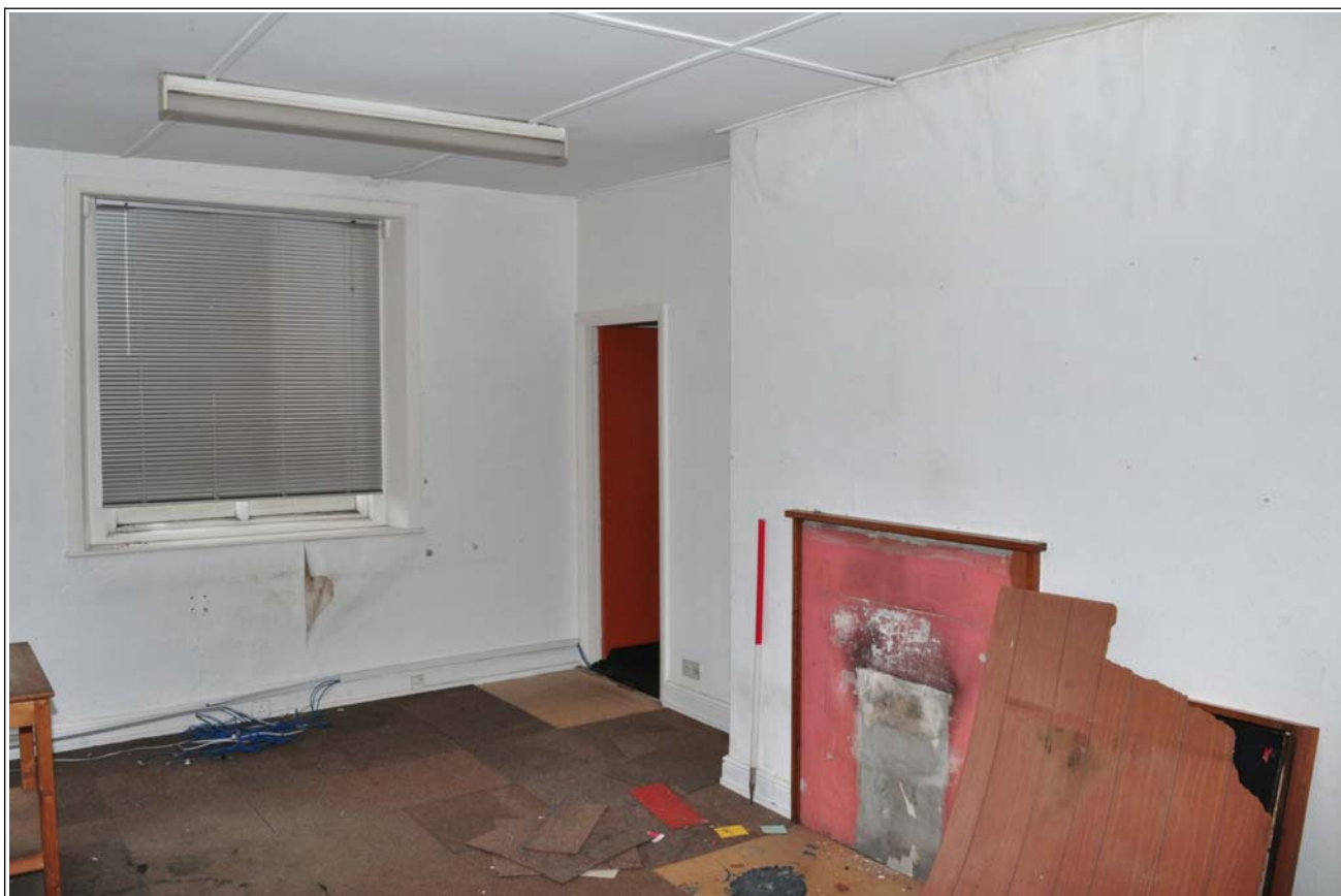
67: Building D1 (offices): interior, showing front, first floor room, with fireplace in cross-wall, looking north-west
