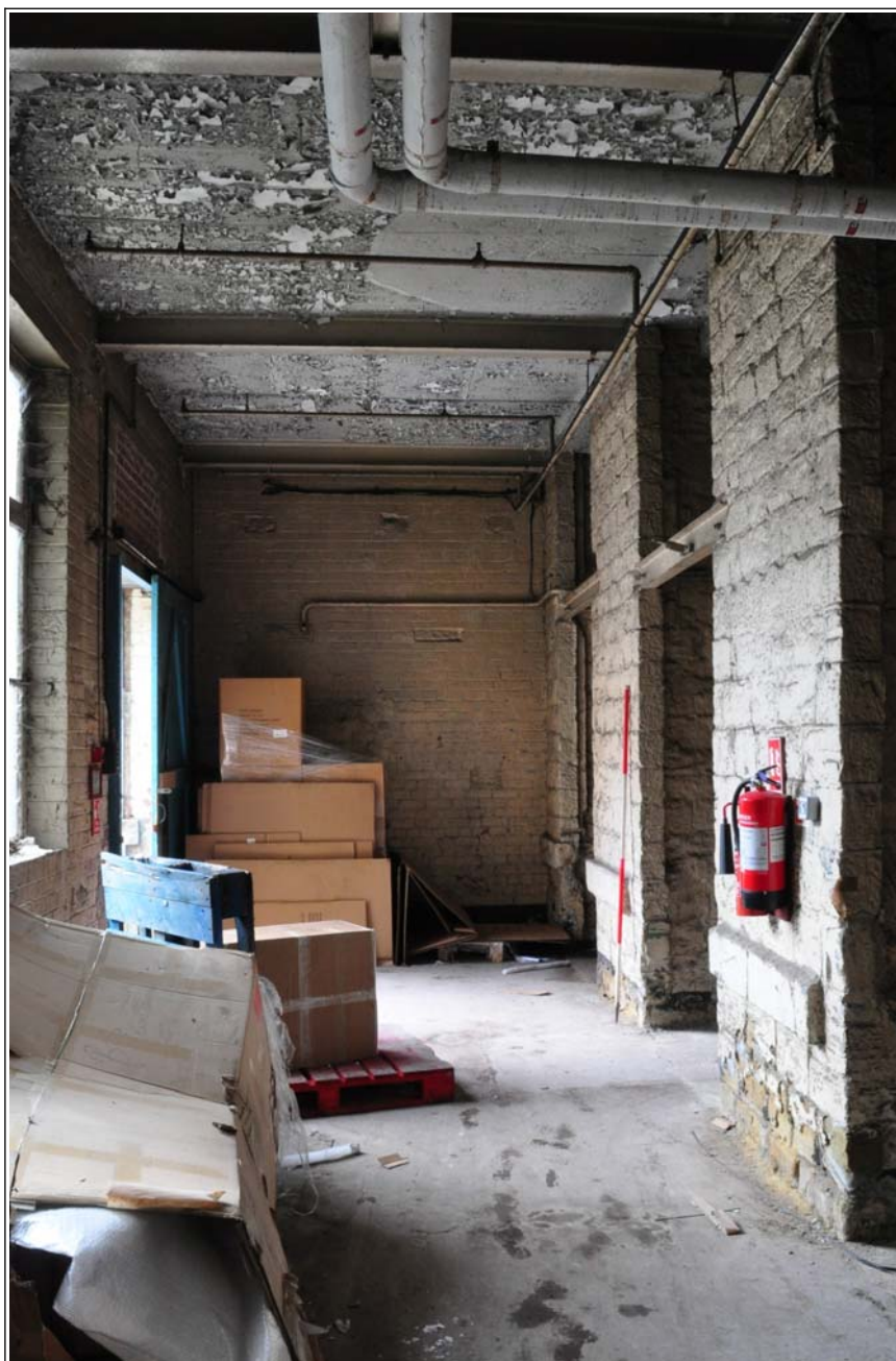
83: Building G (store), ground floor passage looking west, with original south front to right
