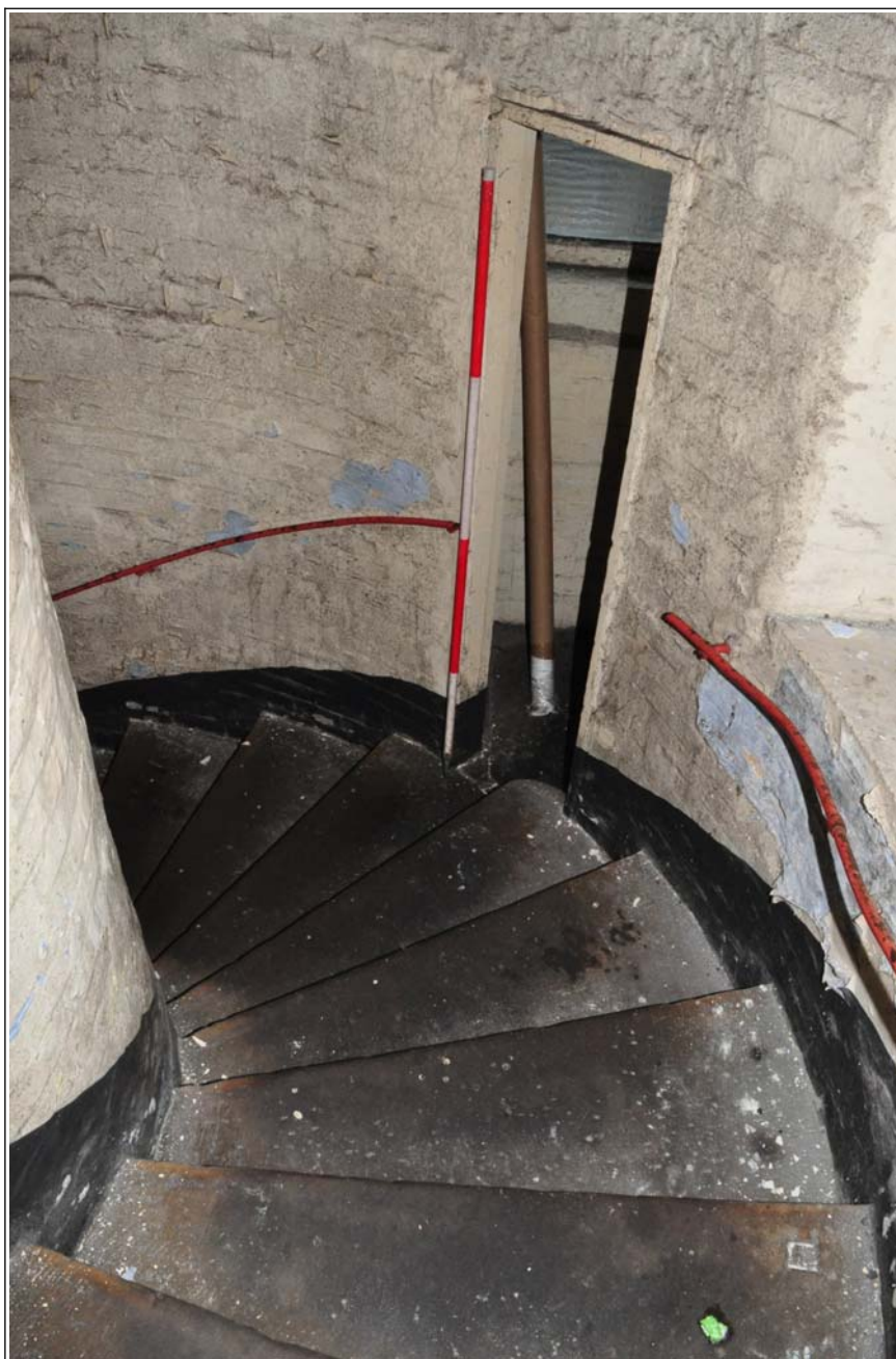
49: Building B (spinning block): stair tower on fifth floor, looking down to the south, with entrance to former privy (?)
