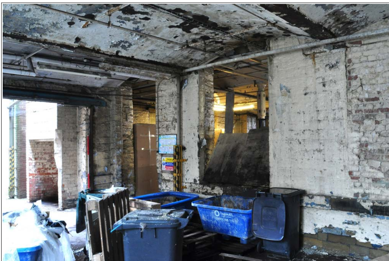
55: Building B (spinning block): extension at west side, ca. 1900, ground floor, looking north-east
