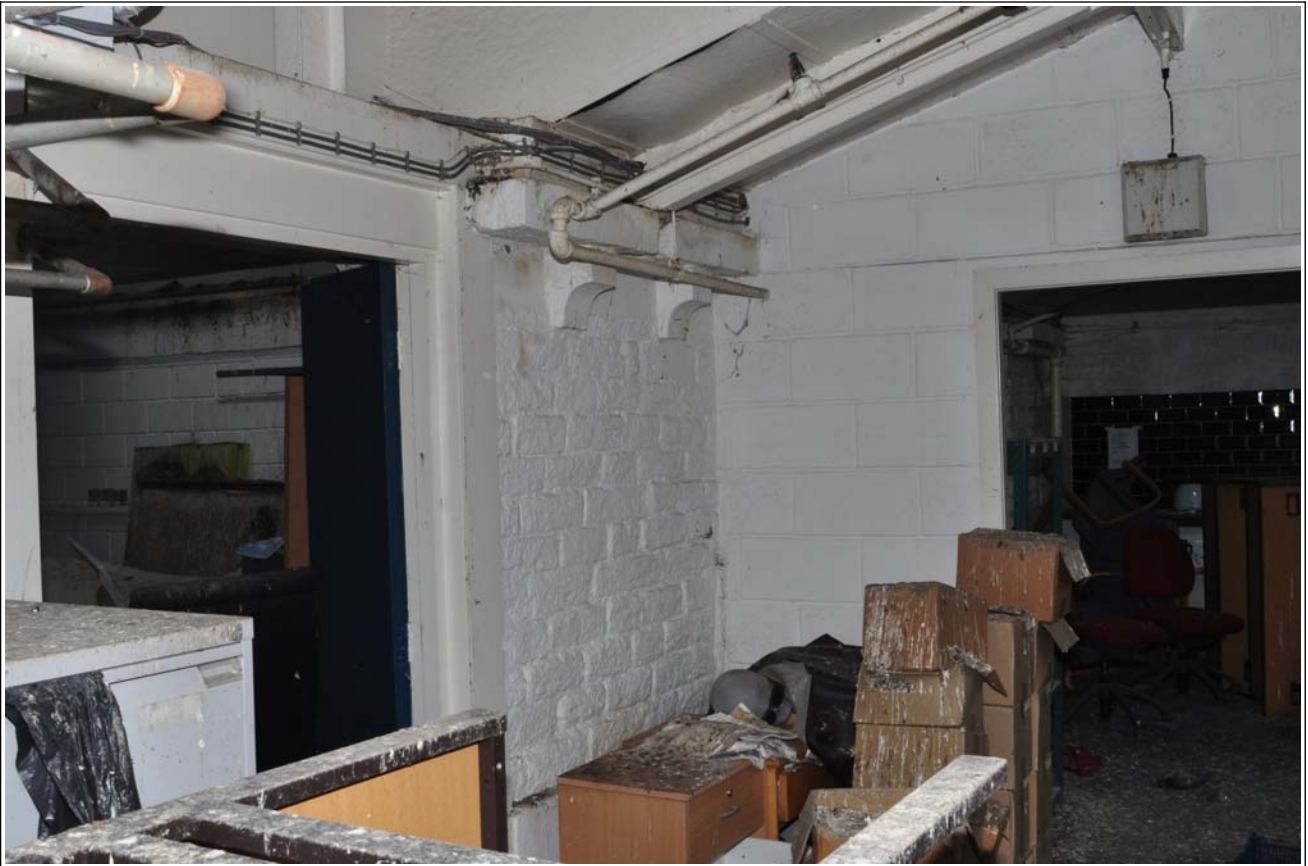
84: Building G (store), first floor, showing original eaves of south front, looking north-east
