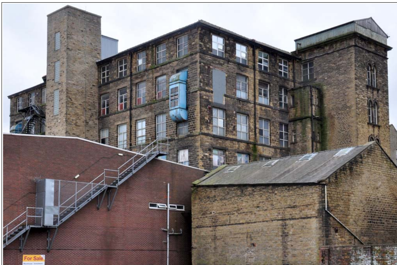
18: Building B (spinning block): general view looking south-east, showing WC tower added to north side of stair tower
