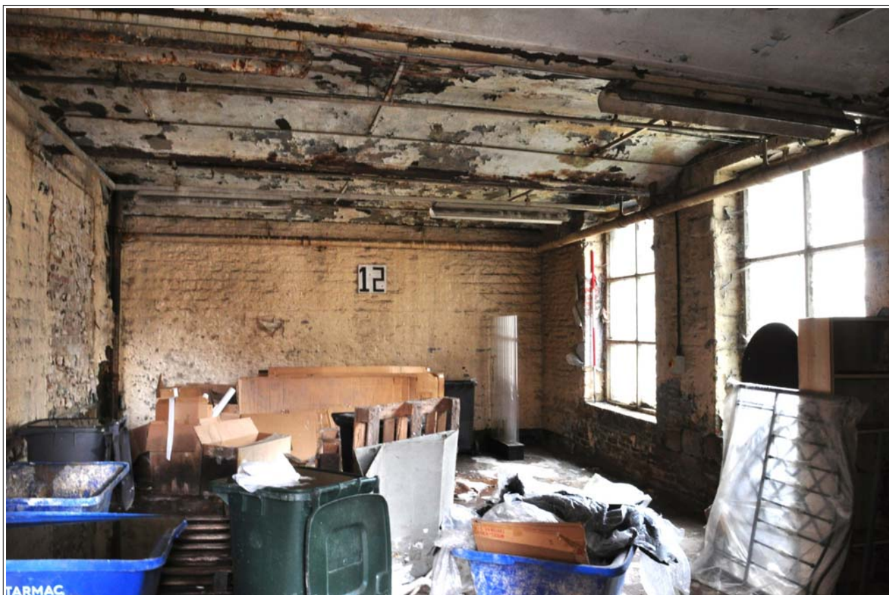
54: Building B (spinning block): extension at west side, ca. 1900, ground floor, looking south-west
