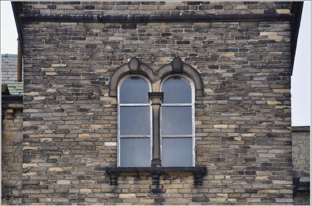
14: Building B (spinning block): top two-light window in west side of stair tower
