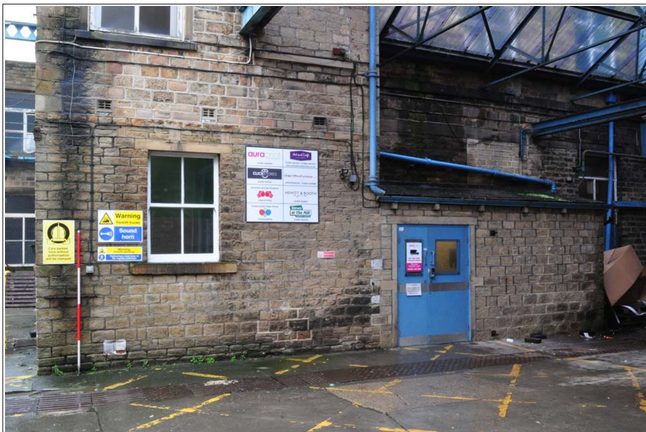
07: Building B (spinning block): south-west corner, with additions of ca. 1900 and later
