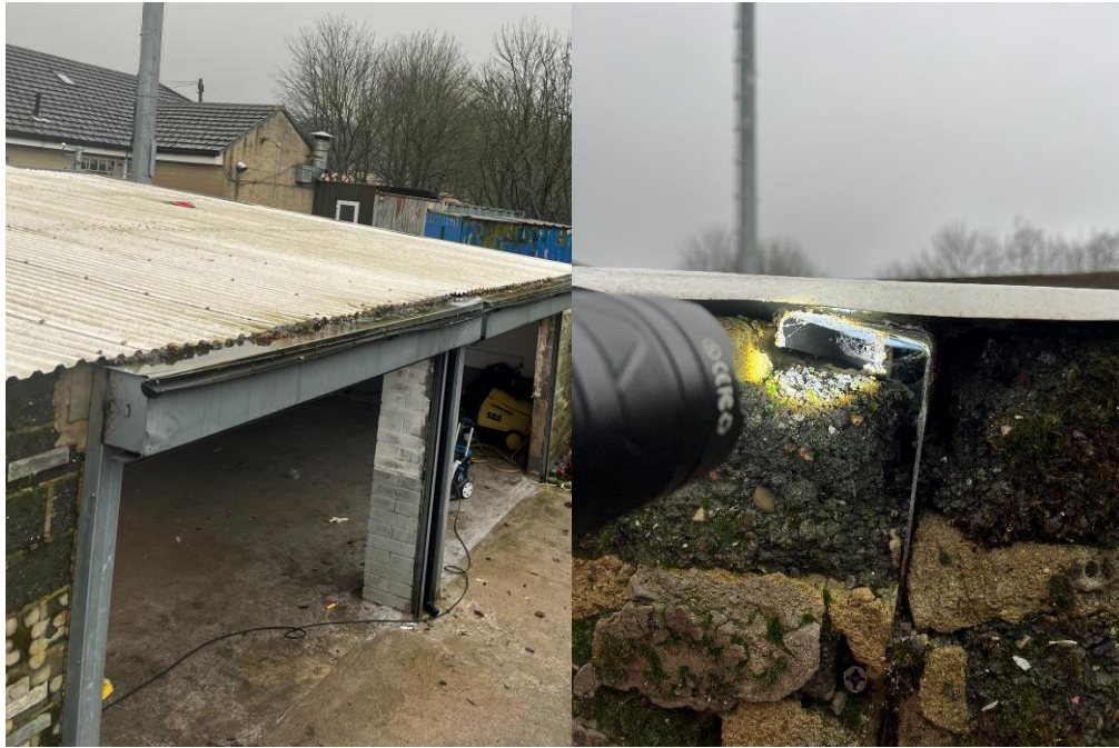
Plate 5: Infilled gaps under corrugated roofing sheets on Building C (left). Cavity to the south (right).
