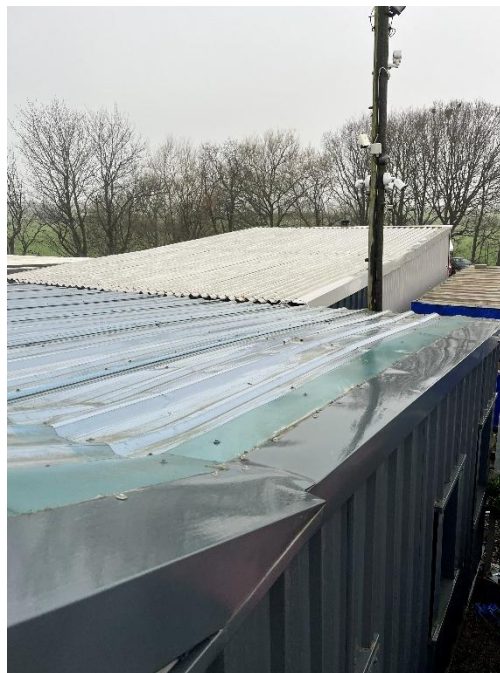
Plate 3: Gaps under the fascia where the cladding joins to the east of the Building A.
