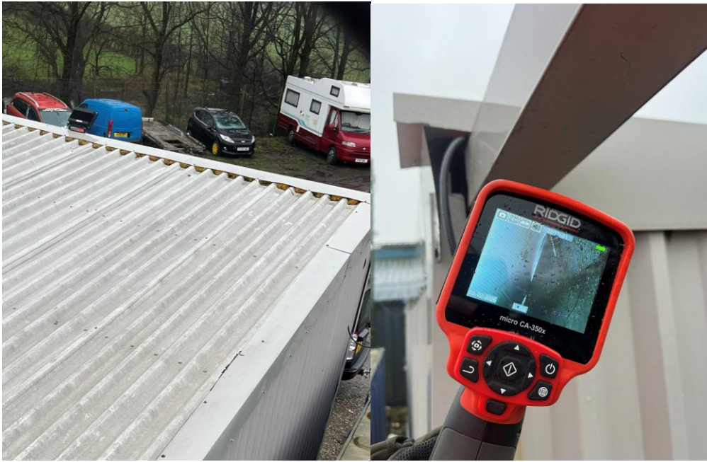
Plate 6: Infilled gaps under metal roofing on Building D (left) and the cavity between structural support and cladding (right).
