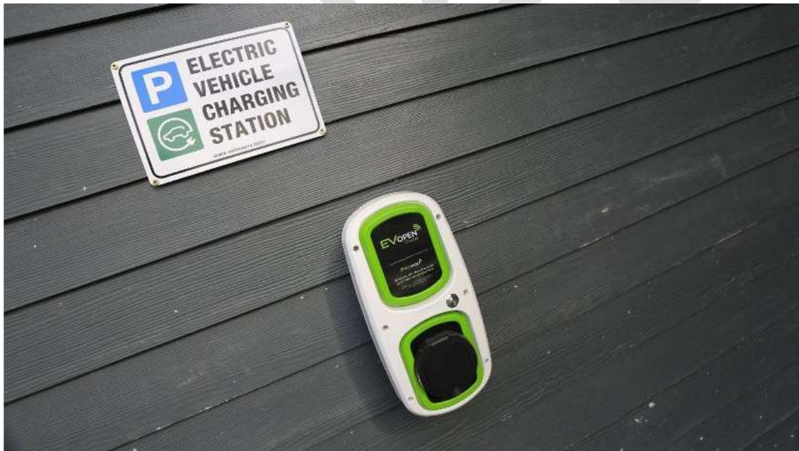
Electric Vehicle charging point
