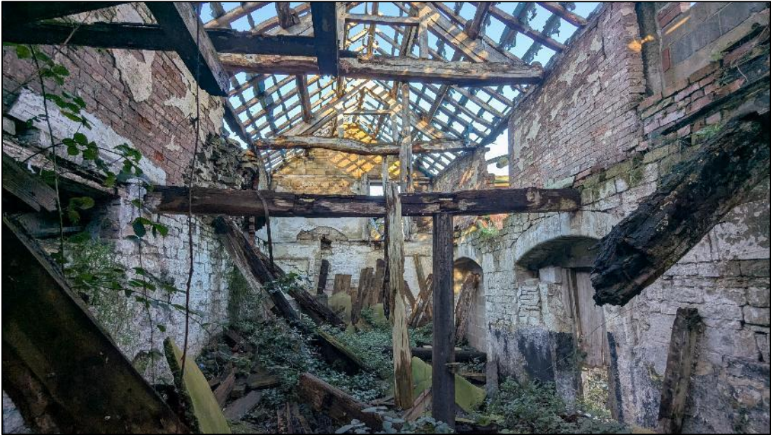
Plate 6. Example of open masonry joints on internal face of northwest gable of Building Section 1
