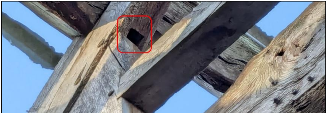
Plate 8. Open mortice joint on queen post-truss in Building Section 1
