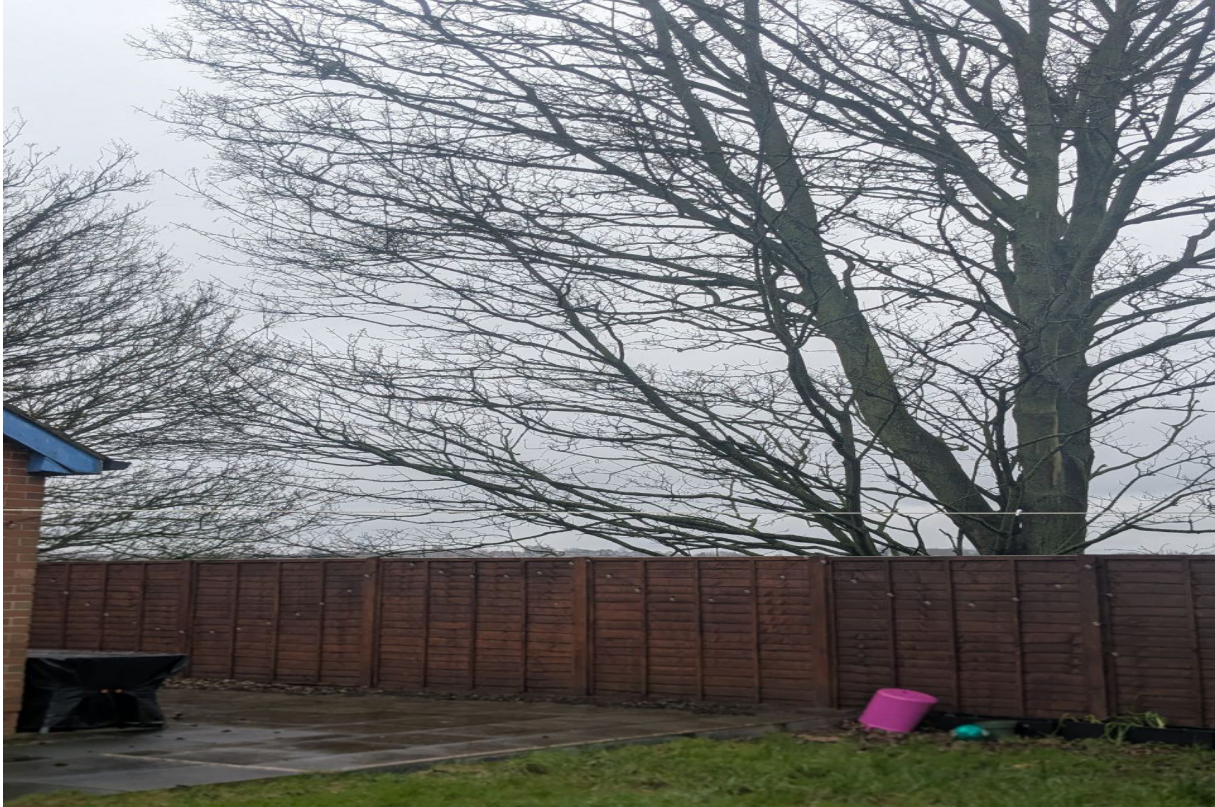
Photo 2 – Tree Height and Proximity to Roof Line: Large mature tree extending significantly above boundary fence. Upper branches extend close to roofline, raising concern during high winds.
