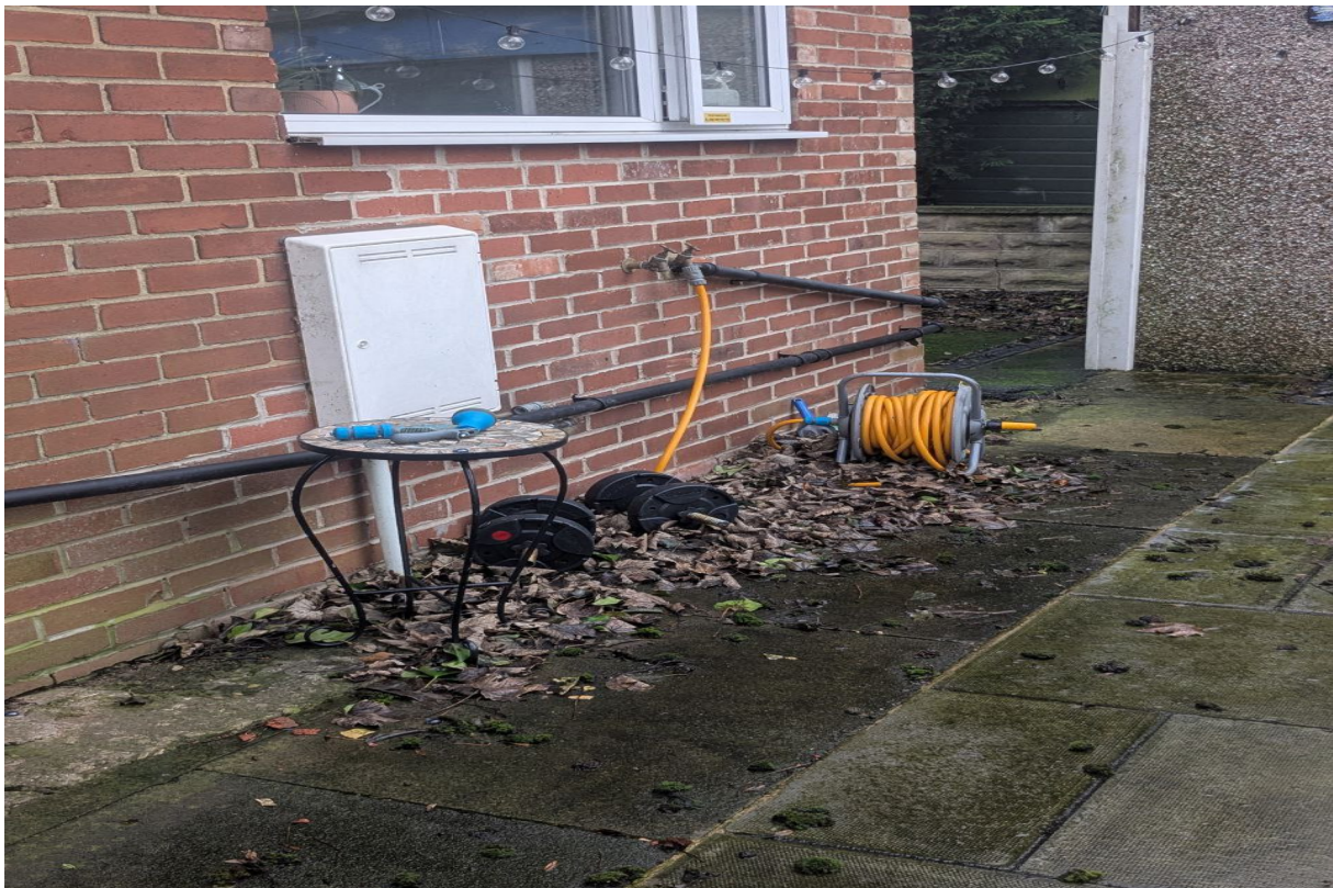
Photo 1 – Fallen Debris Along Property Wall & Kitchen Window: Accumulation of moss, twigs and leaves along patio and wall. Leaves collecting near kitchen window require frequent clearing.
