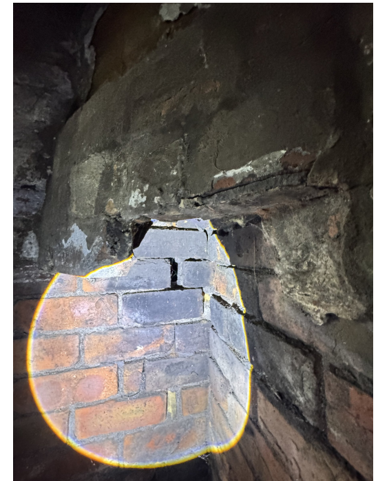
Figure 1b: Internal crevices still present in B1
