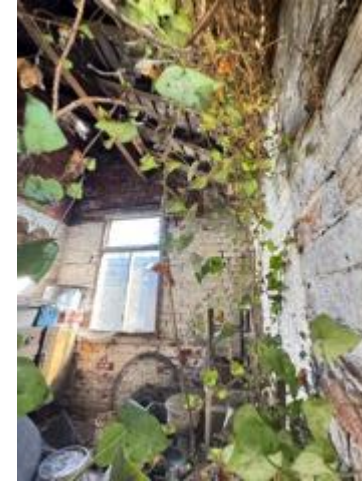
Photo 2: Light ingress and ivy preventing door to room 3 from being opened
