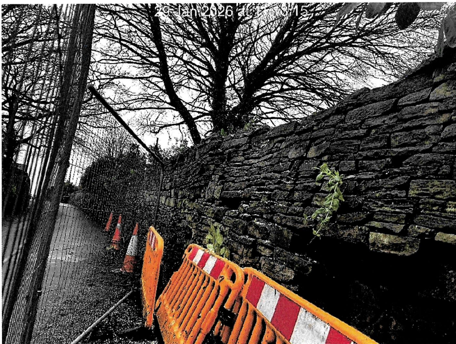
Wall has been pushed out by tree roots.
