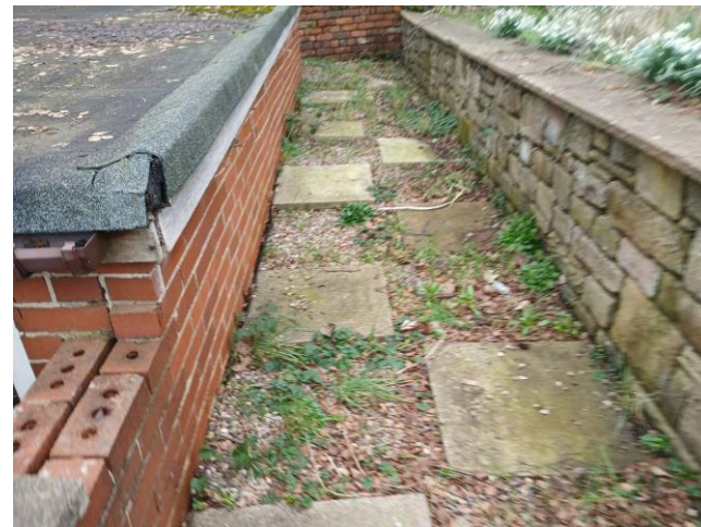
Photo 8: Gravel around the garage
