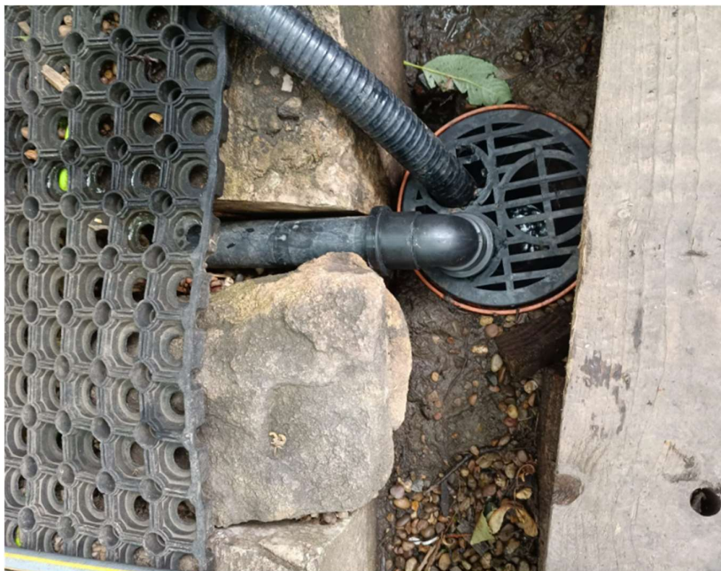
Photo 2 – Cold plunge and shower Sewer connection
