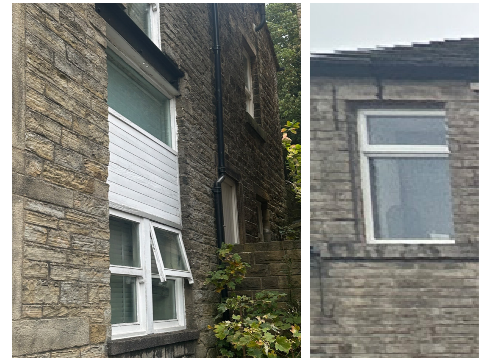
Unsympathetic modern additions.
