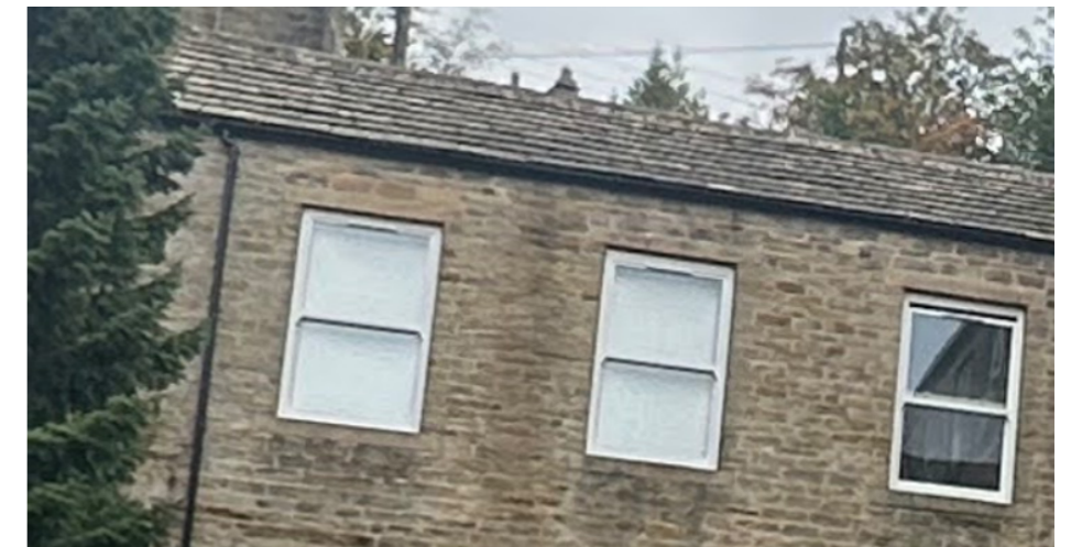
Retain high quality Timber effect UPVC sliding sash windows to West Elevation
