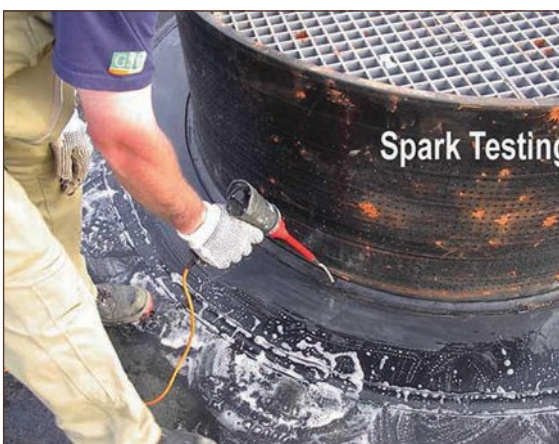
Figure A4.45 Spark testing (courtesy GSE Environmental)
