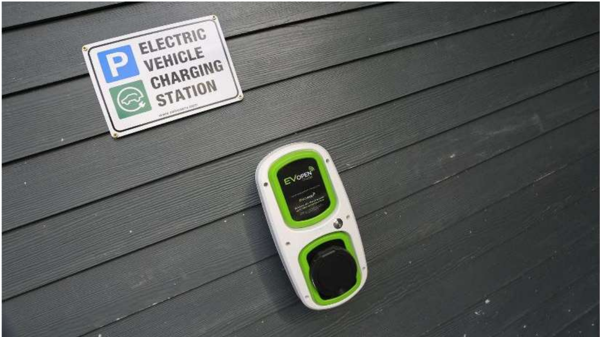
Electric Vehicle charging point
