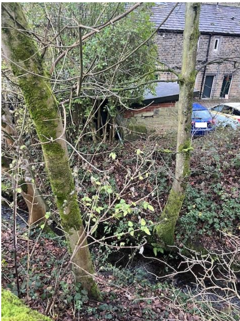
Photo 4- Sycamore growing out of side of bywash channel brick work to be removed
