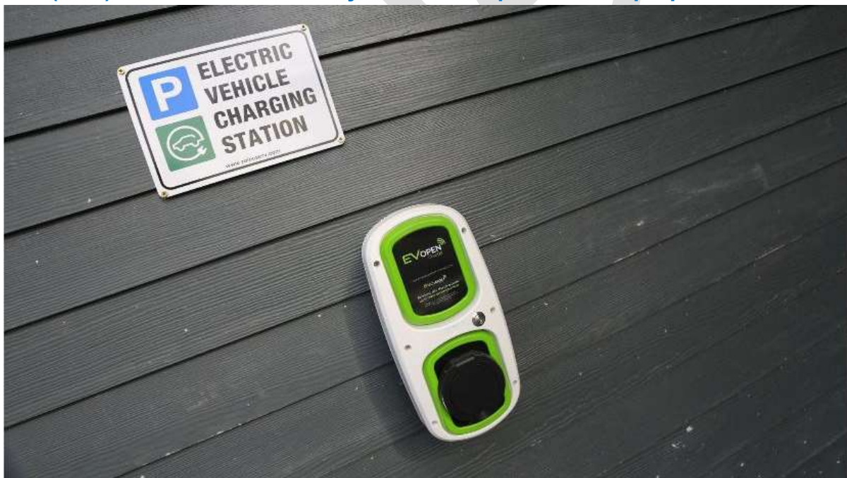
Electric Vehicle charging point
