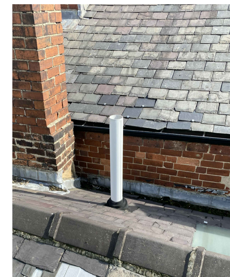
Soil Stack to Remove and Conservation Rooflight to Replace
