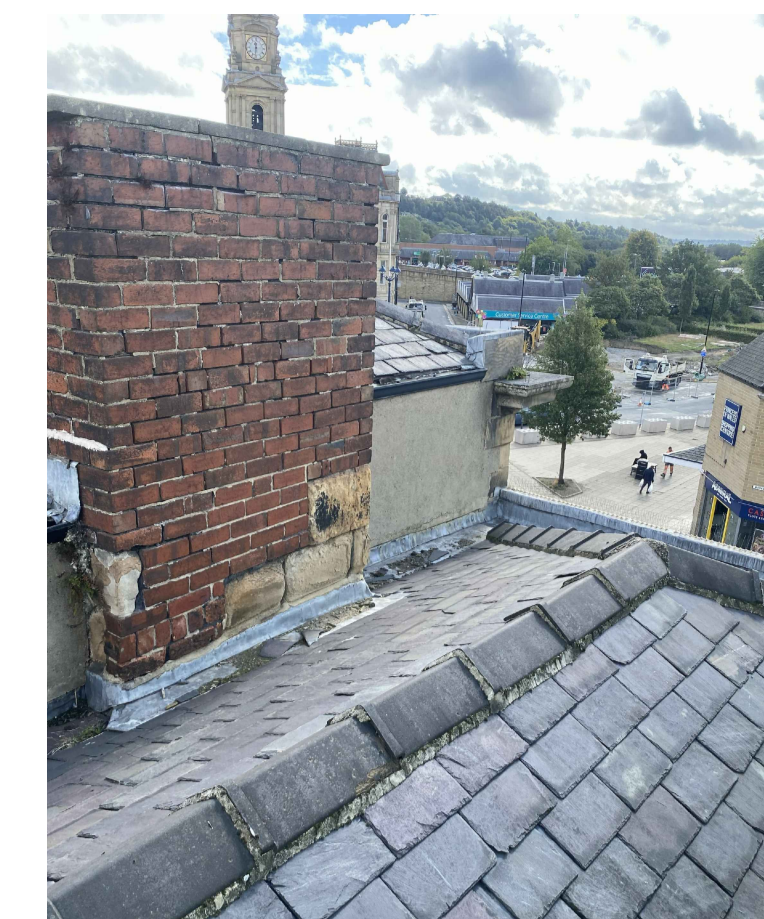
General View in Direction of Front Elevation. Note Heavily Eroded Stone Work to Neighbouring Chimney
