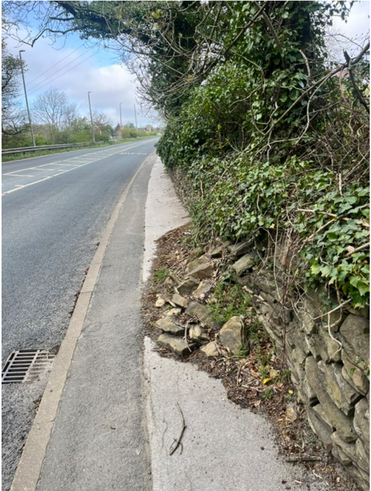
Photograph 3 – Wall collapse. The whole length of this wall is structurally unsound and poses a serious hazard to pedestrians. Footway would need to be closed and there is no footway at the other side of the road for diversion.
