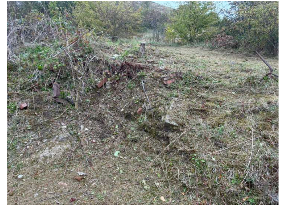
Brickwork & concrete rubble on embankment to the north of the existing building
