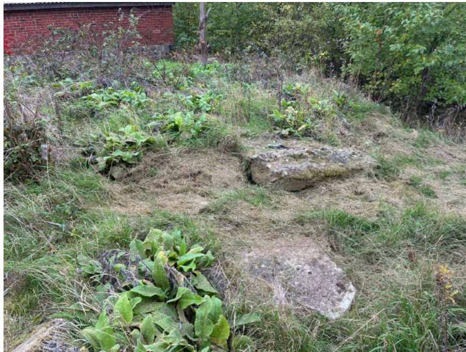
Broken up concrete slabs on plateau to the north of the existing building
