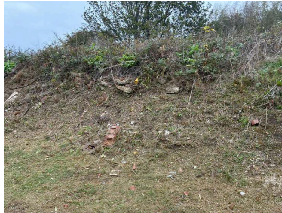
Brickwork & concrete rubble on embankment to the north of the existing building
