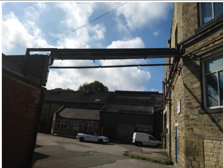
Photograph 57 – Above ground gas and electricity conduits between warehouses
