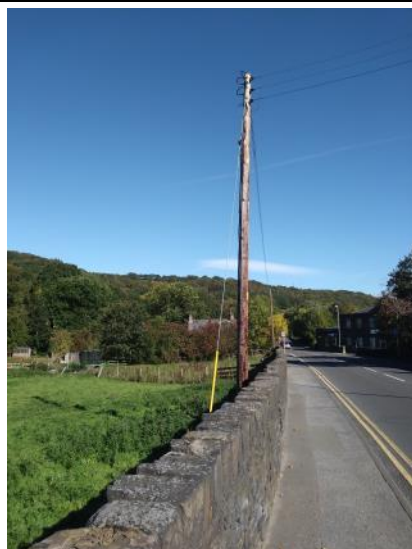
Photograph 7 – Above ground power cable entering the site
