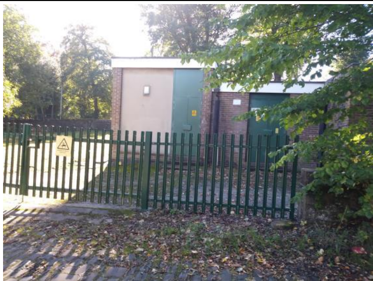
Photograph 15 – Substation located to the south of the site boundary
