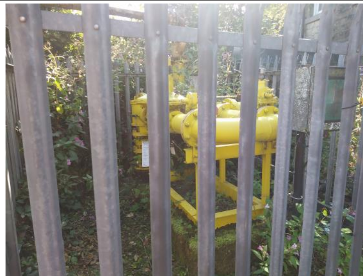
Photograph 62 – Gas governor to north of Northern Dyers building
