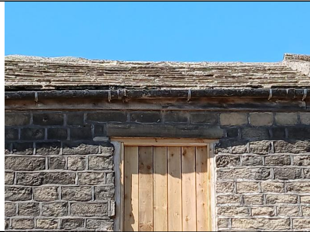
Photo 31: Lifted tiles on the eastern facing roof of building 4.
