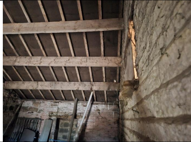
Photo 23: Wooden boarding under tiling in building 4.
