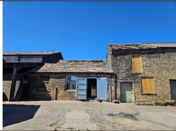
Photo 19: Eastern facing view of building 4. Lifted tiles and wooden panelling.
