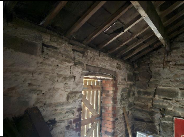
Photo 25: Holes in the wooden boarding of building 4.
