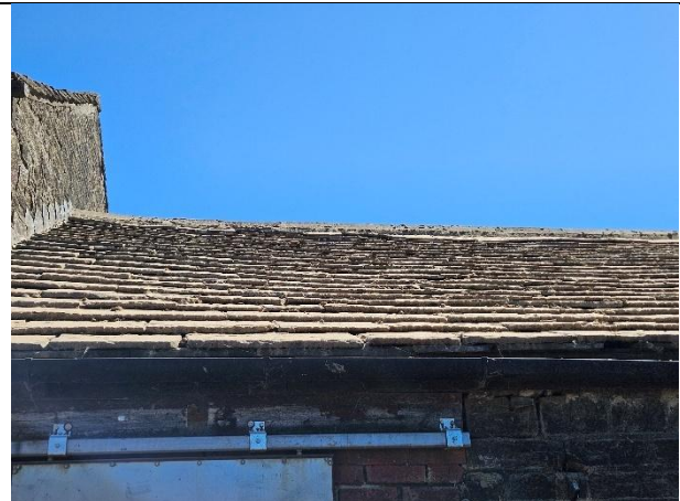
Photo 18: Lifted tiles on building 4.
