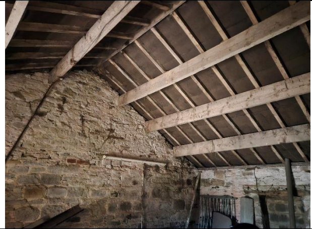
Photo 24: Wooden boarding under tiling in building 4.
