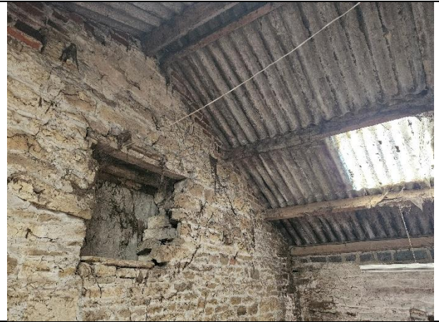
Photo 26: Holes in the inside walls of building 4.
