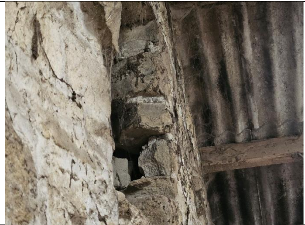
Photo 22: Hole in the wall inside building 4.
