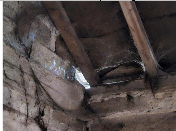
Photo 21: Hole in the wall inside building 4.
