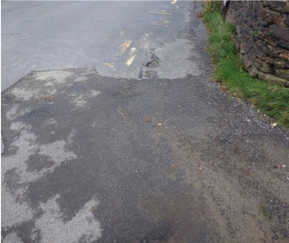
Figure 71 Dobb Lane location BO
