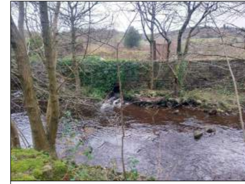
Photo 6 View of River Colne to the south, and evidence of a culvert.
