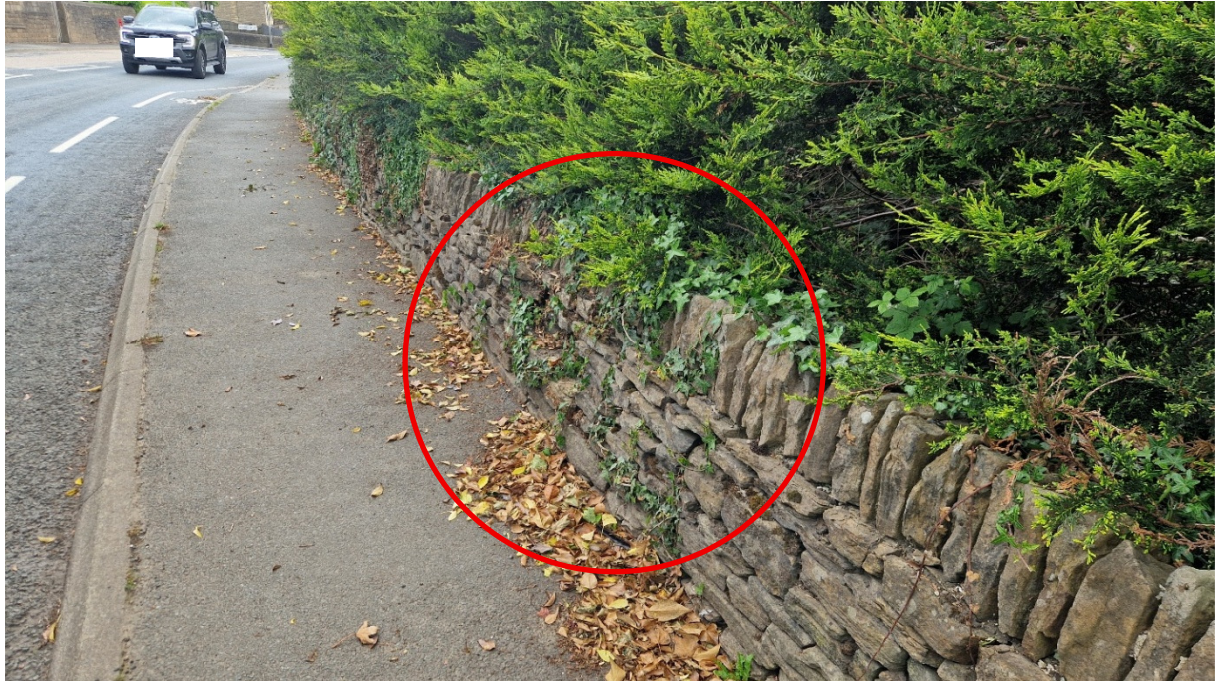
Figure 4. Minor impact damage
