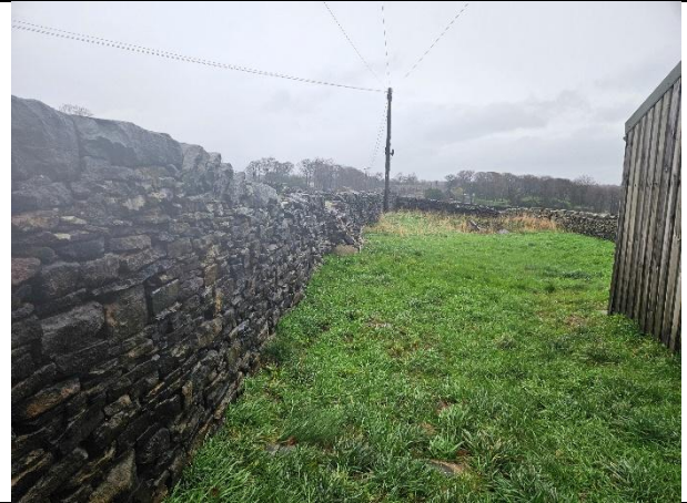
Photo 8: The back of B1 and G2 and location of collapsed drystone wall.
