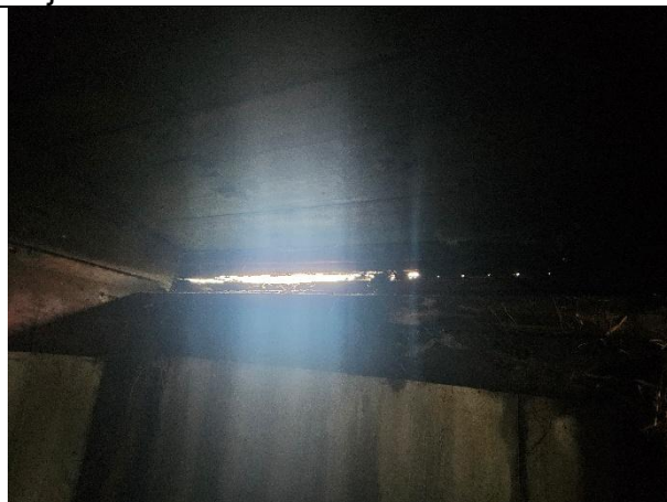
Photo 4: Gap in roof noted in B2.
