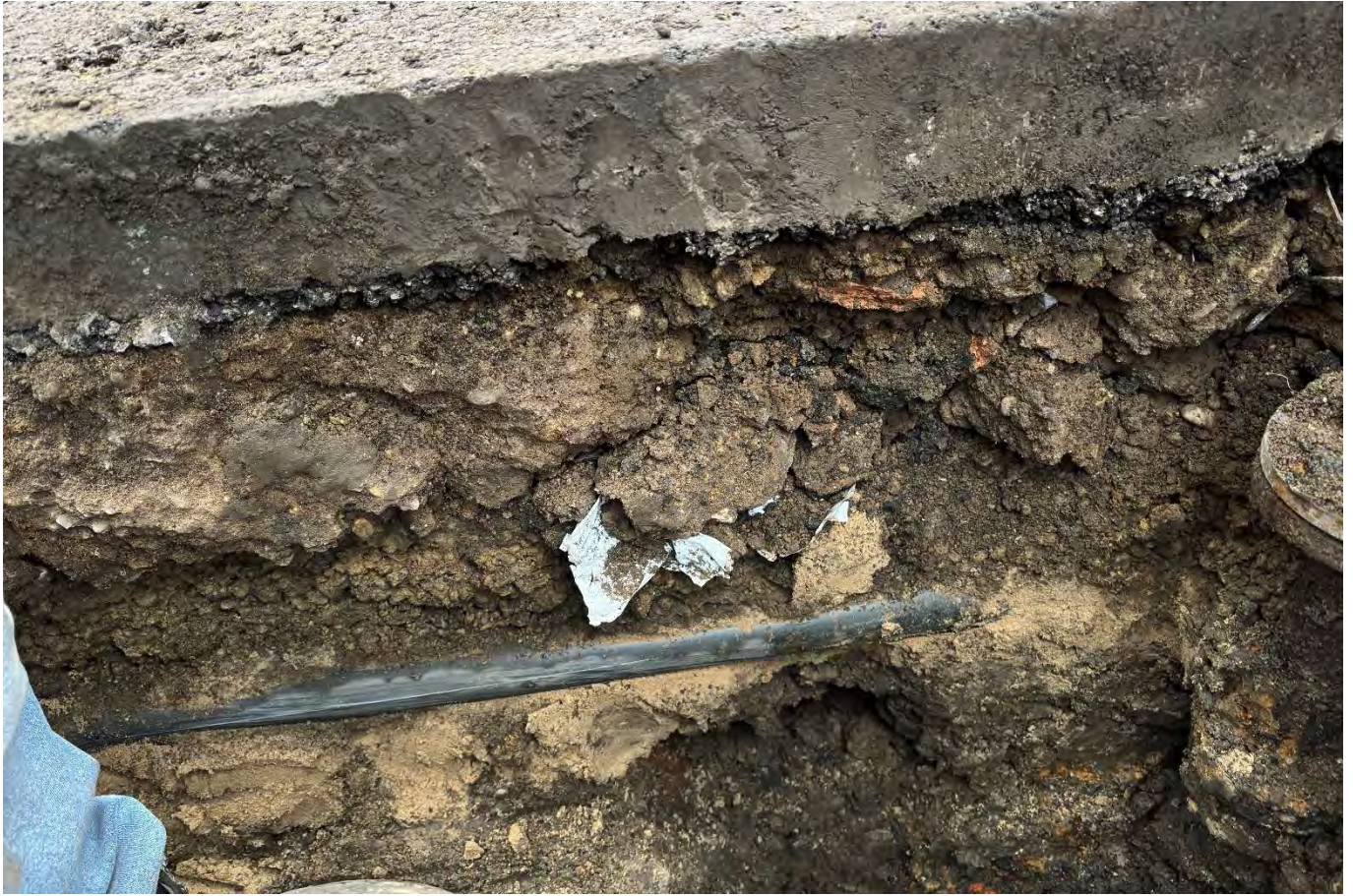
TP15: Showing unspecified service extending along trench alignment
