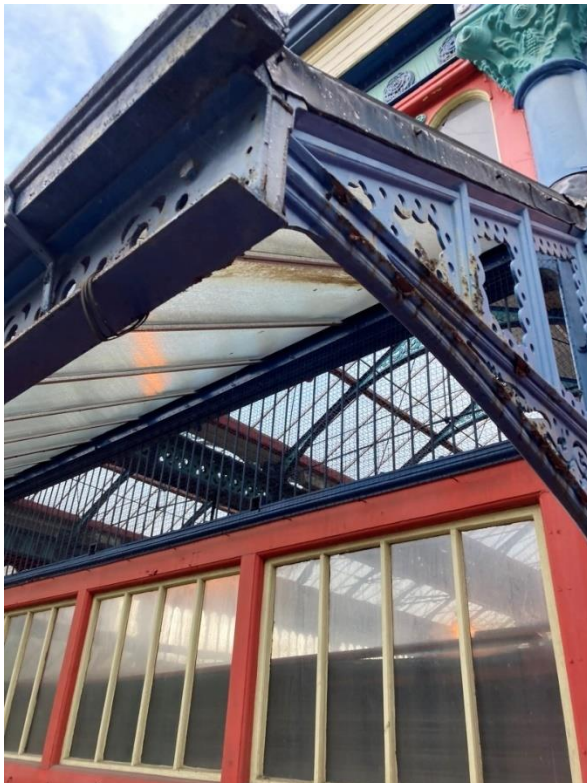
20. Corrosion of canopy spandrels – typical throughout
