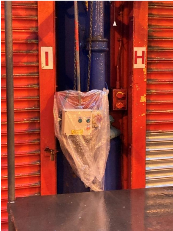
32. Blocked downpipe (D5) has resulted in water cascading onto electrics (roller shutter mechanism)
