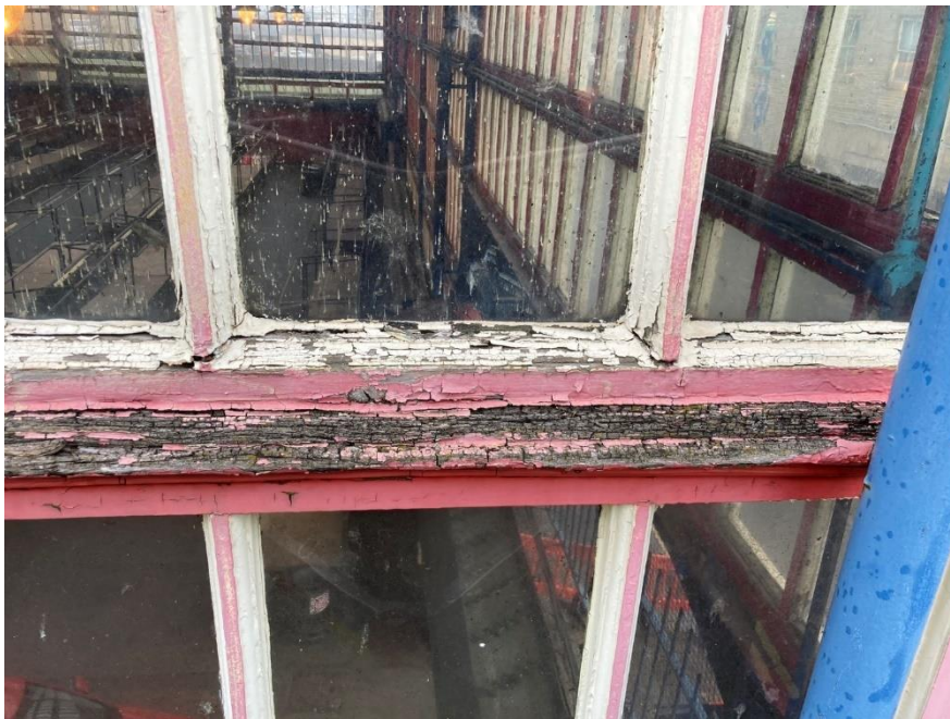
10. Bay 6 of the Back Street elevation of the main market – window frame has significant rot to bottom bar
