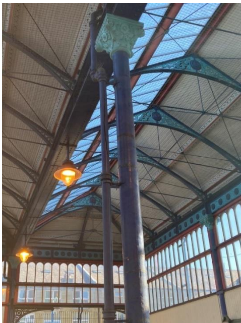
29. Downpipe (D9) cracked and general view of netting
