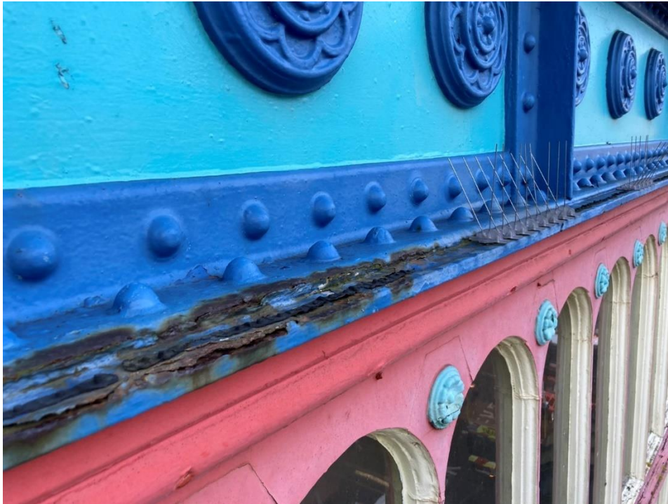
19. Delamination of flange to exposed east corner
