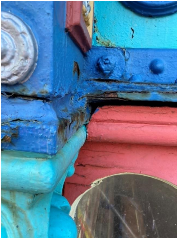
18. Slight loss of section on flange of beam-to-column connection
