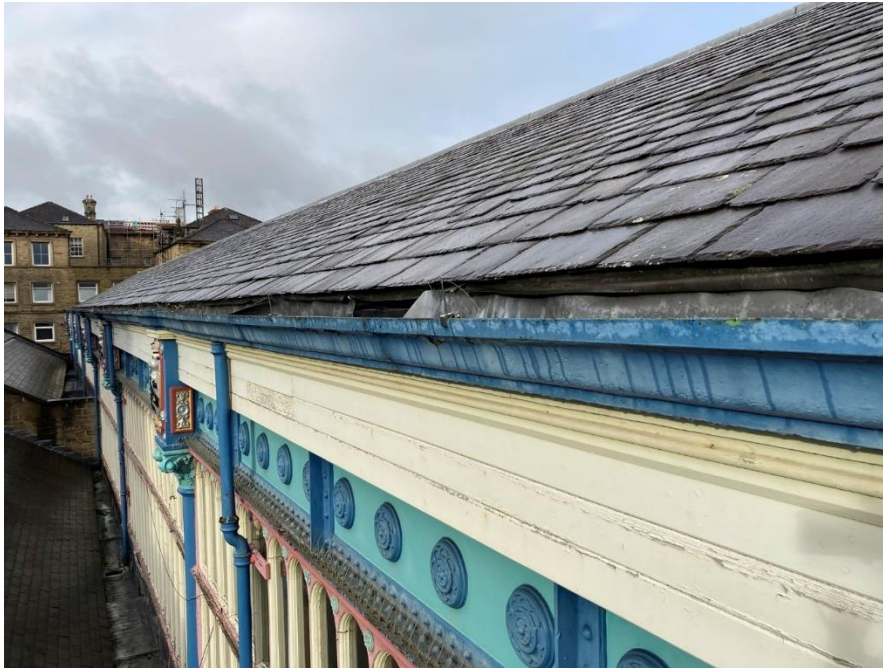
11. Back Street elevation of the main market – missing leadwork and typical condition of fascia board with decorative finish failing but minimal amounts of rot
