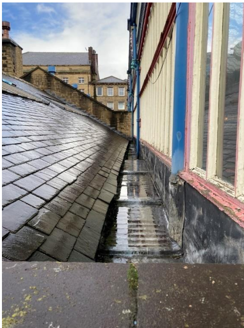
8. Box gutter between main market building and stone extension
