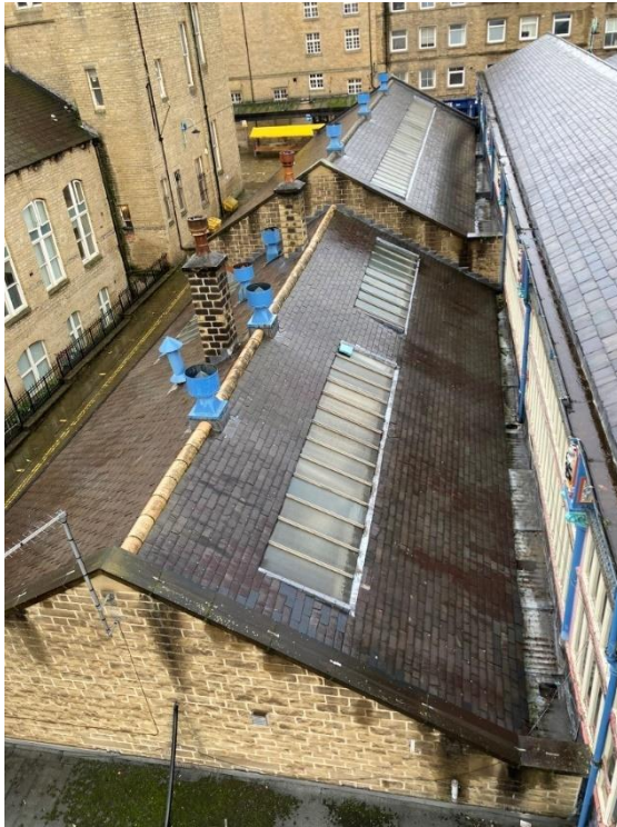
7. General view of stone extension roofs (ER1 and ER2) – note the redundant vents and saturation of stonework due to failure of parapet coping jointing
