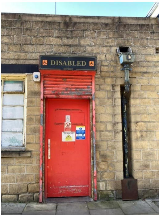
27. Lord Street elevation of stone extension – note cracking to lintel behind roller shutter housing and typical condition of cast iron downpipe
