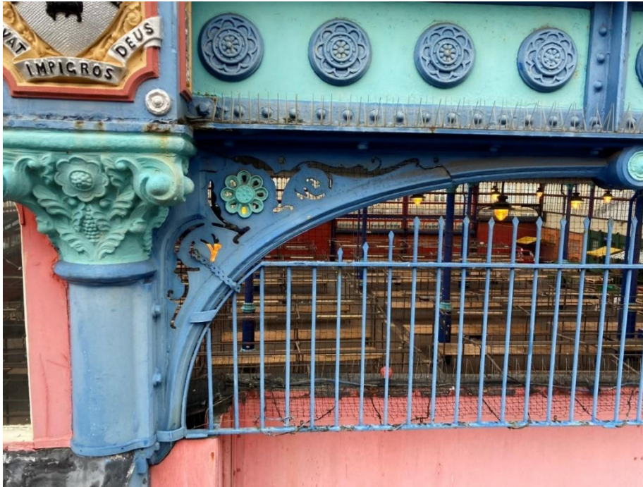
21. Crack to spandrel on Byram Street
