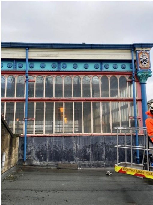
9. Bay 6 of the Back Street elevation of the main market – window frame has significant rot to bottom bar and glazing has dropped
