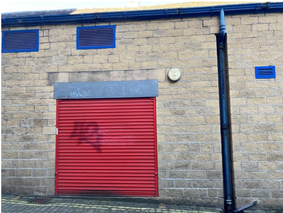
25. Back Street elevation of stone extension – corroded downpipe and cracking to masonry
