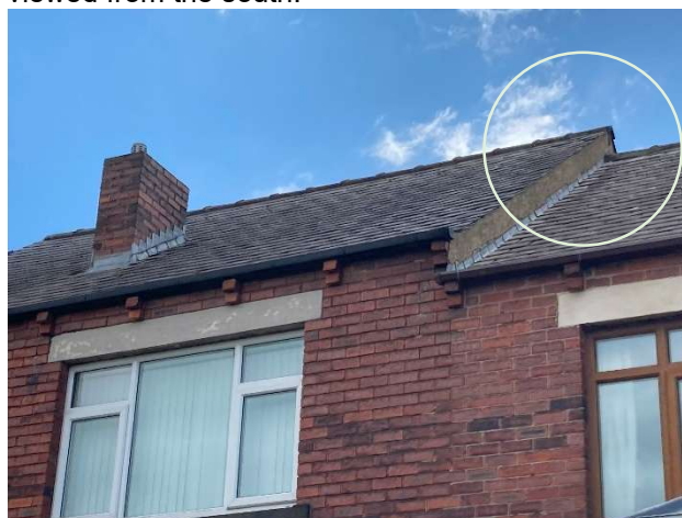
Photo 24: Lifted tile and gap in ridge tile on the northern aspects of Building 1 & 2.
