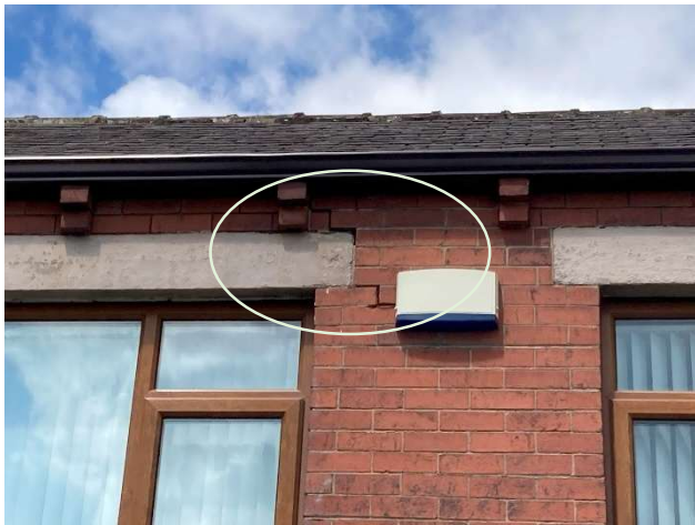
Photo 27: Missing mortar on the southern aspect of Building 2.
