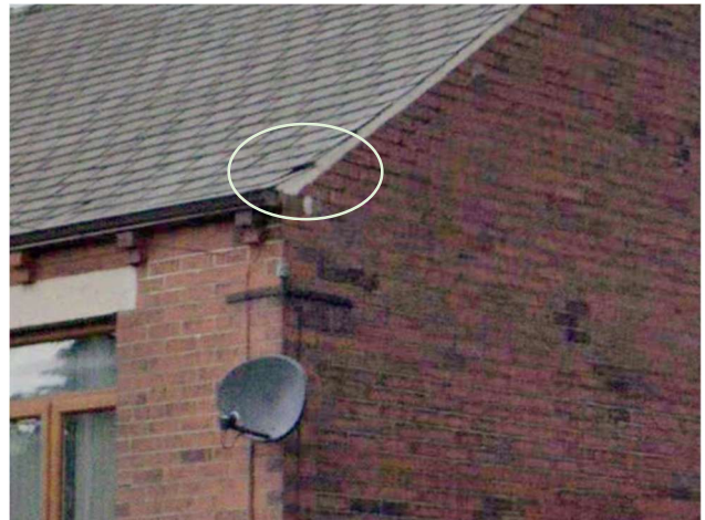
Photo 26: Lifted Tile on the southeastern corner of Building 2.
