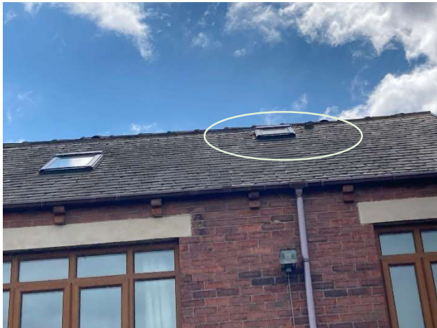
Photo 25: Lifted tile on the northern aspects of Building 1.
