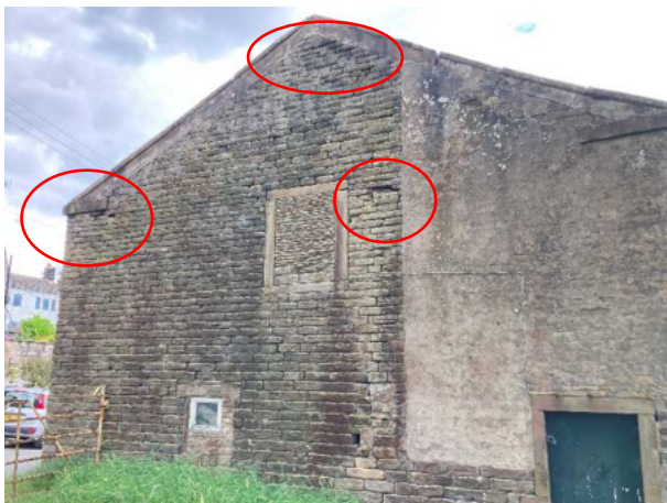
Photo 11: Missing mortar and air vents on the western aspect of Building 1.
