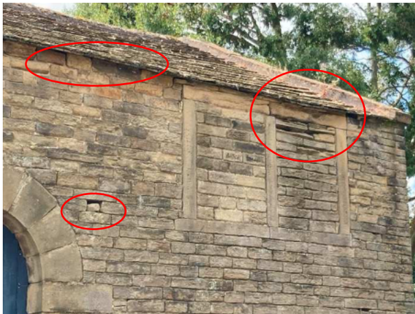
Photo 7: Missing mortar, gaps in the eaves and lifted tiles on the northern aspect of Building 1.
