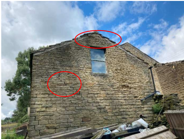
Photo 9: Missing mortar on the extension on the eastern aspect of Building 1.
