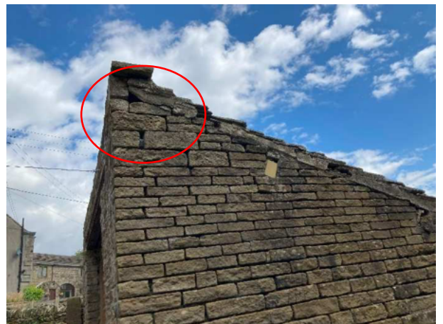
Photo 12: Missing mortar on the southern aspect of Building 2.
