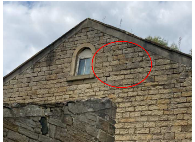
Photo 8: Missing mortar on the eastern aspect of Building 1.
