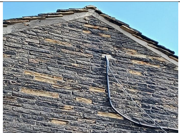
Photo 10: Lifted tiles on building 1.
