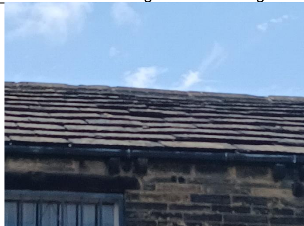
Photo 11: Lifted tiles on building 1.
