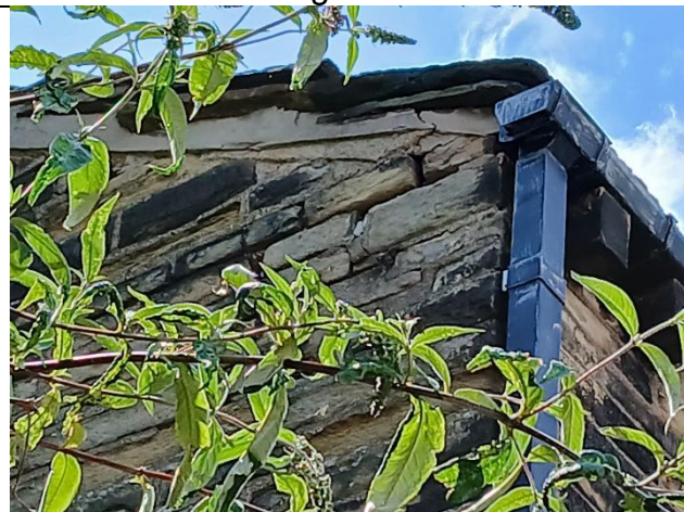
Photo 21: Gaps in the mortar of building 1.
