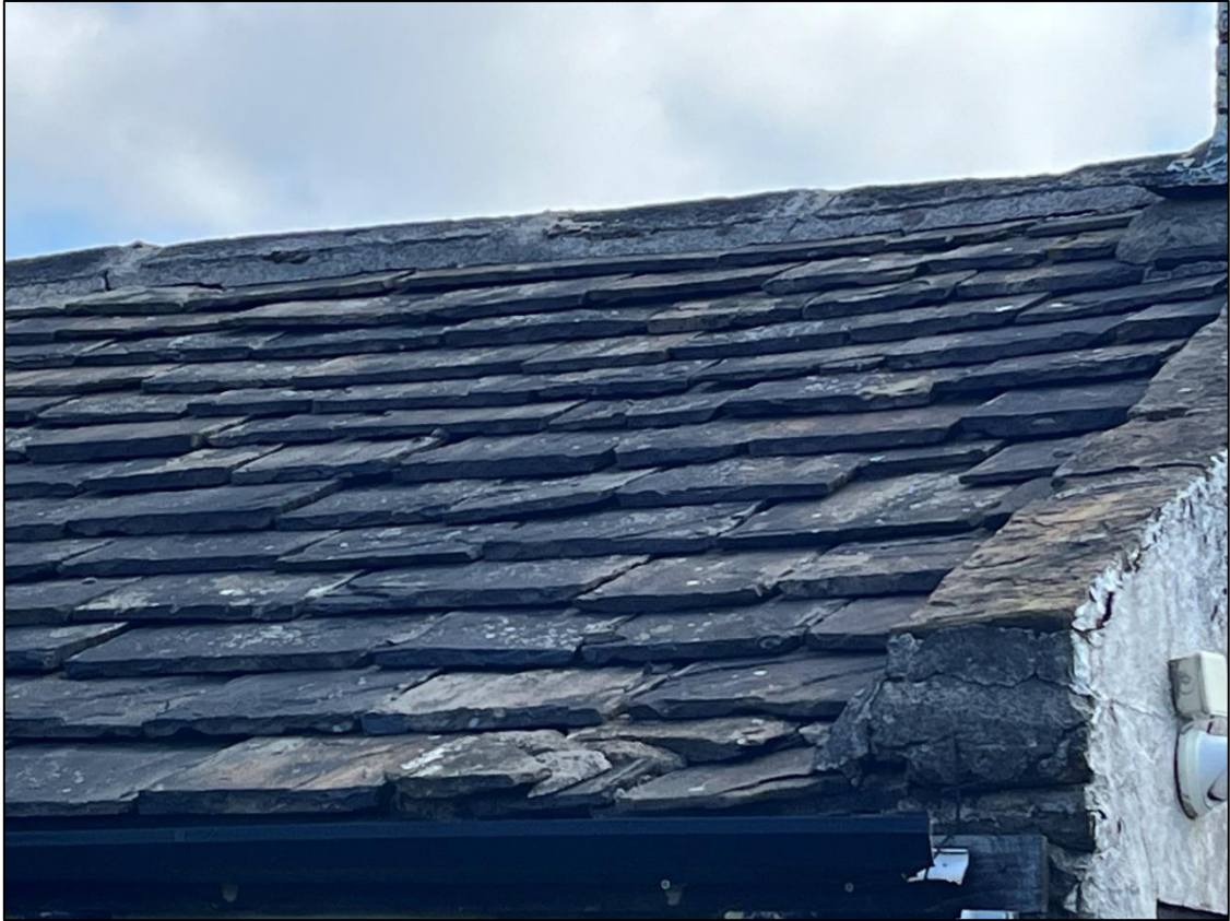
Plate 9 – Uneven nature of roof tiles
