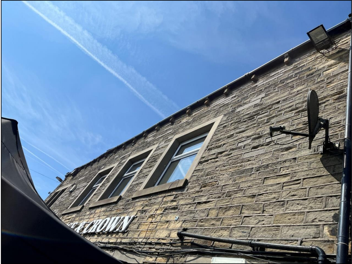
Plate 11 – Gaps at open eaves
