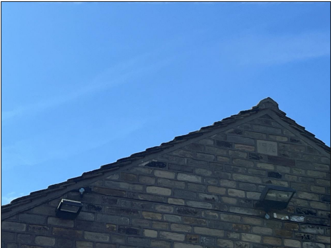
Plate 8 – Gaps along gable verges
