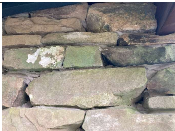
Photo 8: PRF missing mortar in building
