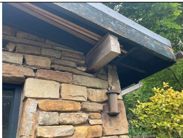
Photo 6: PRF gap between wall and roof on building
