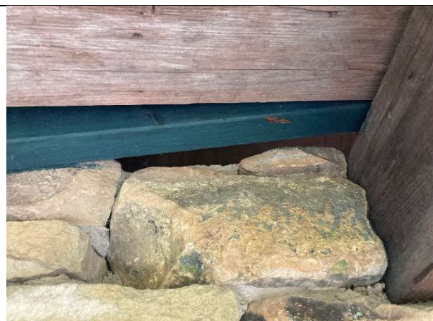
Photo 7: PRF gap between wall and roof on building
