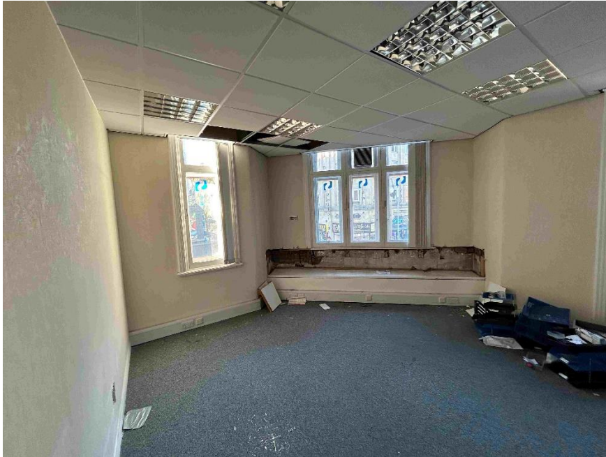
PHOTOGRAPH 1 – Modern fixtures to be removed. Vertical Boarding added under window. Window Surrounds to Remain. Skirtings to be replaced.
