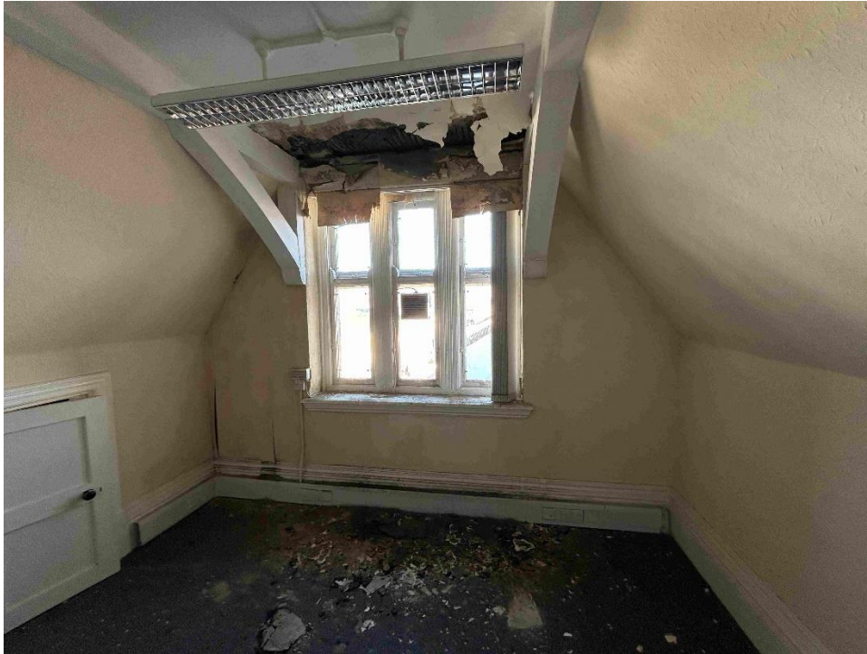
PHOTOGRAPH 16 – Modern fixtures To be removed. Window Surrounds to Remain. Skirtings to be restored / replaced. Roof to be repaired.
