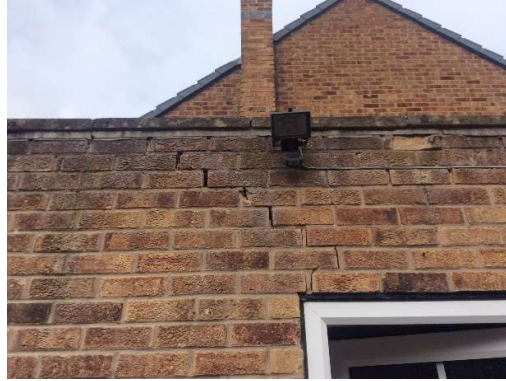
External cracking to LHS of property
