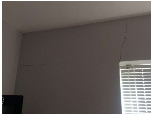
Internal cracking to rear left bedroom
