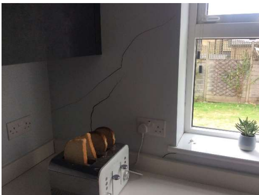
Cracking to rear left corner of kitchen
