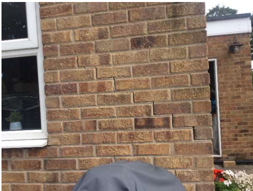
External cracking to rear elevation
