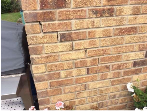
External cracking at rear left corner
