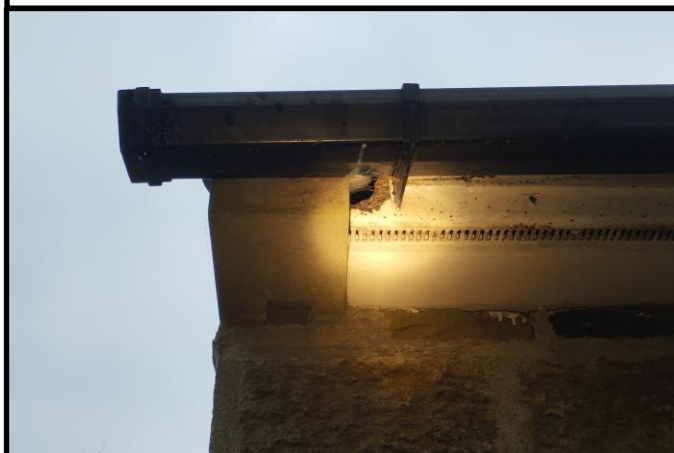
Photograph 3. Example of damage to soffit box allowing access to the voids of the property
