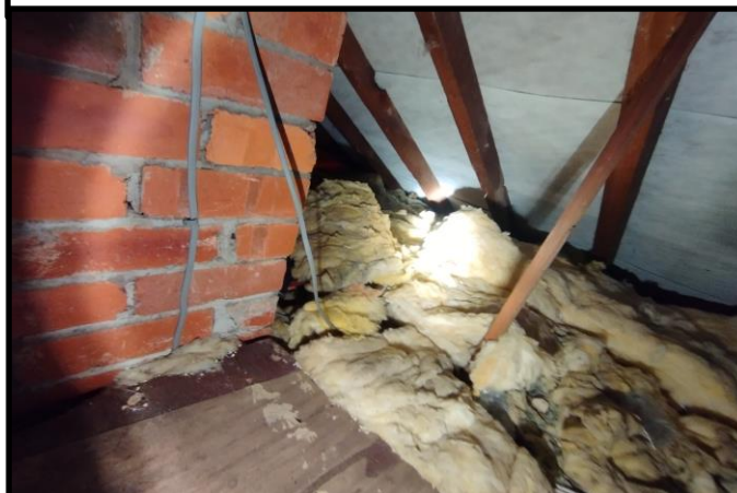
Photograph 5. Example of small sections of roof voids not converted
