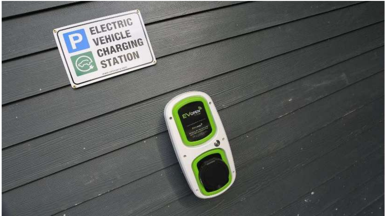
Electric Vehicle charging point
