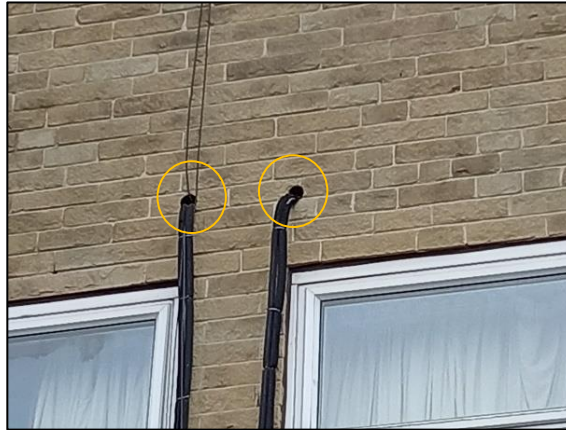
Figure 8 Gaps surrounding electric cable entry points to the north aspect.
