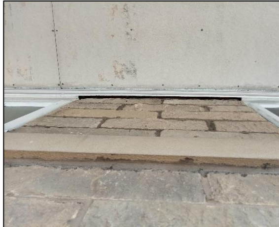
Figure 10 Missing joinery flashing between the brick wall and ceiling, south aspect terrace.
