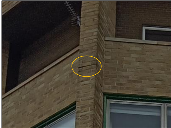
Figure 7 Gaps in mortar on structural columns to the east aspect (hexagonal building).
